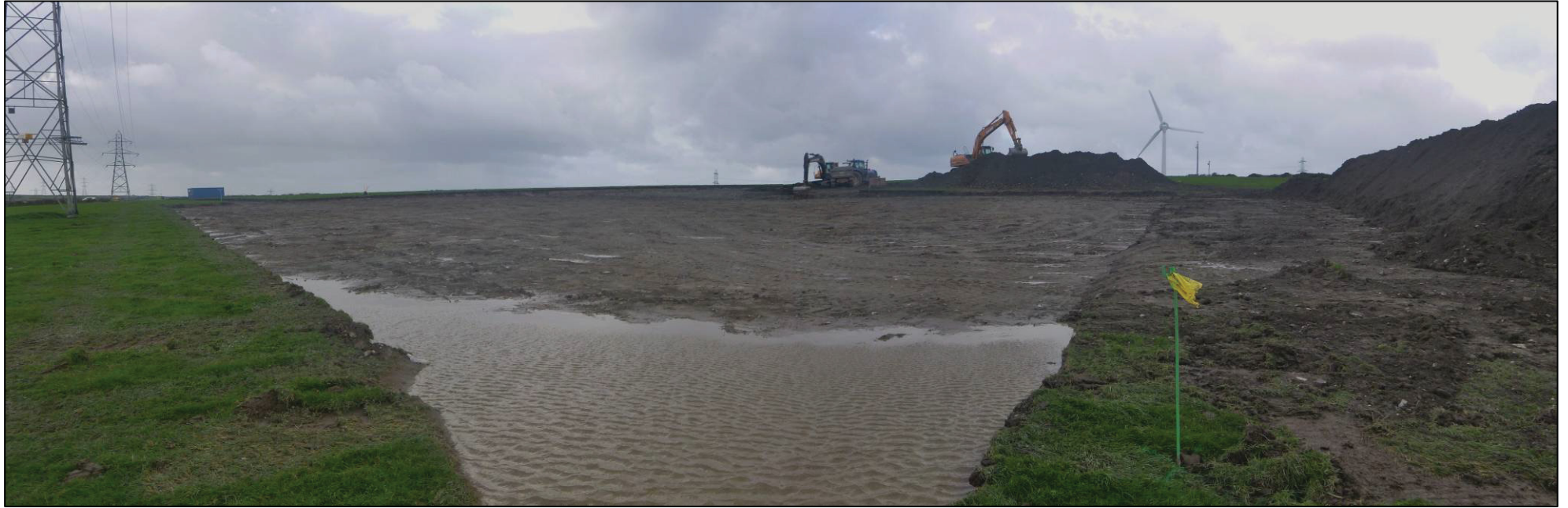
Figure 9: Site after removal of secondary (102) material at northern side (view from NE corner looking NW across site).
