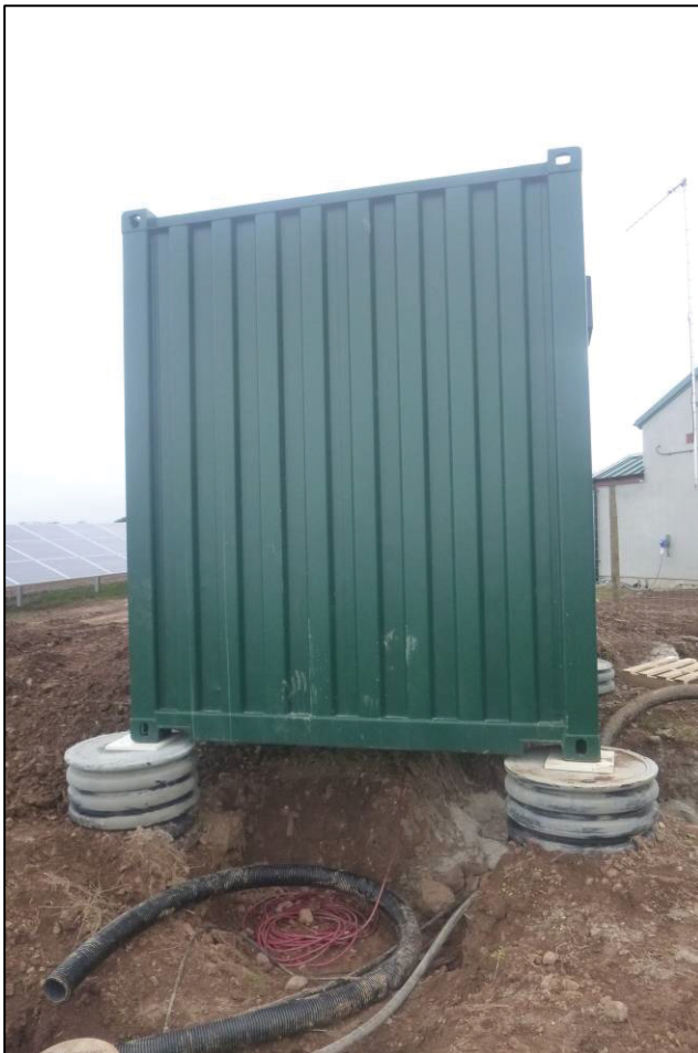
Figure 11: Field B inverter house in situ with cable trench (looking SE)
