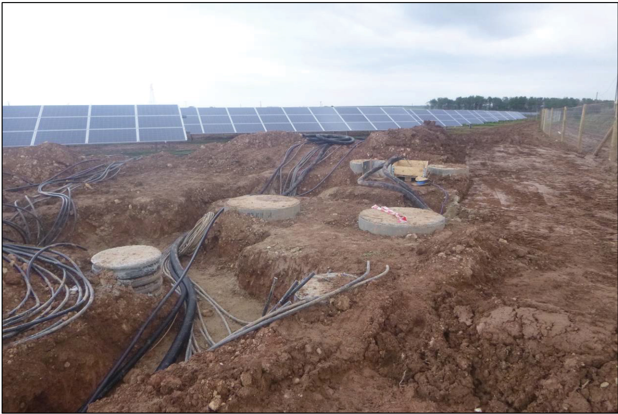
Figure 10: Field F inverter foundation with cable trenches (looking NE)
