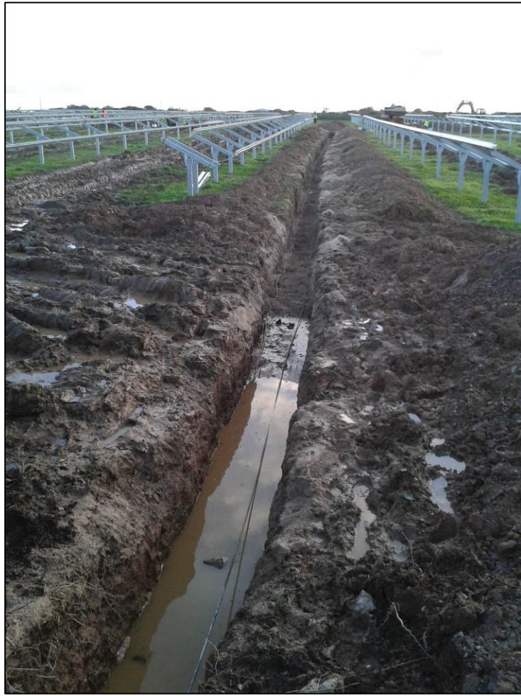
Figure 8: Cable trench in Field B
