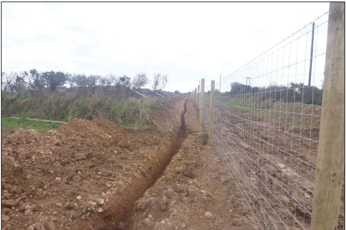
Figure 9: Cable trench in Field C
