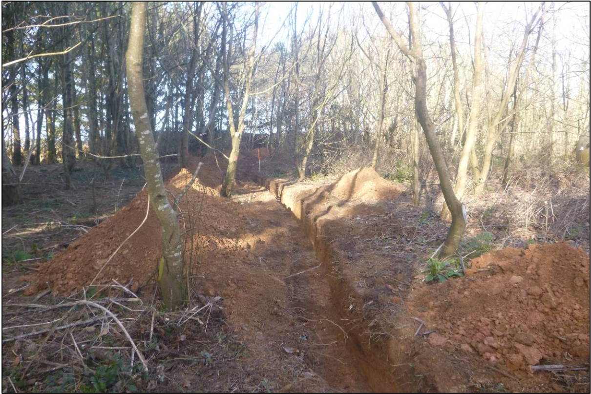
Figure 12: View of cable trench looking NW toward location of ditch (as marked by ranging rod)
