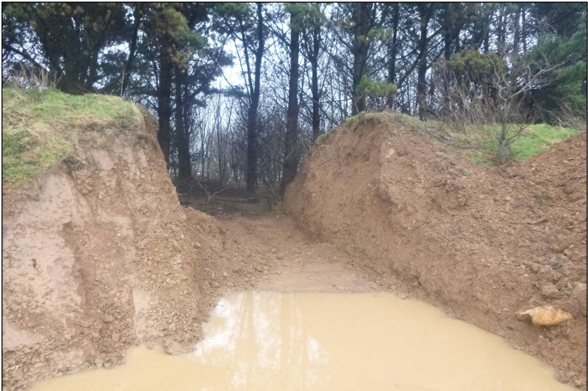
Figure 11: View of breach in field boundary (looking east)
