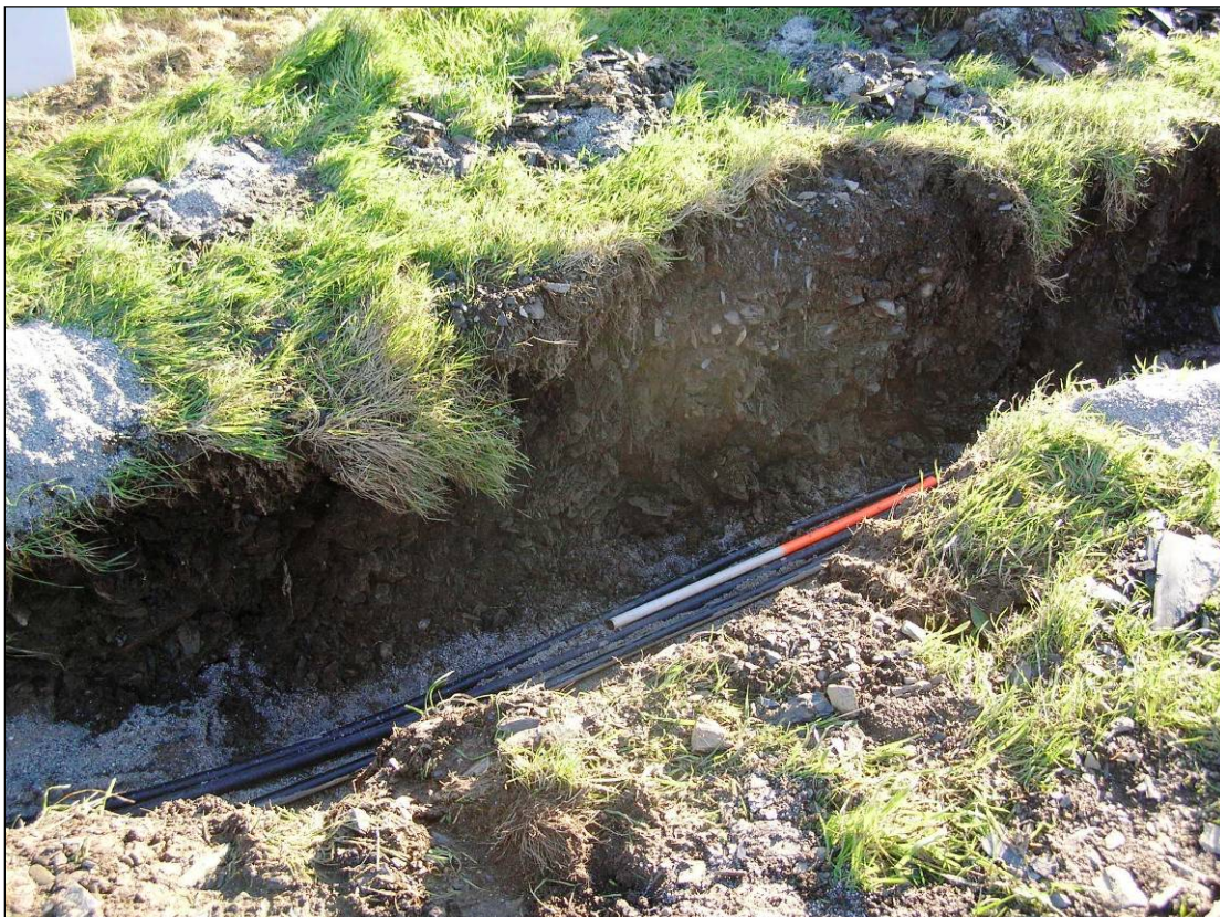
Figure 13 Image (north side) of Section D-D. See Figure 7 for site location. © HE Projects, CC 21/11/2013.
