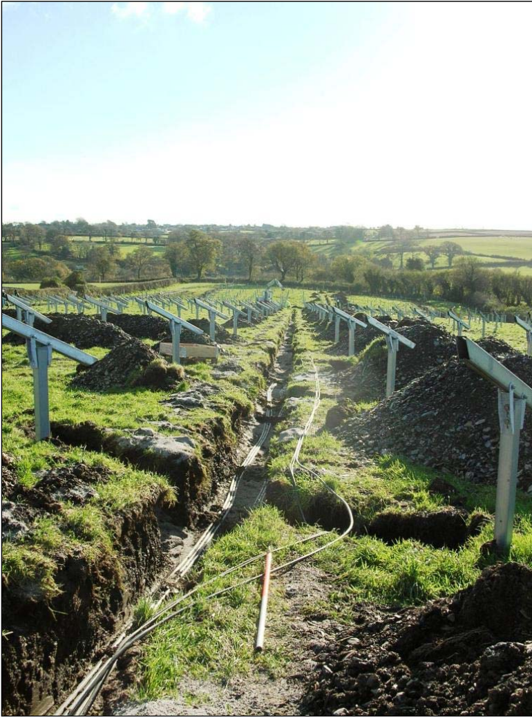
Figure 12 Image (from the north looking south) of field H showing the Type H cable duct trench with inter connecting stringer boxes and partially assemble solar panel frames © HE Projects, CC 21/11/2013.
