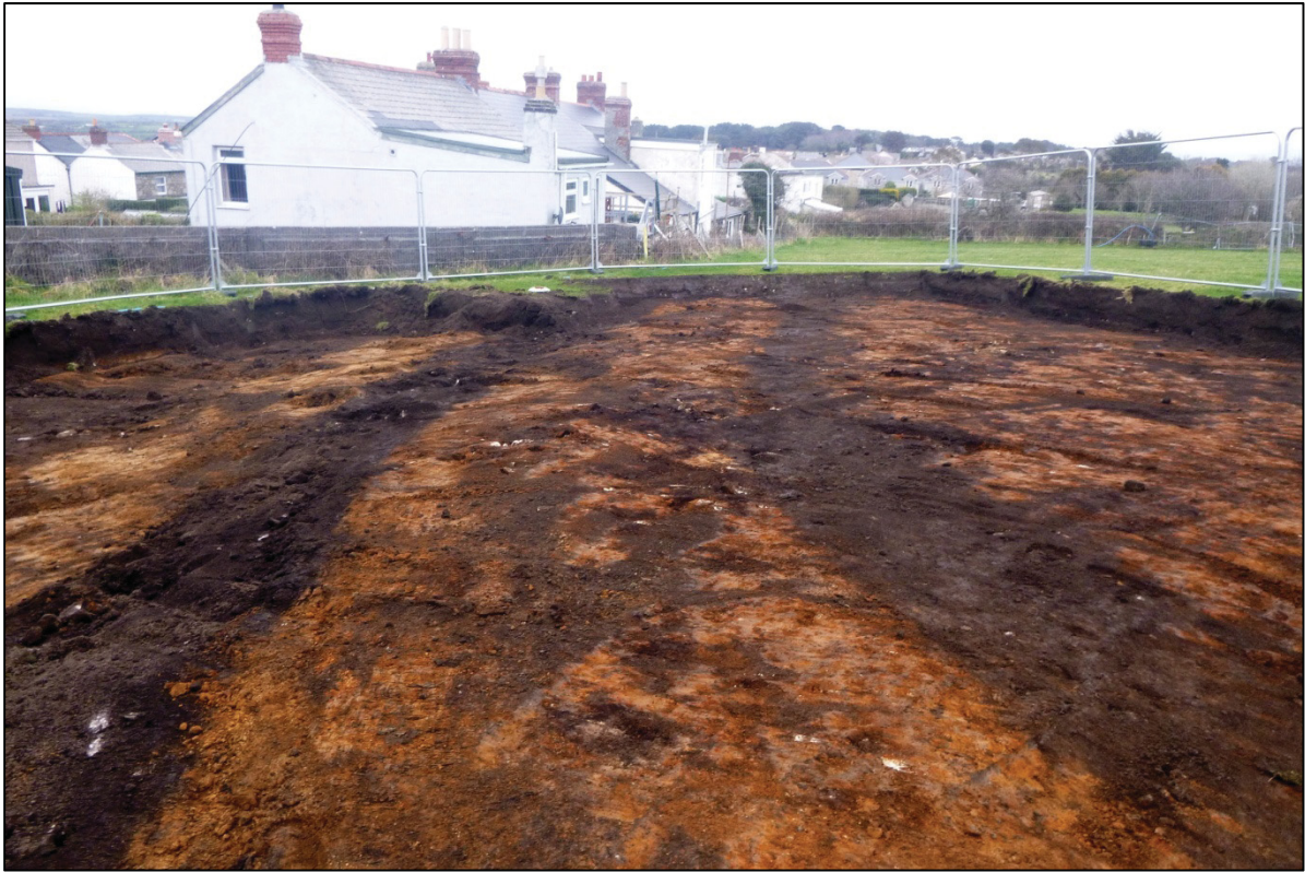
Figure 11: Ditch [113] and shallow ditch [111] once the topsoil had been stripped, view looking north east.
