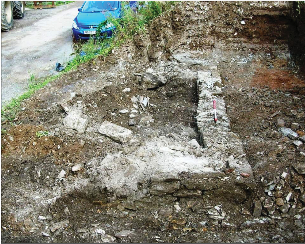
Figure 7 Lower wall foundations of the small building revealed (viewed from the south) © HE projects CC 19/8/2013.
