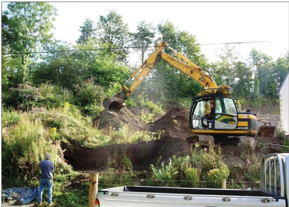
Figure 6 Looking upslope, eastwards at the start of the site excavation © HE projects CC 19/8/2013.
