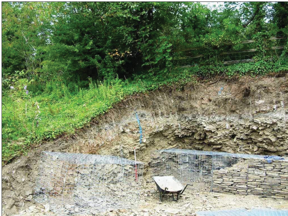
Figure 8 Machine excavations at the north east top corner of the site showing mixed site stratigraphy to shillet/bedrock level © HE projects CC 3/9/2013.
