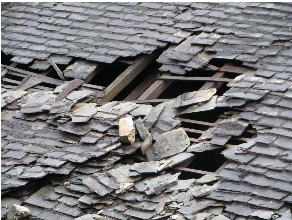
Fig 5 Tolgus arsenic works: the damaged west face of the calciner roof in January 2014: the lower, more detailed, image shows a brick from the flues lodged on the roof
