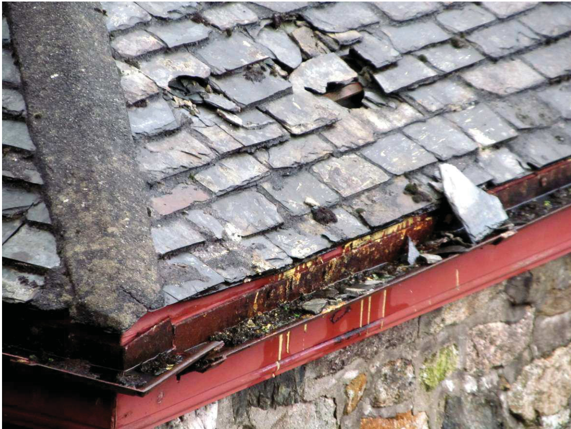
Fig 8 Tolgus arsenic works: missing slates on south face of roof, blocked and broken gutter
