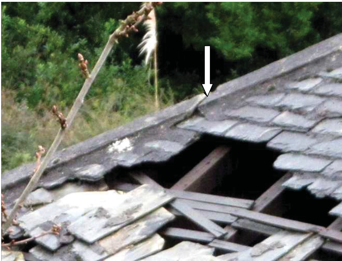
Fig 9 Tolgus arsenic works: cracked cement hip
