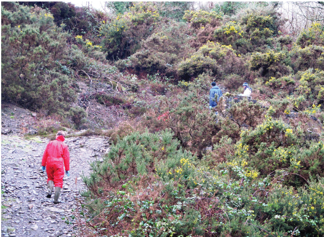
Fig 14 Above: The Conservation Volunteers (TCV) clear rubbish from the upper room of the calciner. Litter picking devices were used and protective suits and gloves worn for Health and Safety. Below: starting to clear vegetation from the flues of the labyrinth
