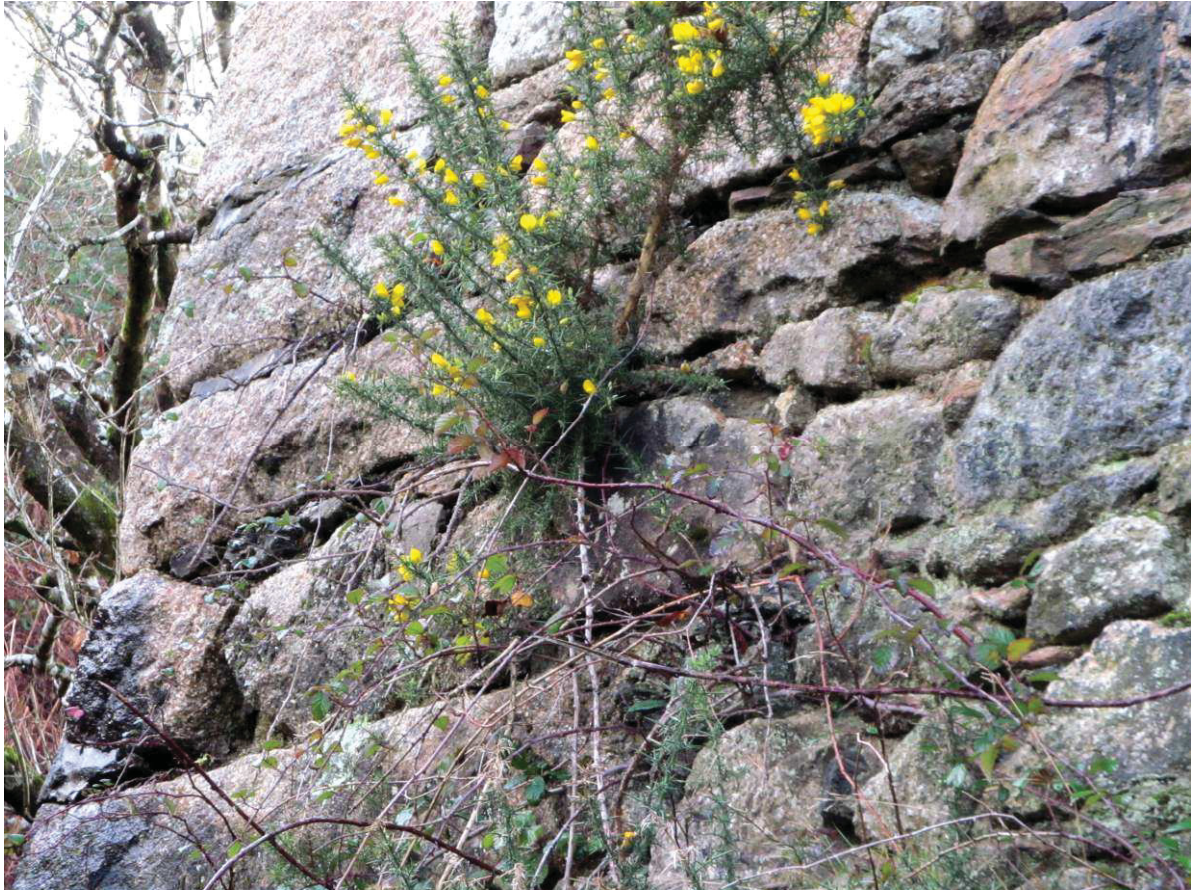
Fig 6 Tolgus arsenic works: vegetation growing from cracks in the stonework
