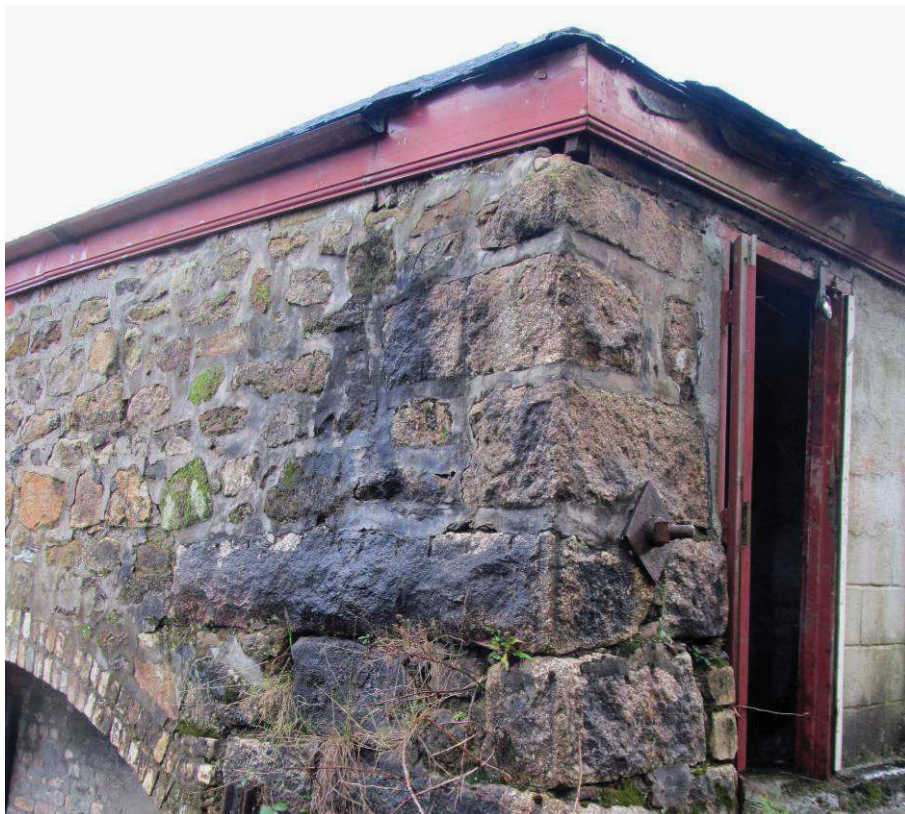
Fig 7 Tolgus arsenic works: missing gutter at NW corner. Water running down the stonework has caused the staining seen on the wall
