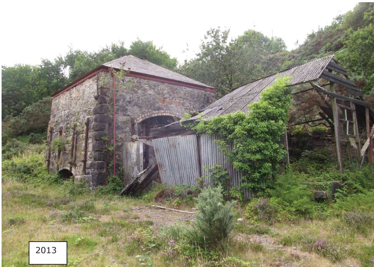
Fig 12 Tolgus arsenic works: the collapsing fuel store beside the calciner in 2011 (above) and 2013 (below)
