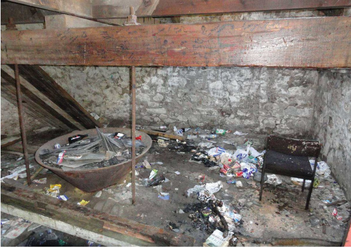
Fig 10 Tolgus arsenic works: rubbish resulting from rough sleeping in the calciner's upper room
