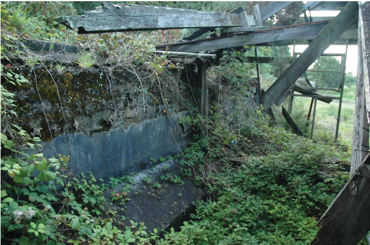
Fig 13 Tolgus arsenic works: the damaged roof of the fuel store (photos: John Gander)
