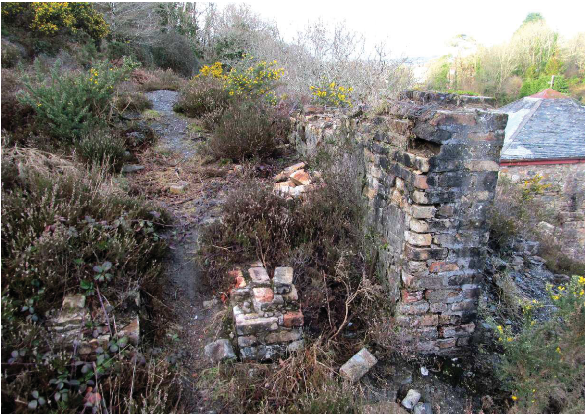
Fig 11 Tolgus arsenic works: the damaged and collapsed brickwork of the flues
