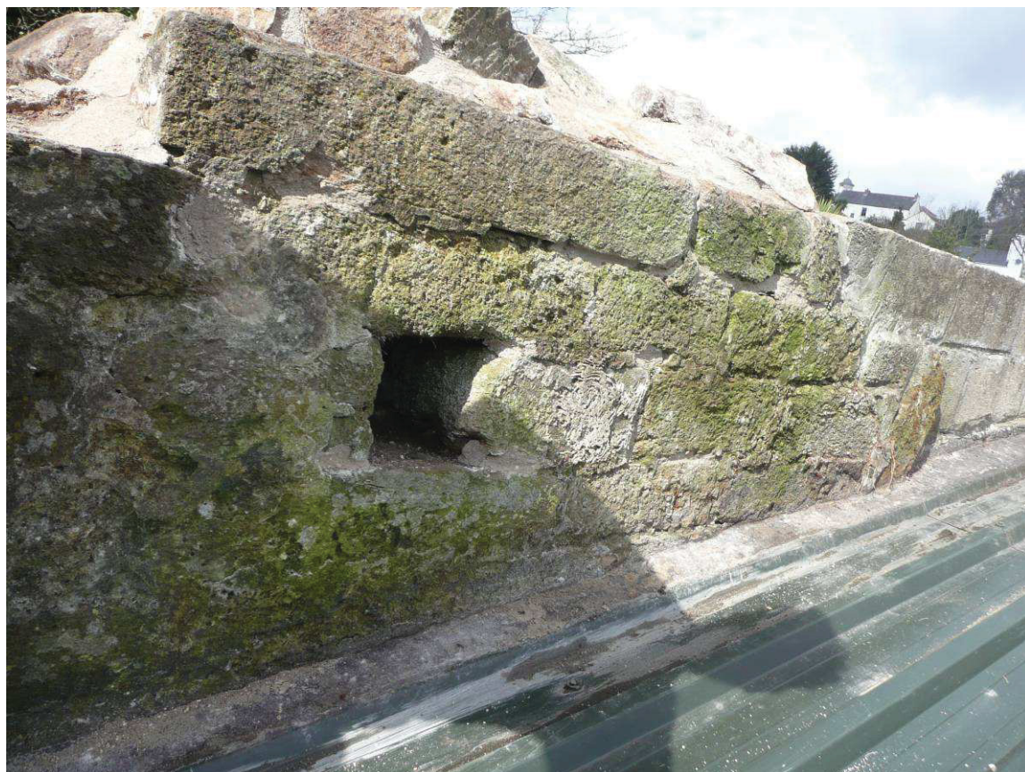
Fig 14 The east face of the wall visible above the workshop roof, with external ashlar face extant and putlog hole visible
