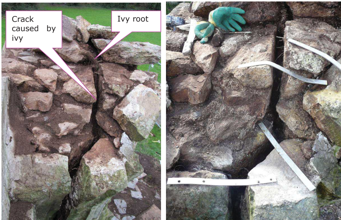
Fig 12 On the left, the crack caused by ivy and on the right the strapping fixed to stop any further movement of the crack. The crack was filled with stone and mortar and a wall capping was then built over this to hide the strapping and help shed water from the wall-top
