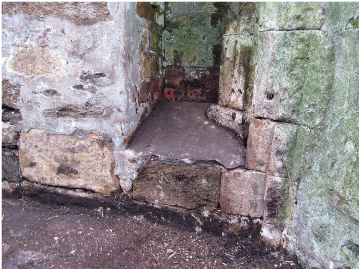
Fig 13 Above: detail of north side of window, in Bohl's Yard, beside the oil tank which has now been removed; and below: detail of the sill, also in Bohl's Yard, before removal of concrete
