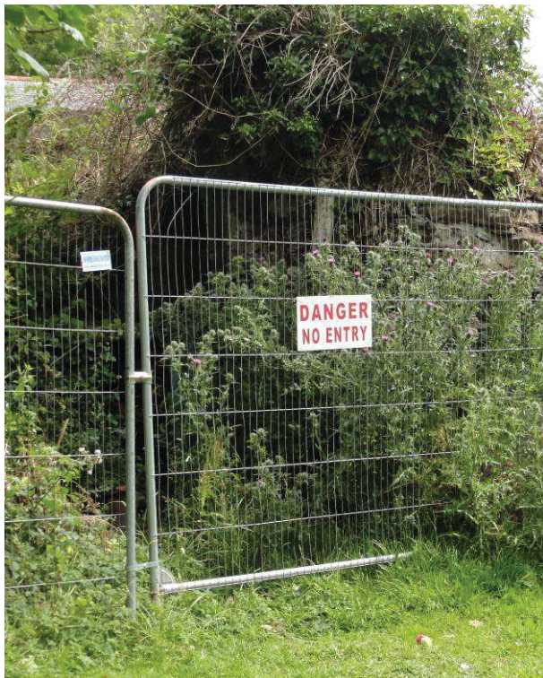
The wall behind the security fence and hidden by ivy
