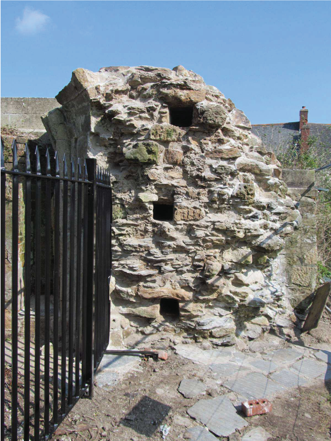
Fig 18 The almost completed project. The slate plinth can be seen at the base of the wall. This has now been covered over to protect it.
