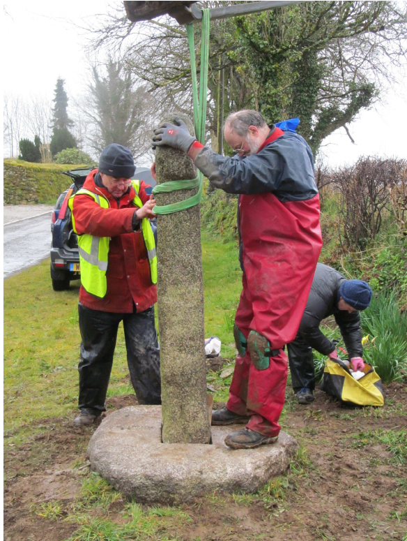
Above left: Andrew Langdon and Lawrence Kelland setting the cross in its new base
