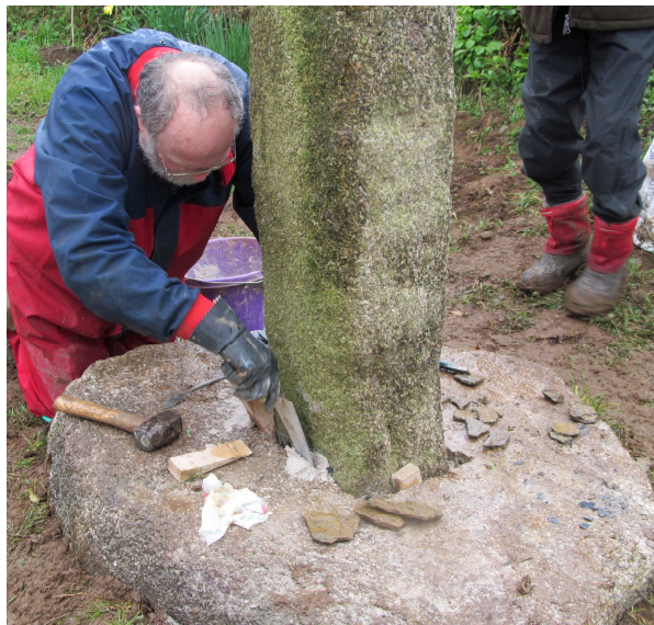
Below right: Lawrence Kelland uses lime mortar to fill the joint between the cross and the base
