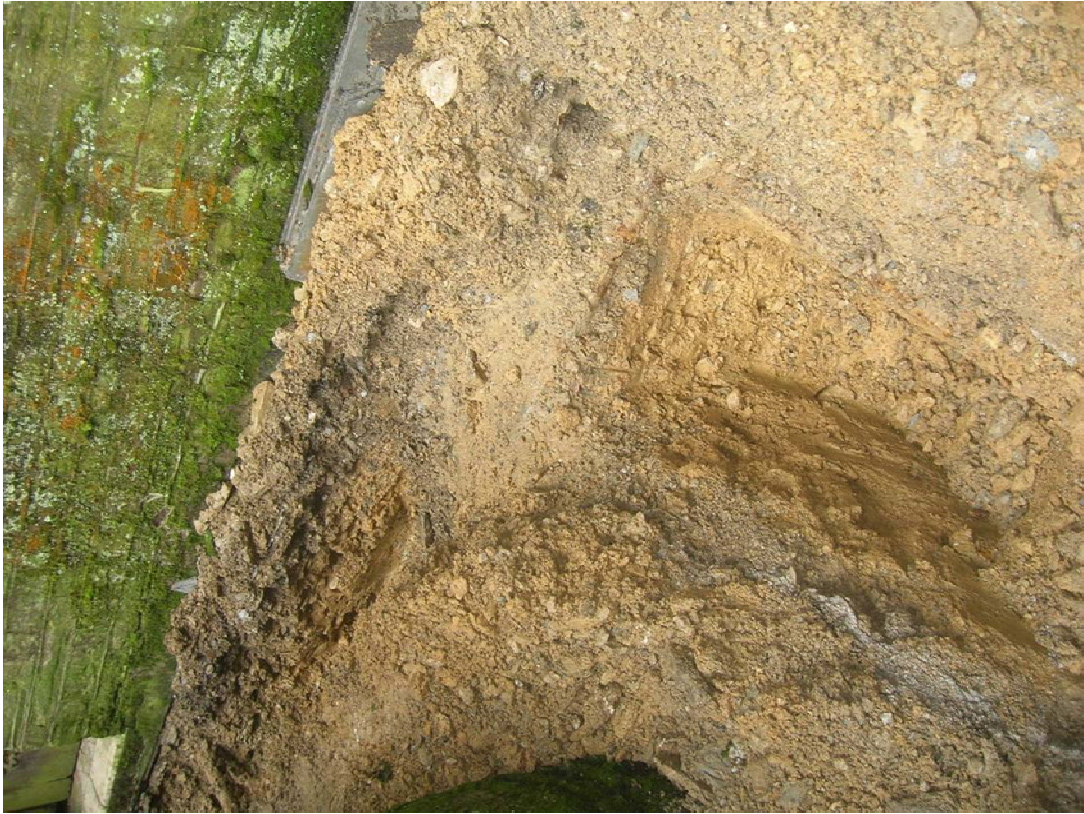
Figure 13. Sample section along east spur of the trenches showing nature of ground encountered.
