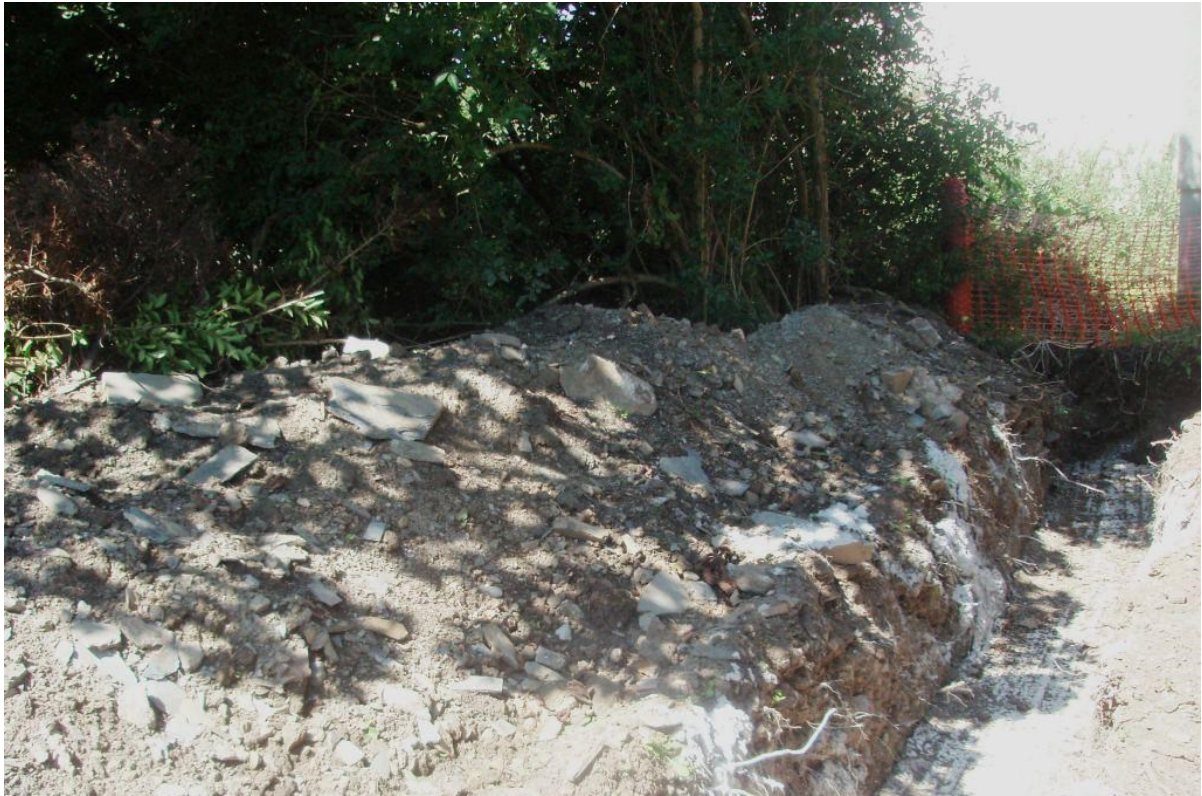
Figure 7: The excavated trench and spoil, note the high quantity of modern debris and rubble.
