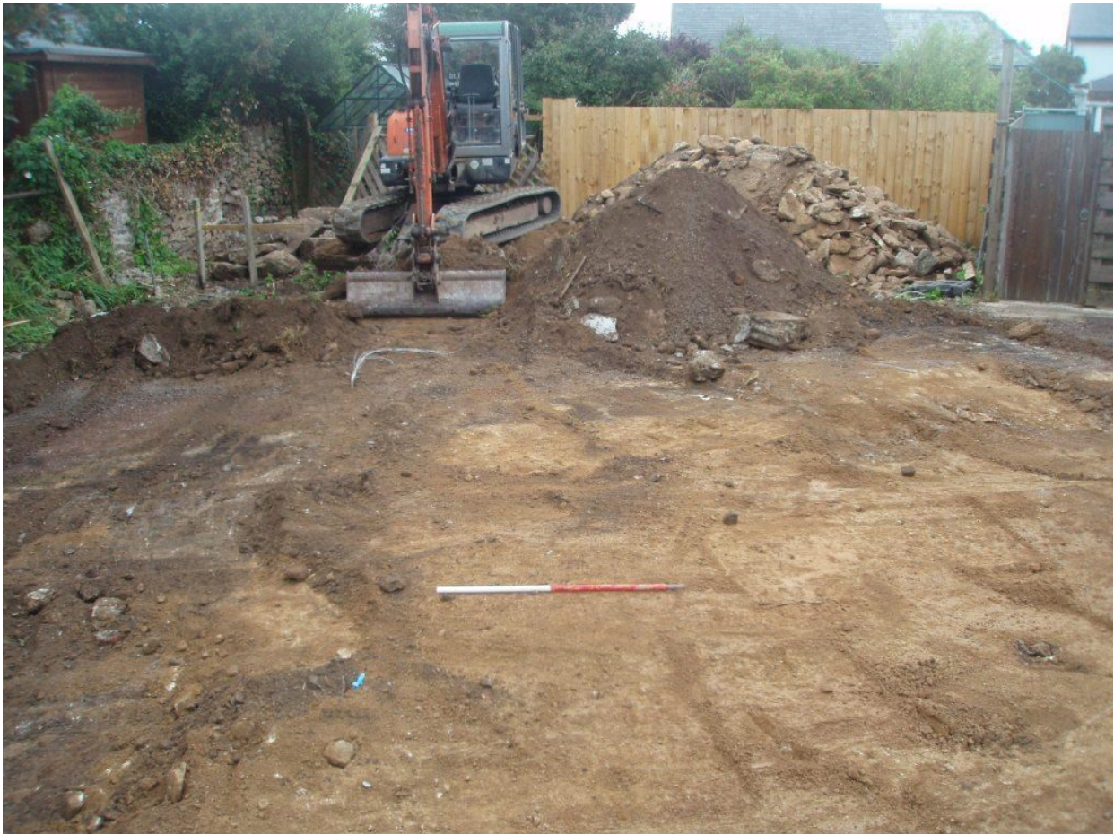
Figure 7: The excavated area prior to completion with the dark oil staining and unexcavated gravels on the left of the image and large quantity of rubble and debris in the background which was cleared from the site.
