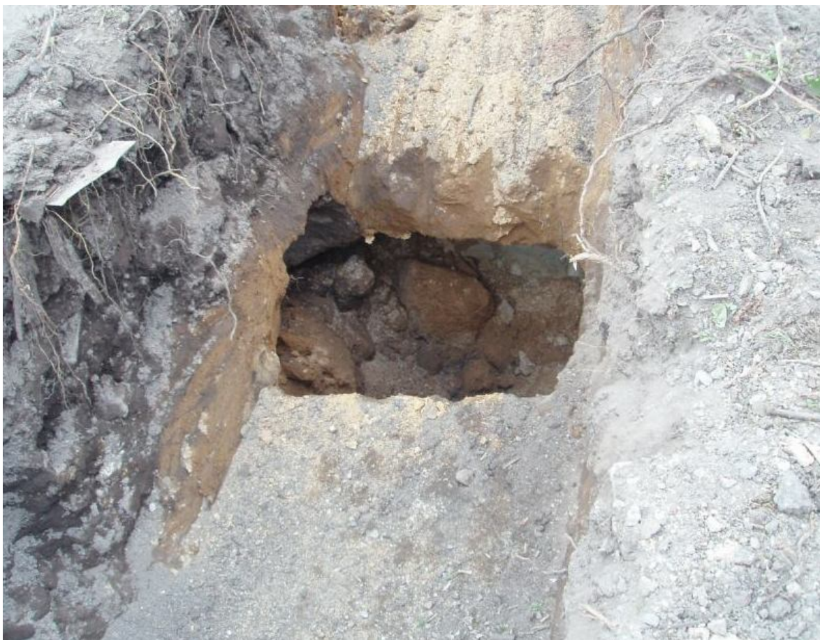
Figure 10: The void, probably caused by progressive roof collapse in a mining lode, that opened below the foundation trench.
