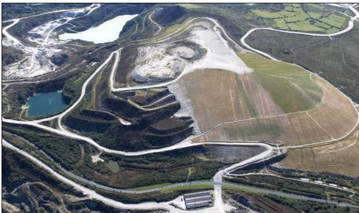
Figure 73 Re-profiling and re-vegetation of modern stepped china-clay waste tips in progress on Hensbarrow Downs in 2009. The characteristic form of the tips created by the modern industry is almost entirely obliterated, leaving a smoothed and rounded landform which shows little of the topographical characteristics of south-western granite uplands. The Bronze Age Hensbarrow (top right), formerly the third highest point in Cornwall and a prominent landmark in the region, is now overtopped and dominated by the tip (cf Fig 47). (Photograph: Historic Environment, Cornwall Council: F95-025; 10 September 2009.)
