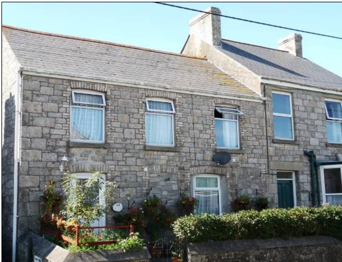
Figure 84 Granite and brick, the latter almost certainly from local brickworks, used on the elevations of late nineteenth-century houses in Fore Street, St Stephen-in-Brannel. (Photograph: Graeme Kirkham.)
