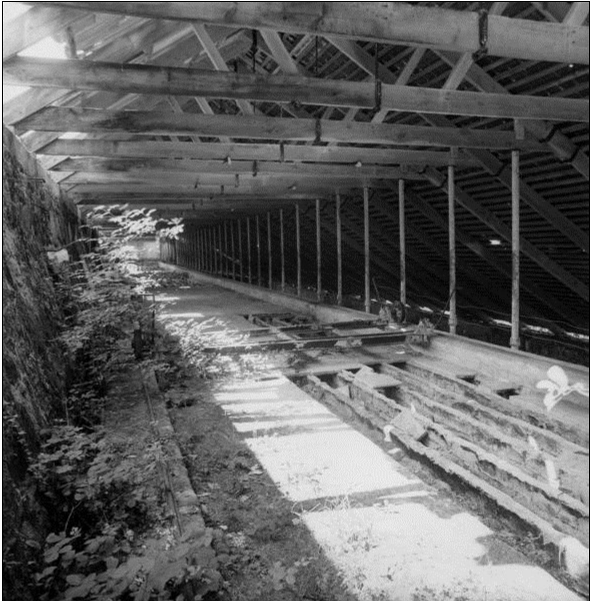
Figure 37 The drying floor and travelling bridge (used for distributing semi-liquid clay across the drying floor) at the derelict Carlyon Farm china-clay dry in the Trenance valley, near St Austell. It was completed in 1921 and was reputedly the largest pan kiln ever built. The photograph dates to between 1968 and 1984. (Photograph: ECC archive, held by the China Clay History Society.)
