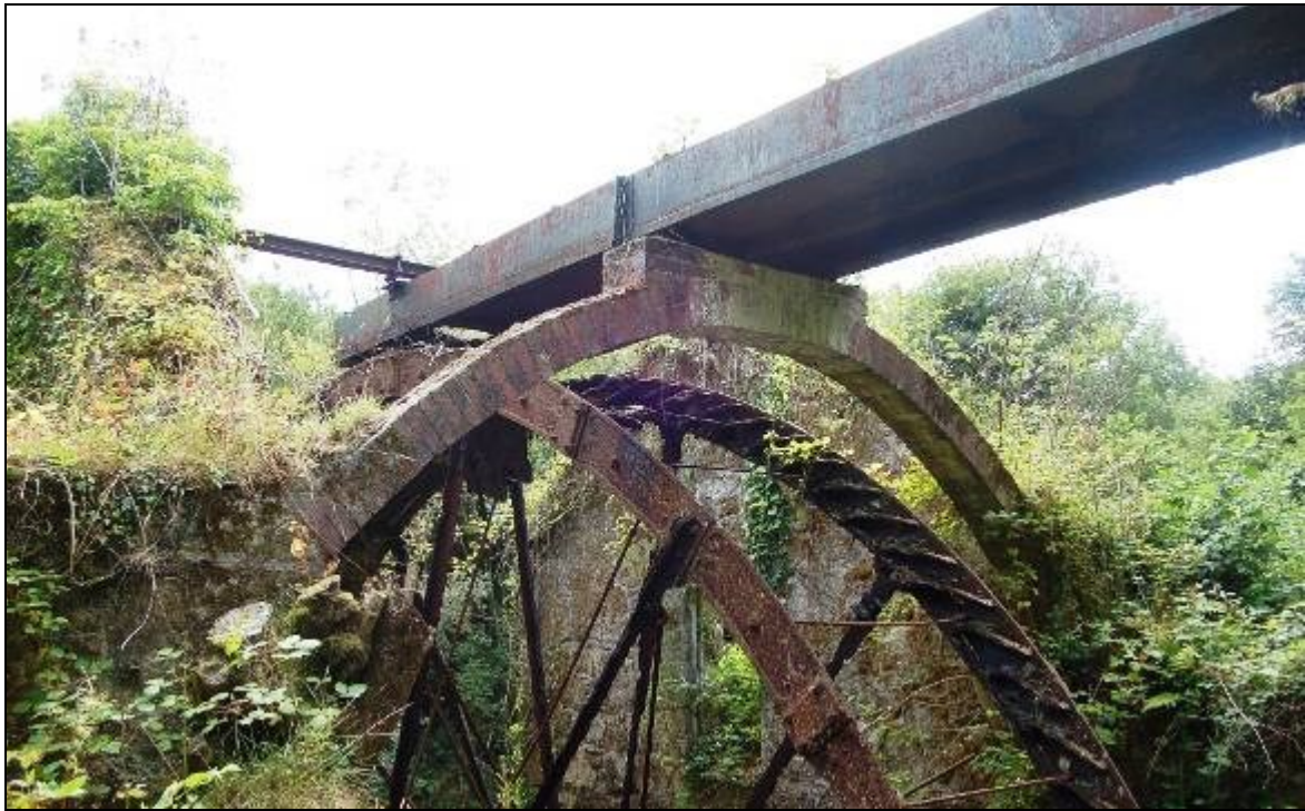
Figure 99 The remains of an overshot water wheel and launder at Big Wheel china stone mill in the Tregargus valley, photographed in 2006. The complex, built about 1898, is a Scheduled Monument and a Grade II Listed Building (Cole and Smith 2002). (Photograph: Historic Environment, Cornwall Council.)
