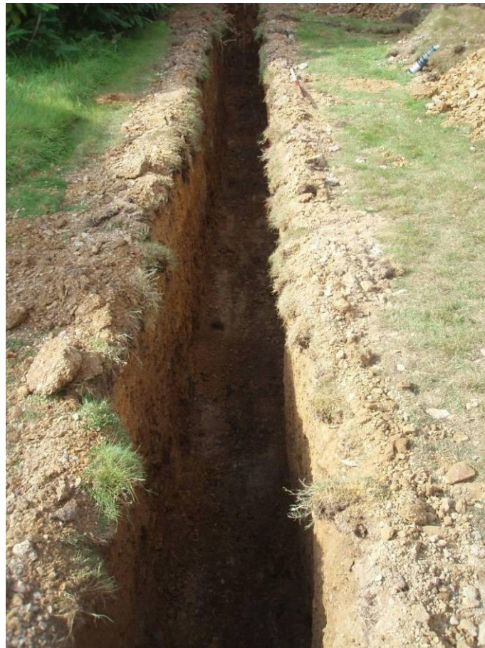
Figure 18: The excavated drainage trench. Note the shallow depth of the turf and topsoil and the gravel, visible to the sides of the trench.
