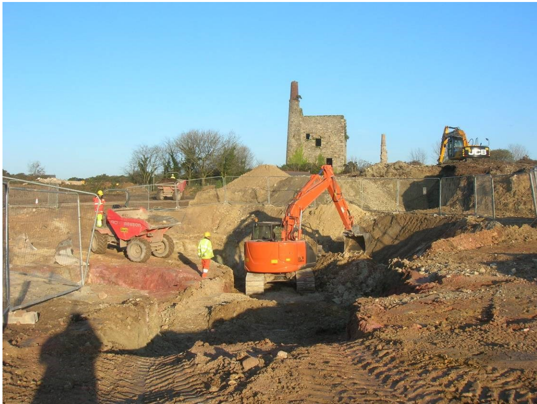
Figure 30. Hallenbeagle West. Openwork [249]. Excavation in progress with the swing shovel sitting completely within the feature.
