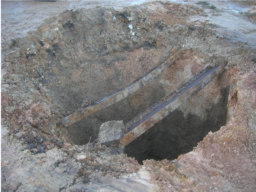
Figure 26. Hallenbeagle West. Shaft [125] after removal of capping showing the steel beams which had supported its concrete cap.
