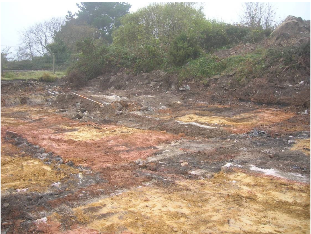
Figure 24. Hallenbeagle East. Area 3. Footings of sawmill [313]. Part of north-west side (see fig 22). Scale bar = 2.0m.
