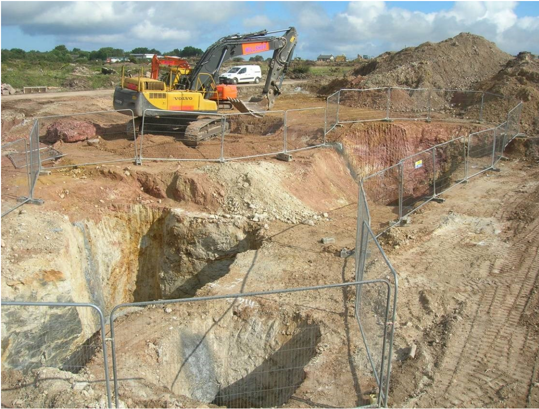
Figure 17. Hallenbeagle East. Outcrop shafts [116], [117], [126], [127] and [128] to the south of Shaft [17] which is in the process of being excavated.
