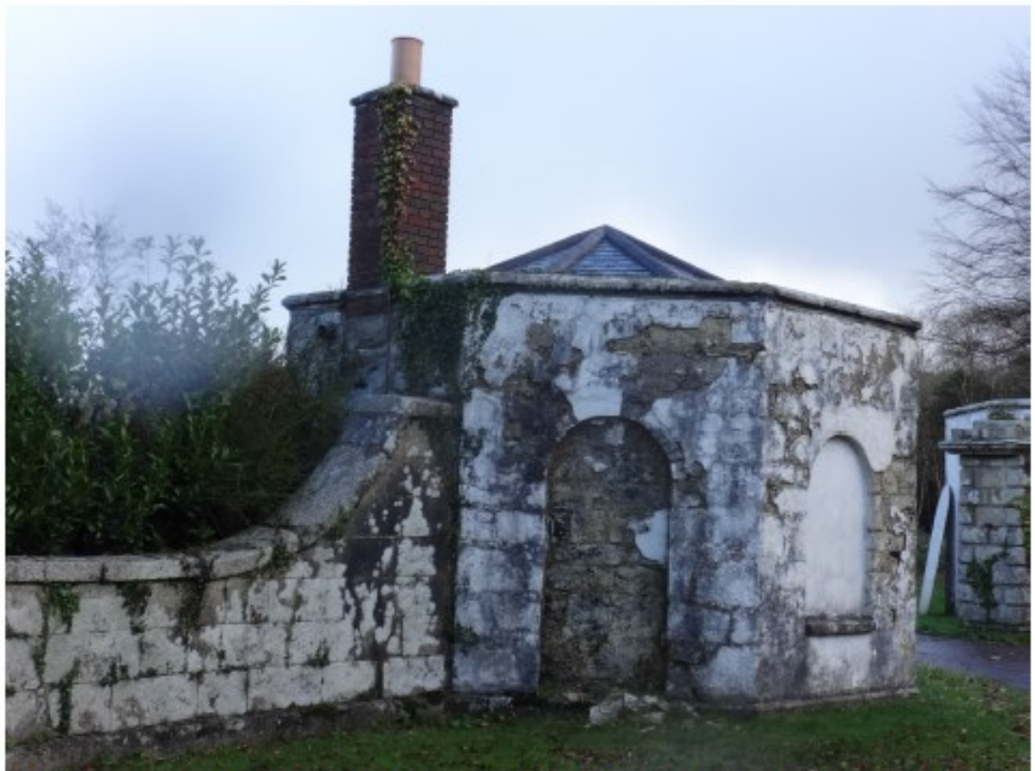
Figure 3. NW Lodge showing degradation of the render finishes and underlying stonework, November 2014
