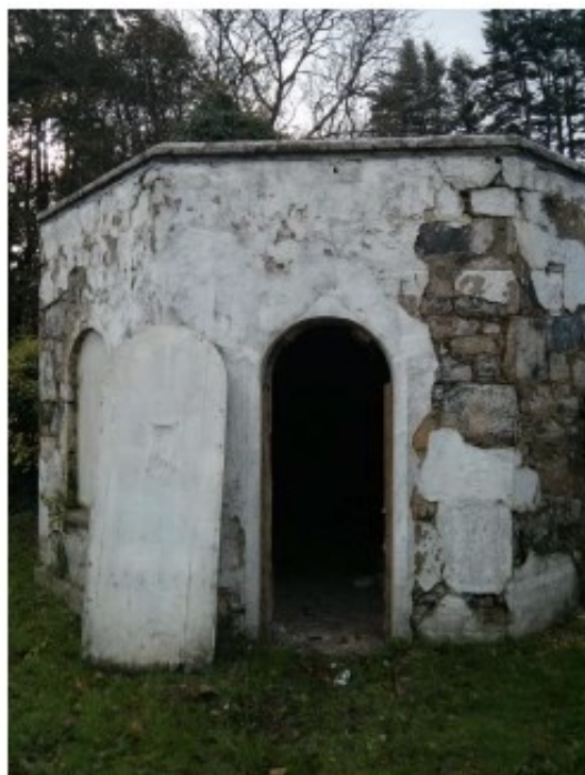
Plate 1: General view of entrance elevation showing missing sections of render.
