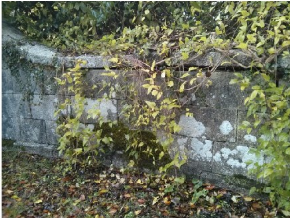
Plate 8: Displaced coping stones.
