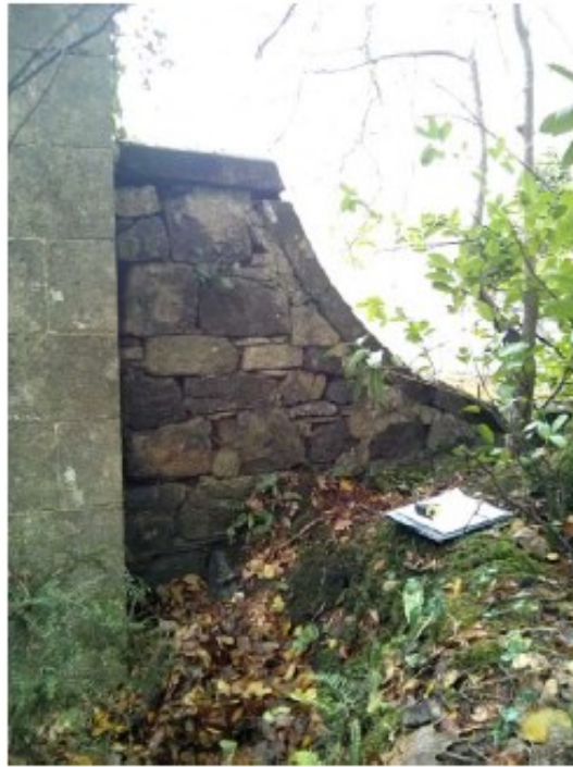
Plate 9: Mortar loss to wall adjacent to terminal pier.
