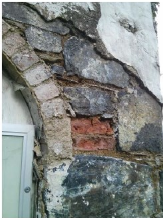
Plate 6: Damage to brick arch and missing render.
