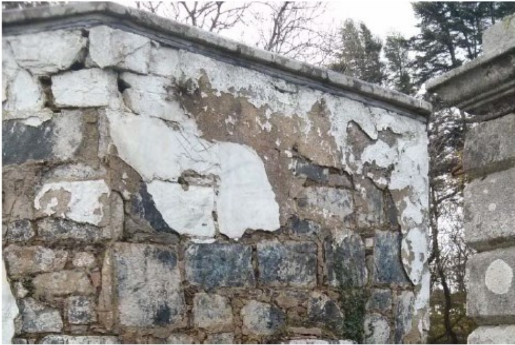
Plate 5: Displaced stone at parapet level. Note large areas of missing render.
