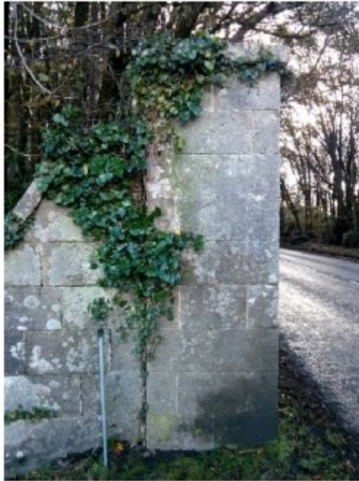
Plate 13: South East Wall Terminal Pier (showing lean)
