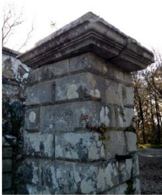
Plate 15: Granite Gate Pier (Note displaced cap stones)
