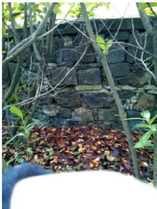
Plate 12: Mortar loss to rear face of North West Flanking Wall.
