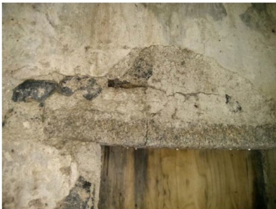
Plate 2: Crack to underside of granite lintel.
