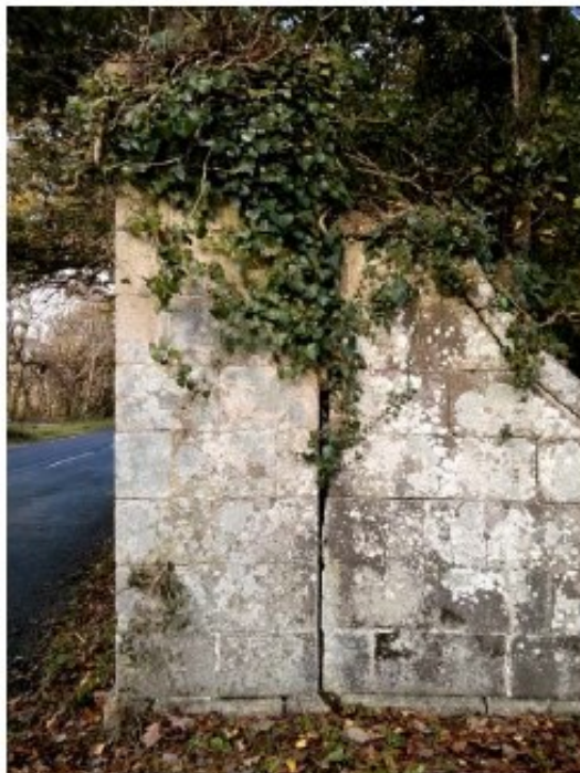
Plate 14: North West Wall Terminal Pier (showing lean)
