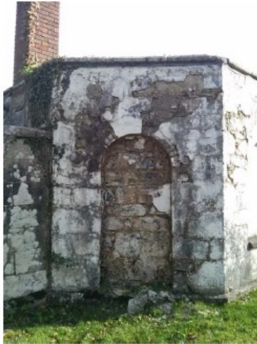
Plate 7: Fallen areas of render, note ivy growth at eaves.
