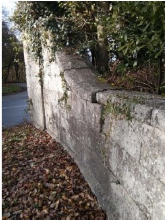
Plate 11: Displacement to North West Flanking Wall.
