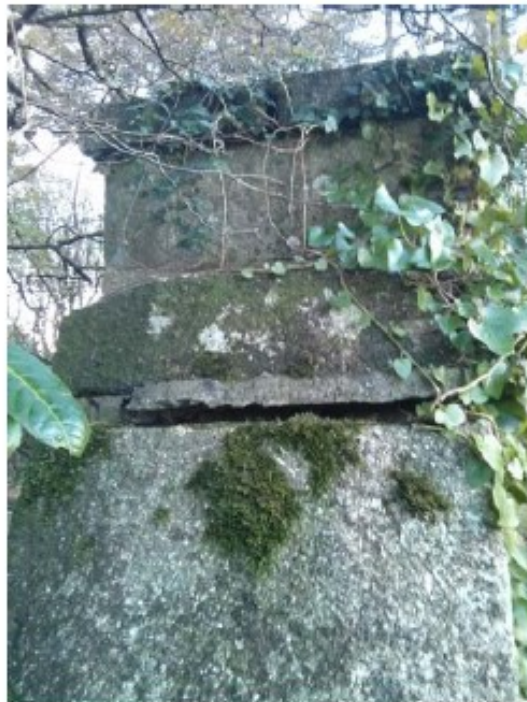
Plate 10: Coping stone in need of rebedding.
