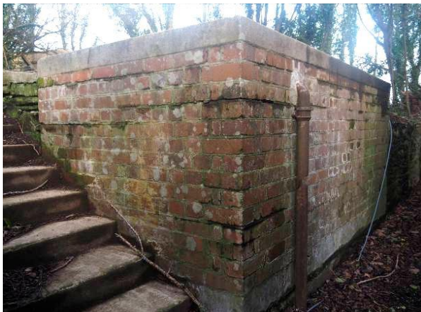
Fig 71 Rainwater tank and steps to rear laundry drying garden.
