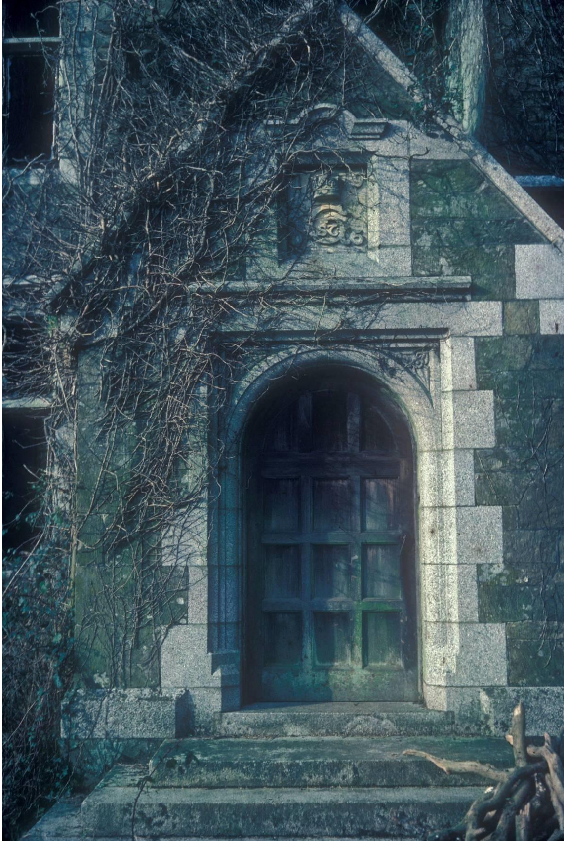
Fig 9 Overgrown entrance porch (still with extant original wooden door) at Penmadow c1988.
