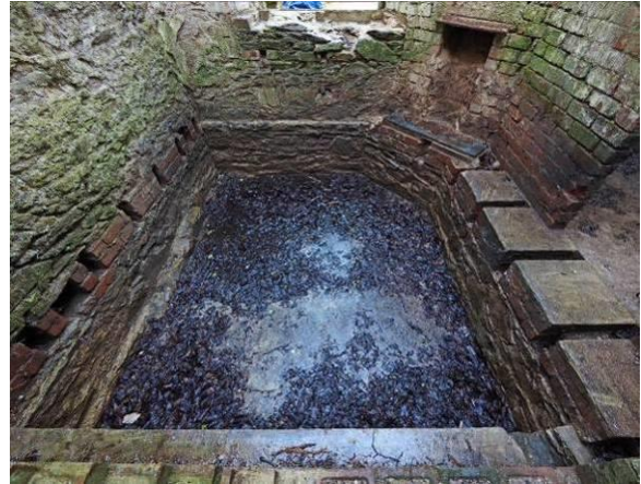
Fig 62 Butler's pantry suspended floor remains.
