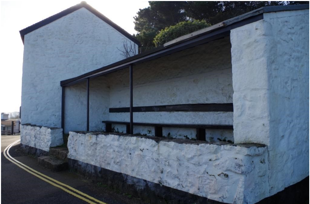
Figure 8: The northern range open shelter with granite steps and benches. The graffiti on the bench and poor roof repair are just visible.
