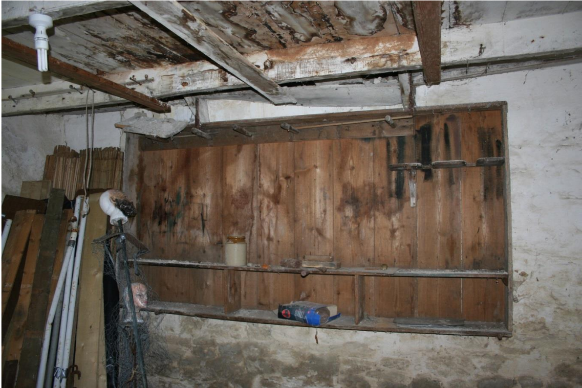
Fig 22 Rack on the west wall of the western store with pegs and shelves, possibly for equipment used in the stable and carriage house range built on to the north c1850
