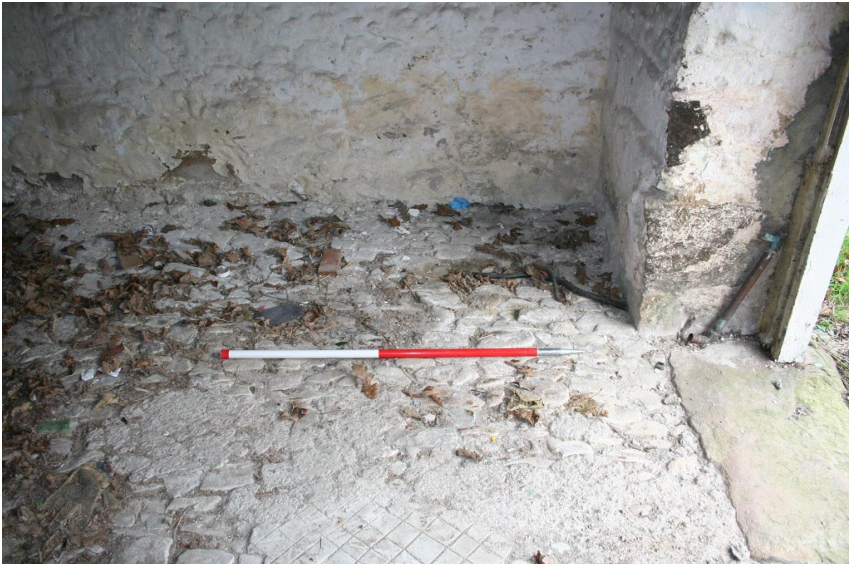
Fig 53 Floor in north east corner of Carriage House showing cobbling with wear patterns and limited modern repair, and one of the irregular threshold slabs of local stone
