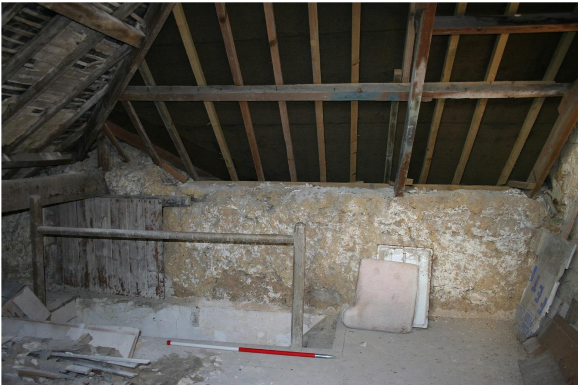
Fig 23 North side of loft in the western store, with limewashed cob walls, window (boarded up), secondary staircase, and church fete signboards of the later 20C
