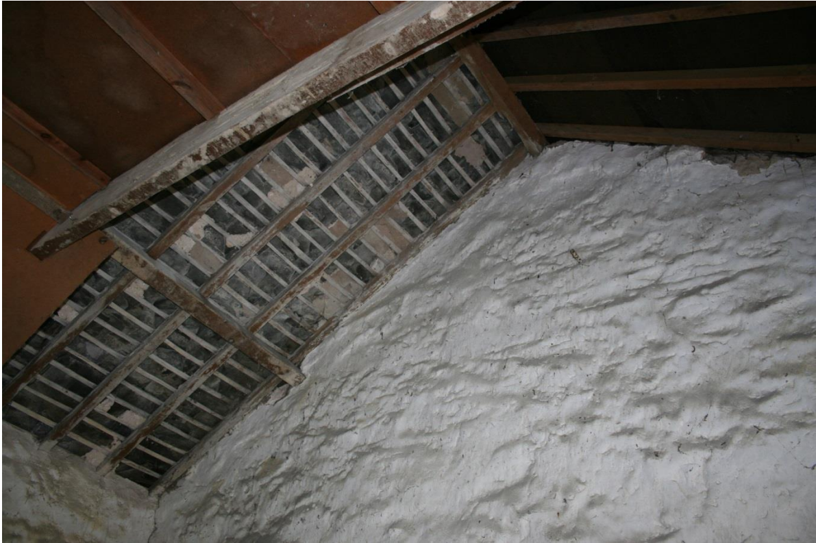
Fig 52 Detail of traditional roofing work at north end of west side of Carriage House
