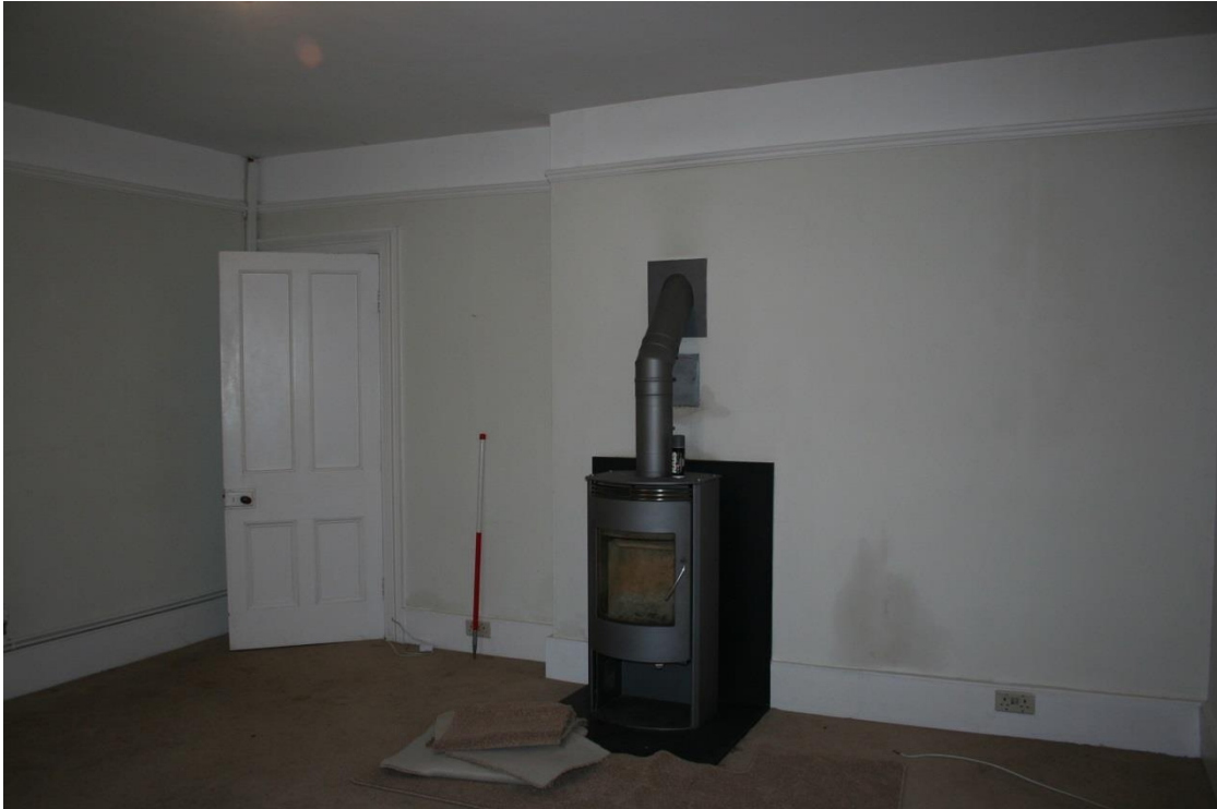
Fig 32 North wall of drawing room of c1850, with doorway giving access from the passage down the rear, west side of the south wing, and stove by a blocked fireplace
