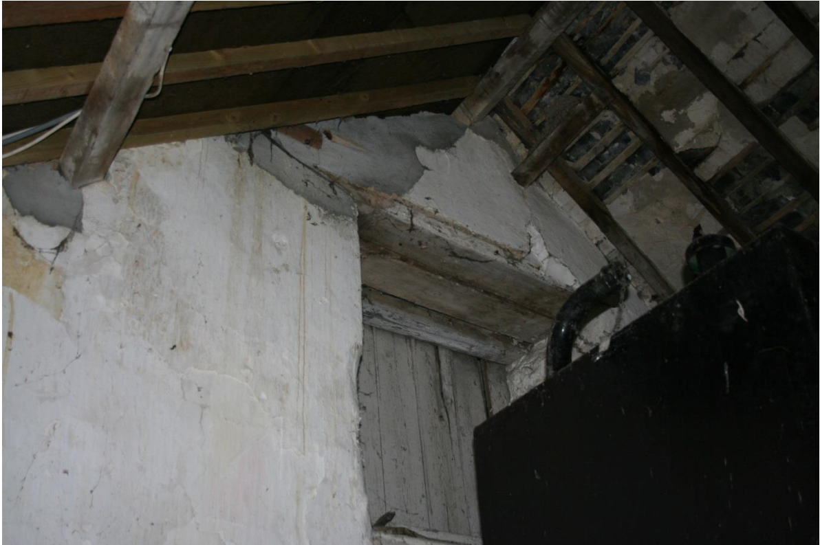
Fig 26 North window of loft over western store, originally opening to the rear court, seen from the stable built against the store c1850 with later oil tank in it (right)
