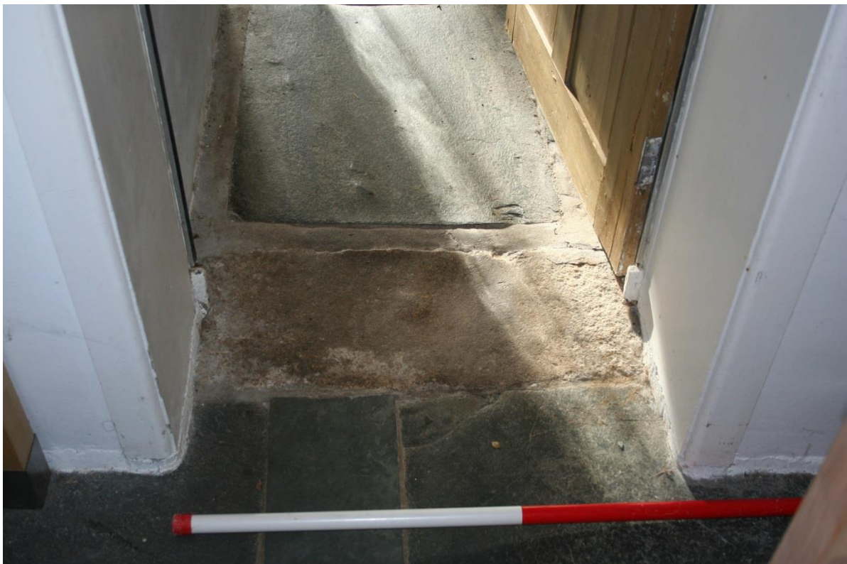
Fig 13 Threshold to Kitchen from the scullery (the [back] 'kitchen' of 1727 and 'flesh house' of 1680), showing granite slab worn in the centre with shoe sized hollows
