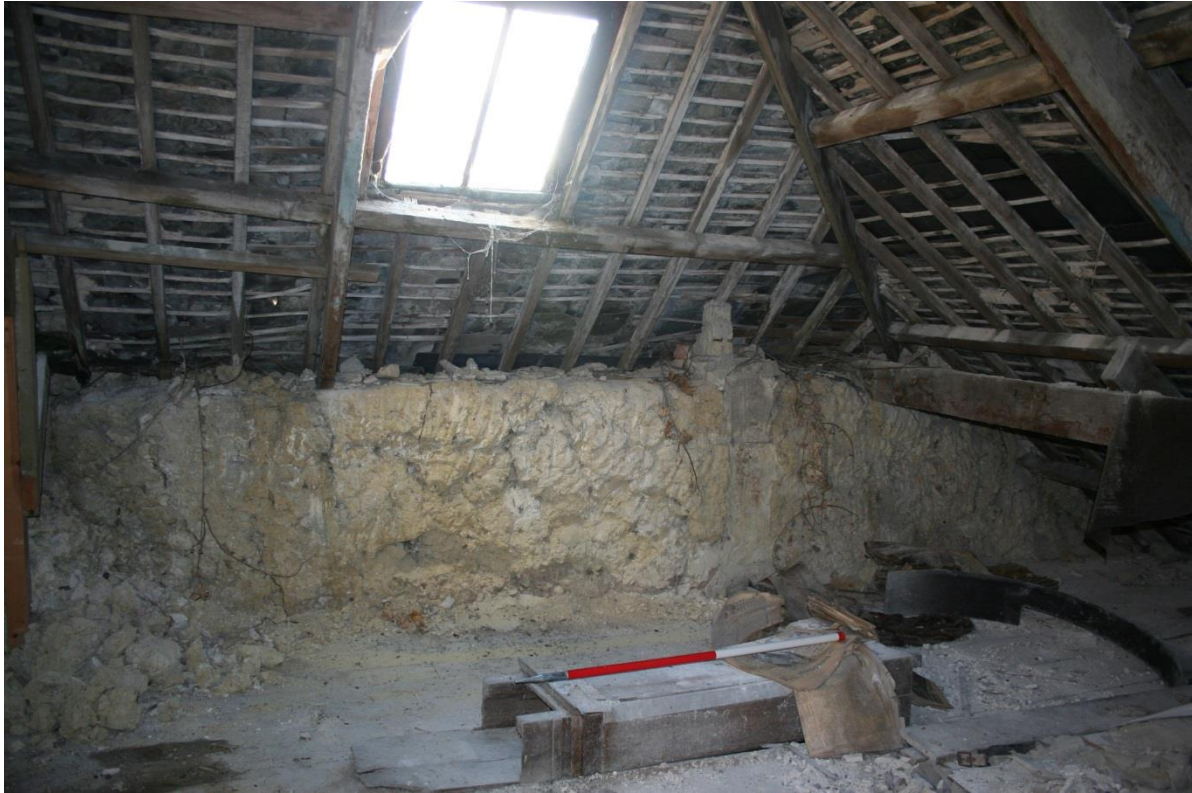
Fig 24 South side of loft in the western store, showing torched scantle slate hipped roof, broad floorboards, and abandoned clock case (with a newspaper of 1976!)
