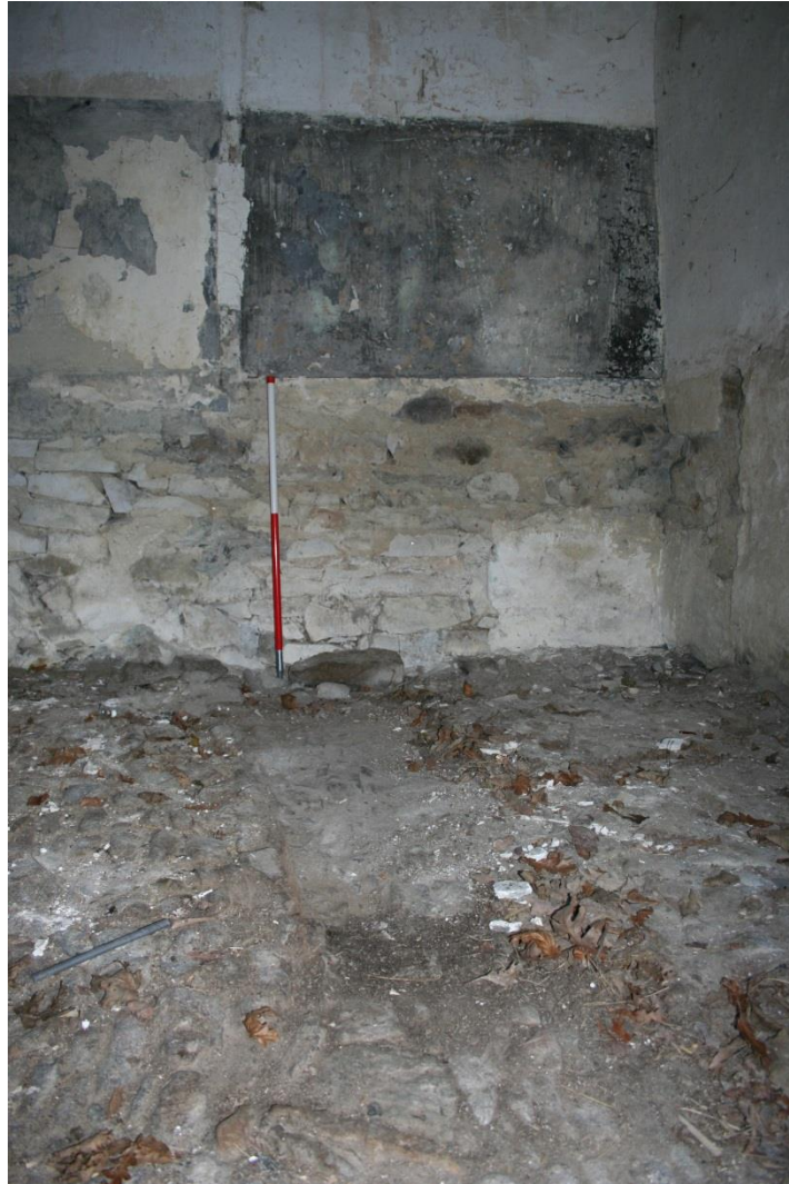
Fig 44 North stall of Stable, looking west to the 'head' end, with traces of stall partition, boarding, and varying wall finishes, and cobbled floor, here very well-preserved
