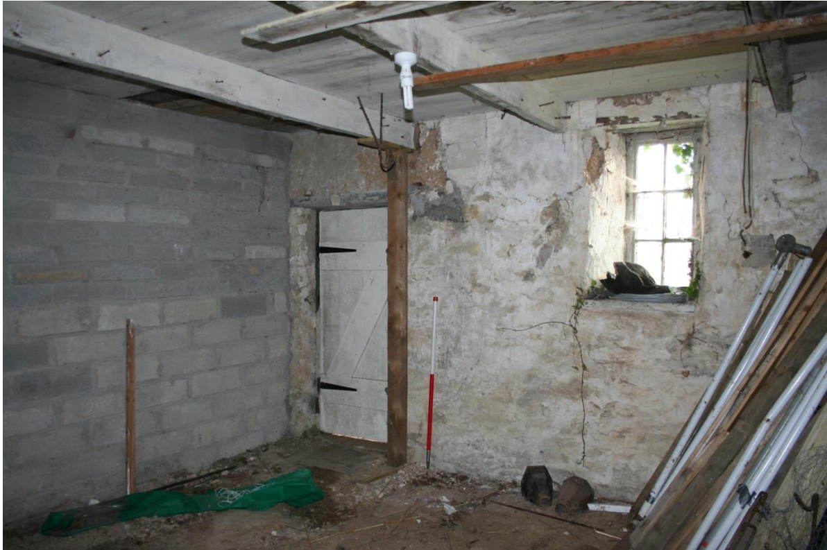
Fig 20 Western Store, showing cob fabric above door level, and rab floor as noted in the house in 1727 (under derelict later boards), and 20C wall to coal store (left)
