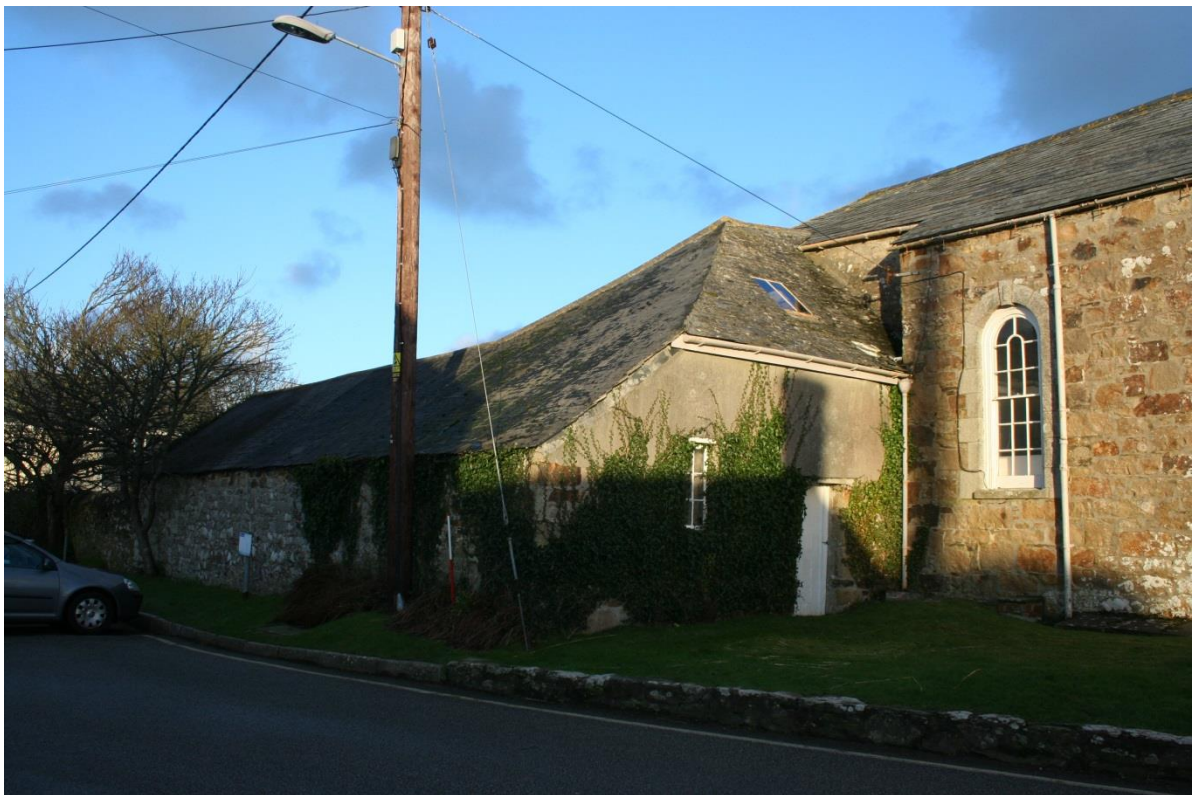
Fig 19 Lean-to store with loft under a hipped scantle slate roof on the west of the early house (centre), flanked by the mid-19C south wing (right) and stable range (left)
