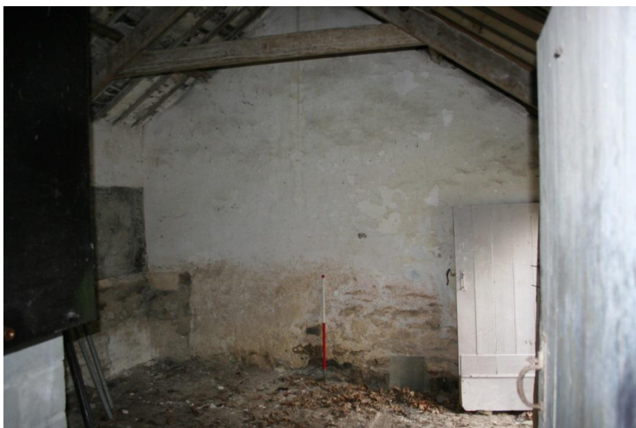
Fig 45 North stall of Stable from the south, showing torched scattle slate roof with the headroom needed for horses, and the fall of the cobbled floor necessary to drain it
