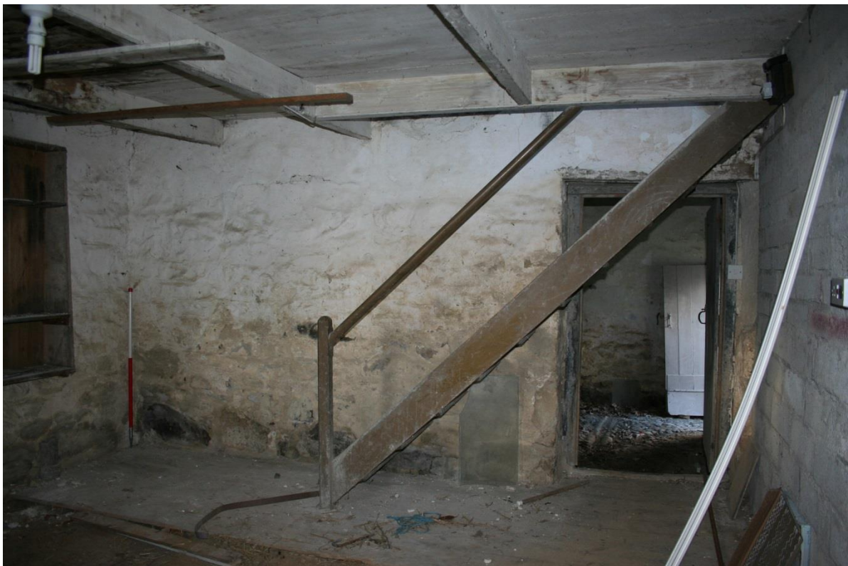
Fig 21 Western store with north door, used c1850 to link it to the new stable wing, beyond, behind secondary stair to loft; note also rack fixed to the west wall (left)
