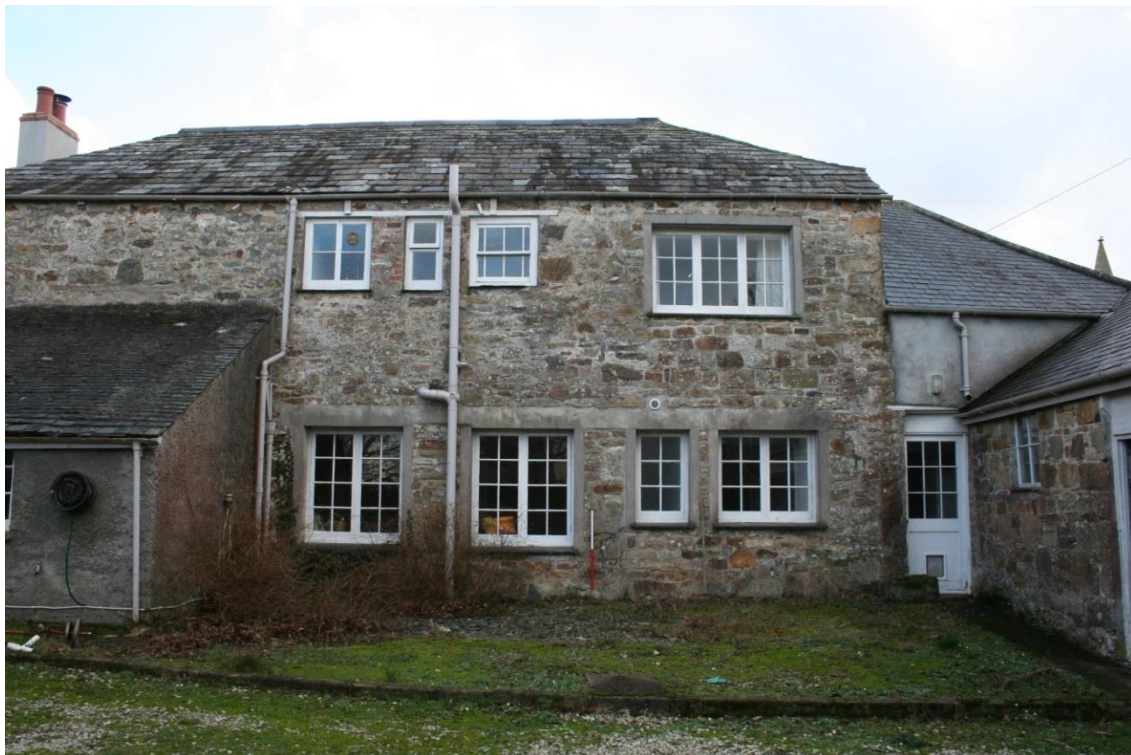
Fig 5 Rear of early range, dominated by modern openings around a Victorian window over the stairs, centre top (with kitchen lean-to, left, and Victorian stables, far right) Its western store, with secondary door later used to access a coal store, is to the right
