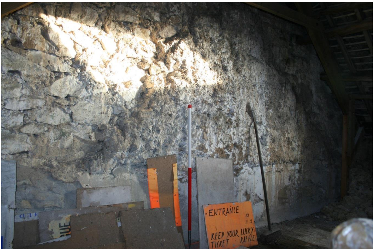
Fig 3 Upper exterior of the early Vicarage's west gable, seen from the adjoining store loft, showing cob-over-stone construction (centre), with later masonry heightening
