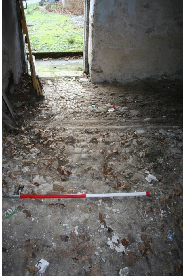
Fig 48 View from north stall across passage to east door of Stable, showing near-intact cobbling laid to fall to a drainage channel at the passage, and to curve to the door
