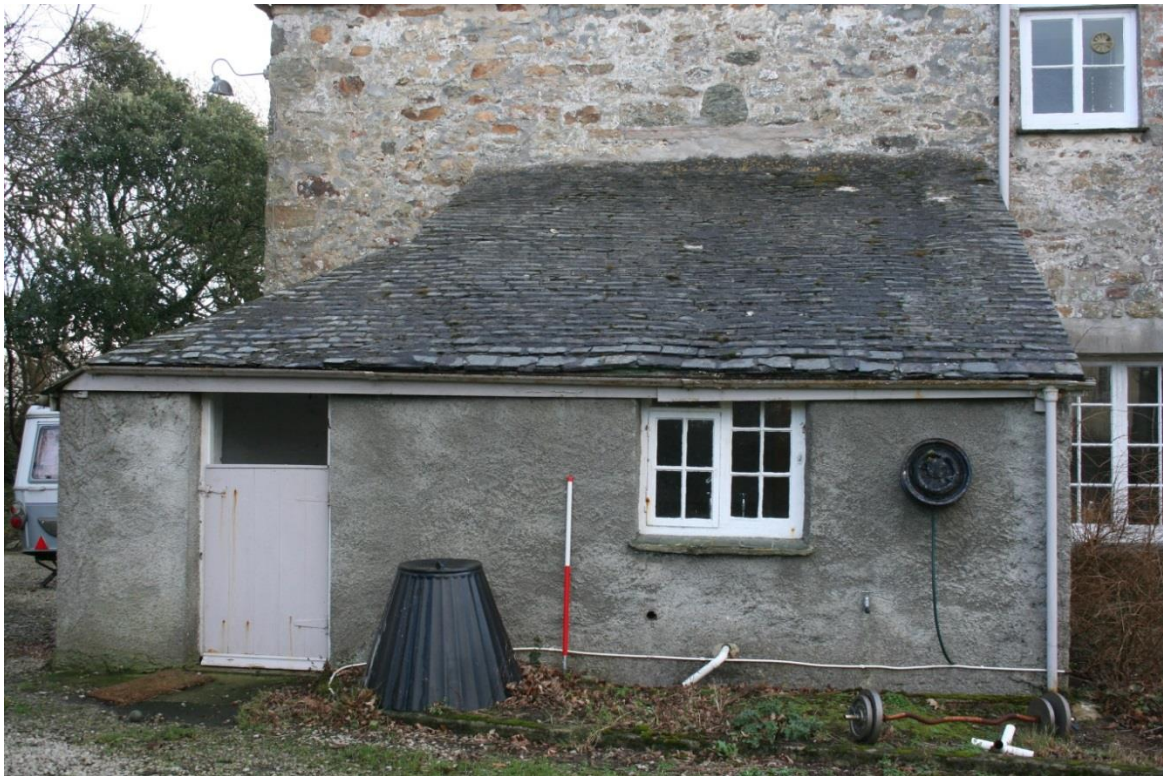
Fig 10 Kitchen lean-tos, north side, similar in length to the rear kitchen noted 1727. A mark in the wall above may be the roofline of the 17C flesh house, smaller but taller
