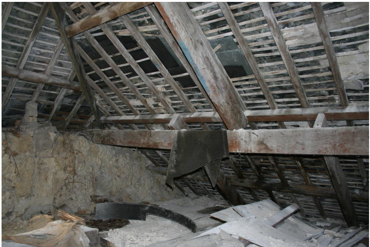
Fig 25 Detail of the roof over the south west corner of the loft of the western store, showing many laths missing or displaced, and potential for unstable timbers
