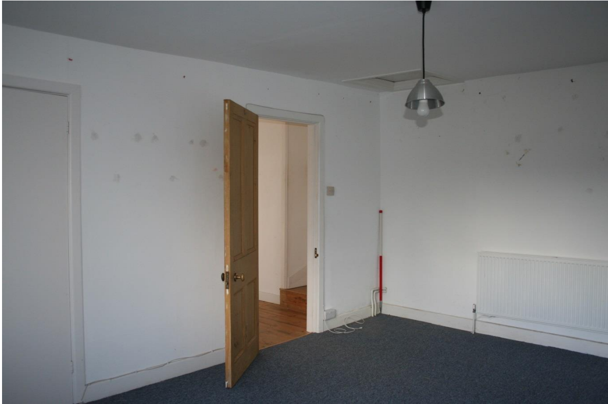
Fig 14 West chamber, with lined, thick south side likely to incorporate cob fabric of the early house front (right); the steps beyond mark the 19C link to the south wing
