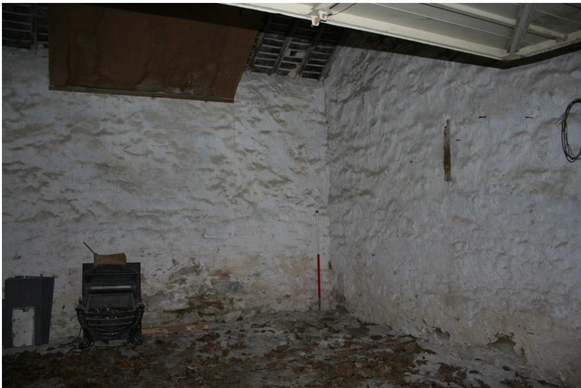
Fig 51 Rear, west side of Carriage House, showing plain whitewashed rubble stone walls, torched roof of scantle slate with some later boarding, and cobbled floor
