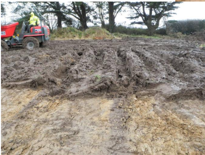
Fig 31 The very wet conditions causing deep wheel rutting in the top of the underlying natural.
