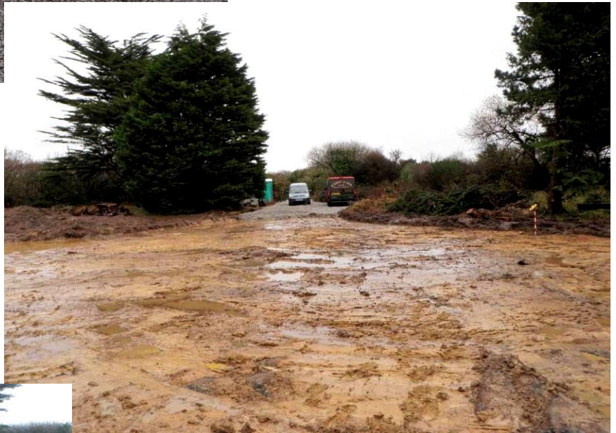
Fig 30 Topsoil stripped area of the new build looking east towards the road showing natural orange clay (19). The barrow is located on the right hand side behind the tree.
