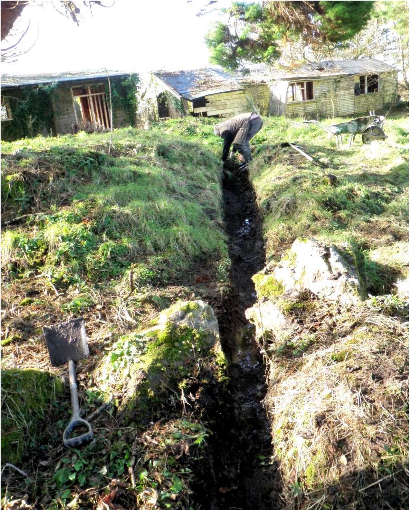
Fig 14 Looking west along the trench (during its excavation), showing two kerb stones – 12, spanning the trench in the foreground and the timber buildings after the removal of glazing (prior to their total dismantlement).
