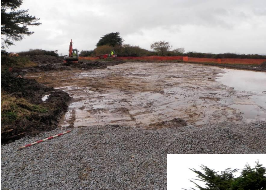
Fig 29 Looking west across topsoil stripping in the area of the new build. The barrow is to the left of the picture. Note occasional protrusions of grey green stone through natural orange clay (19).
