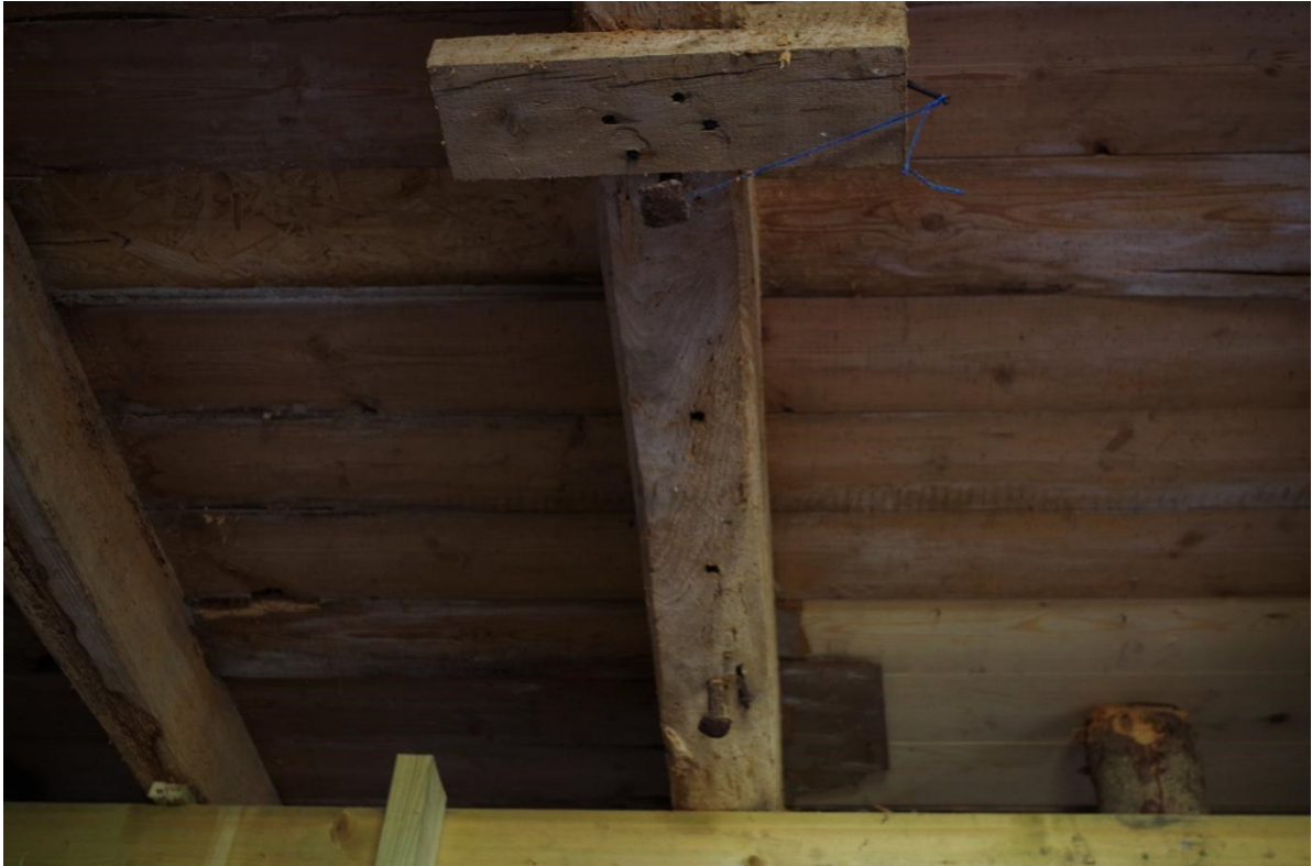
Fig 21 Iron bolts set in a joist in the north-west part of the ground floor, probably as supports for a phase 3 cider press
