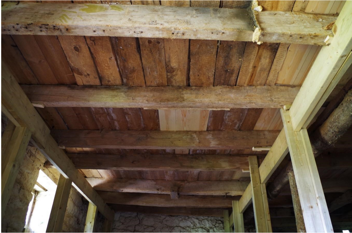
Fig 23 North-west part of the first floor structure viewed from the ground floor showing reused joist in foreground
