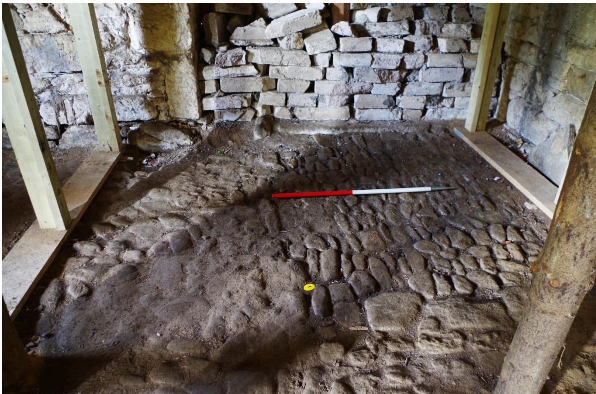
Fig 18 Interior ground floor showing cobble infill in north-east corner where cider press has been removed
