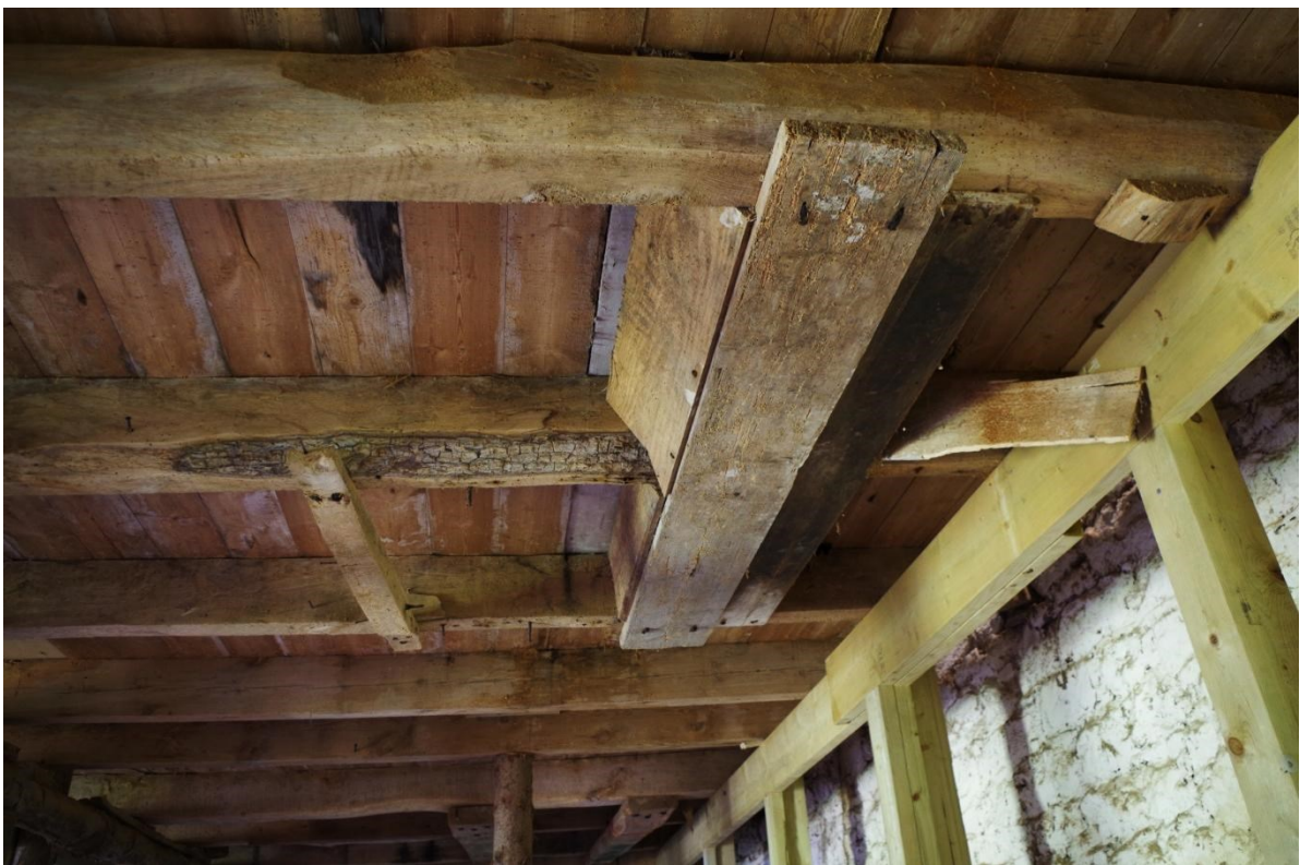
Fig 22 Remains of apple chute attached to joists along the east side of the ground floor
