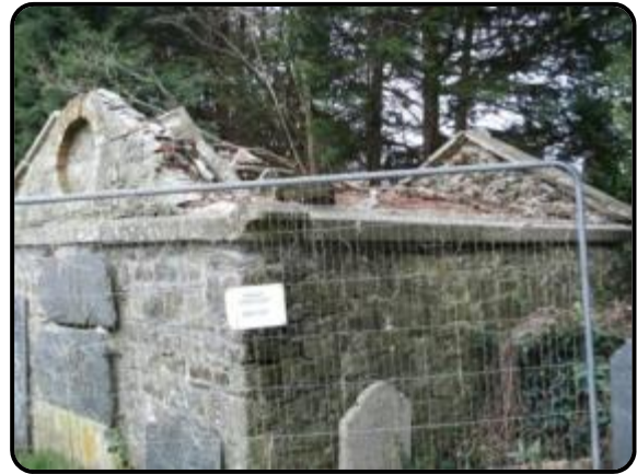
Figure 28 Collapsed roof of family funerary vault, St. Stephens, Saltash.
