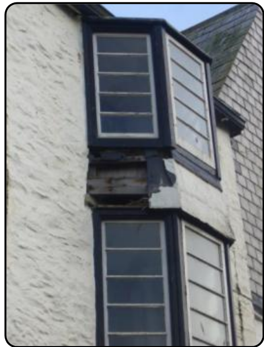
Figure 23 Damage to bay window (missing render-washed slate), with exposure of internal timber structure.
