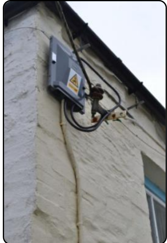
Figure 26 Wiring to building exterior with rusted bracket and insulator hanging free.
