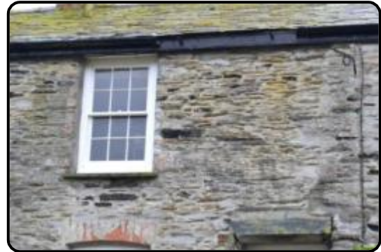
Figure 17 Missing section of gutter.
