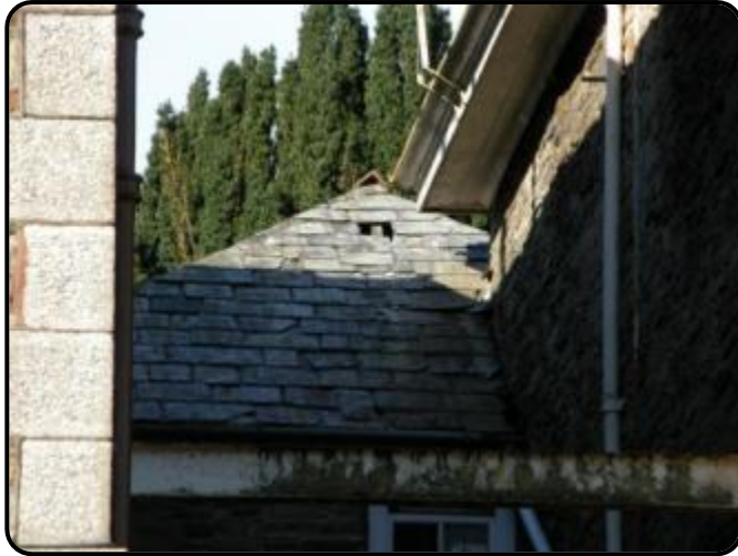
Figure 10 Missing slates, with roof open and rafters exposed.
