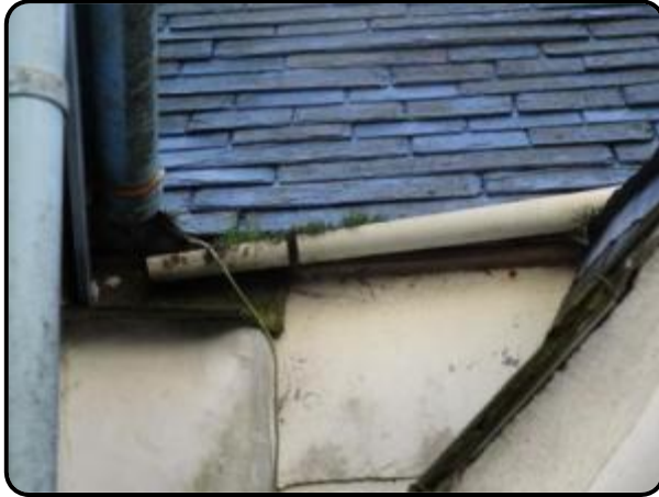
Figure 18 Accumulating vegetation appears to have resulted in disconnection of the gutter.
