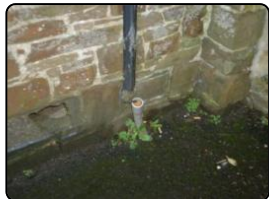
Figure 21 Inadequate downpipe and damage.
