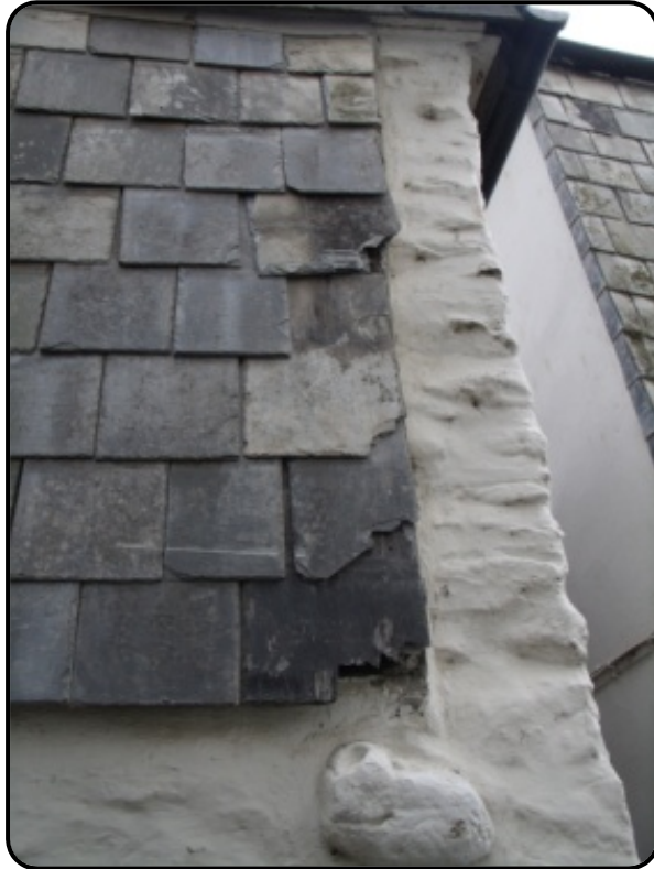
Figure 25 Damage to hung slate, reportedly caused by vehicular traffic.
