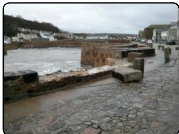
Figure 31 Damage to the historic harbour wall following the recent storms, Porthleven (Image: Peter Smith 2014)
