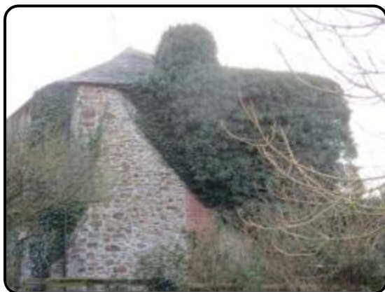
Figure 12 Rampant ivy, over-running walls and roof.
