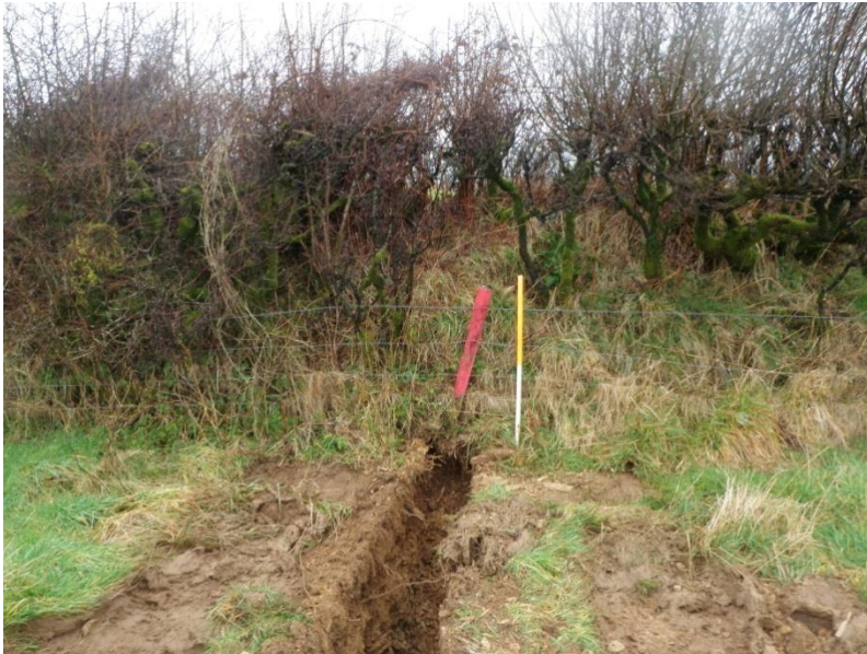
Fig 12 (Left) The low voltage cable trench, looking north towards the soon to be breached southern boundary of the turbine field.
