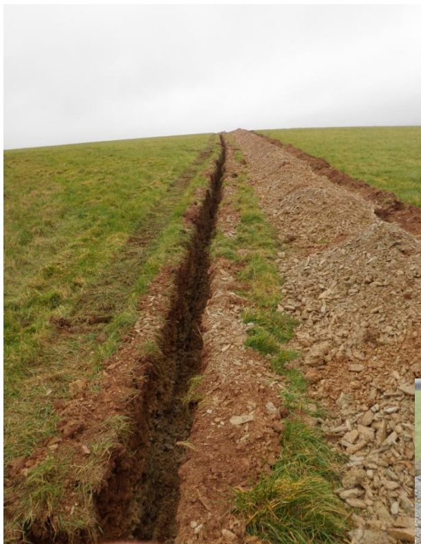
Fig 13 (Right) The low voltage cable trench as it curved around the cowsheds, showing redeposited context (5).
