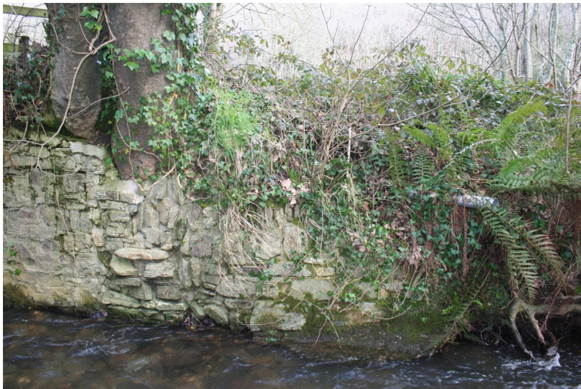
Fig 14 North abutment, upstream side showing evidence of earlier abutment walling beneath and to east of tree roots
