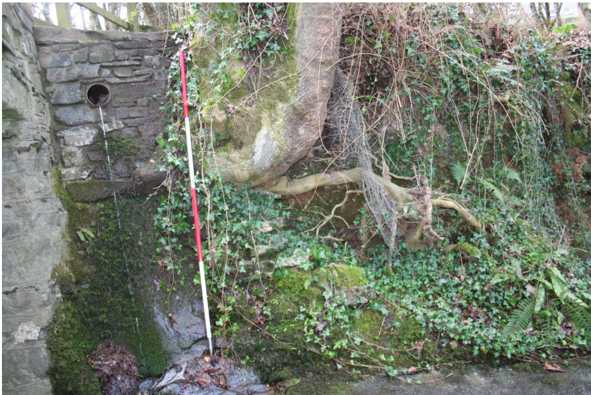
Fig 13 South abutment, downstream side showing evidence or earlier abutment walling beneath tree roots
