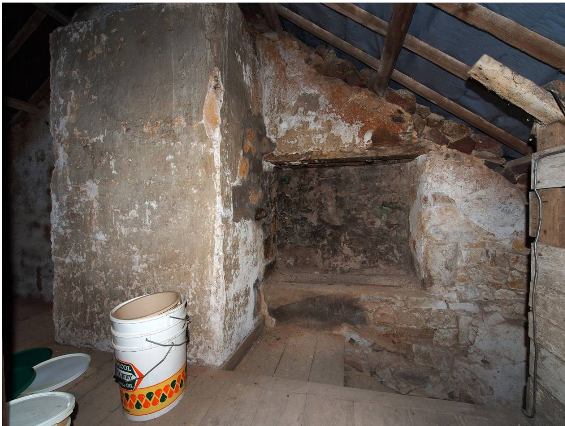
Fig 31 A window (subsequently blocked) originally lit the landing area of the attic stairs. There are also likely to have been small dormer windows in the rear roof slope.
