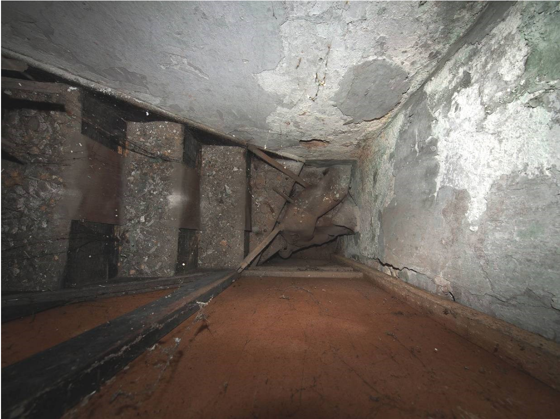
Fig 28 View downwards into blocked service stairway formerly connecting ground and first floors.
