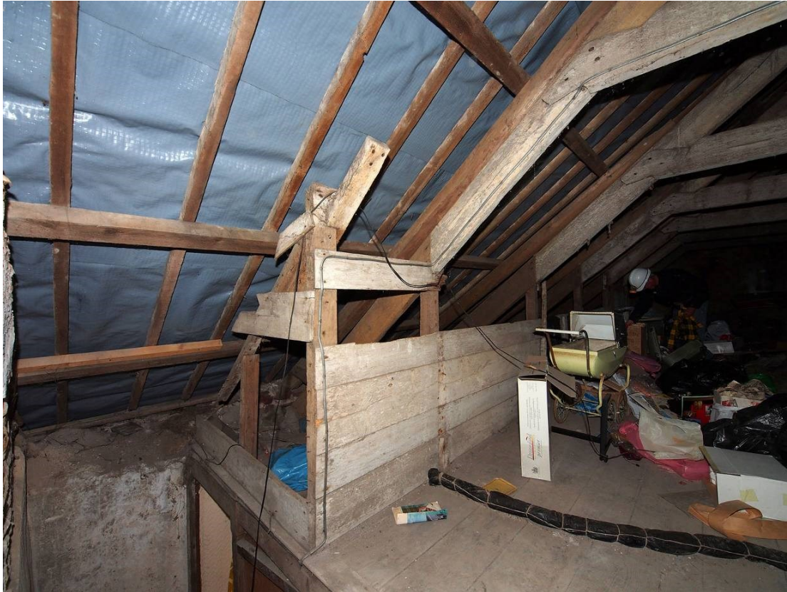
Fig 30 Attic level, showing horizontal boarding which once formed walls of service bedrooms.
