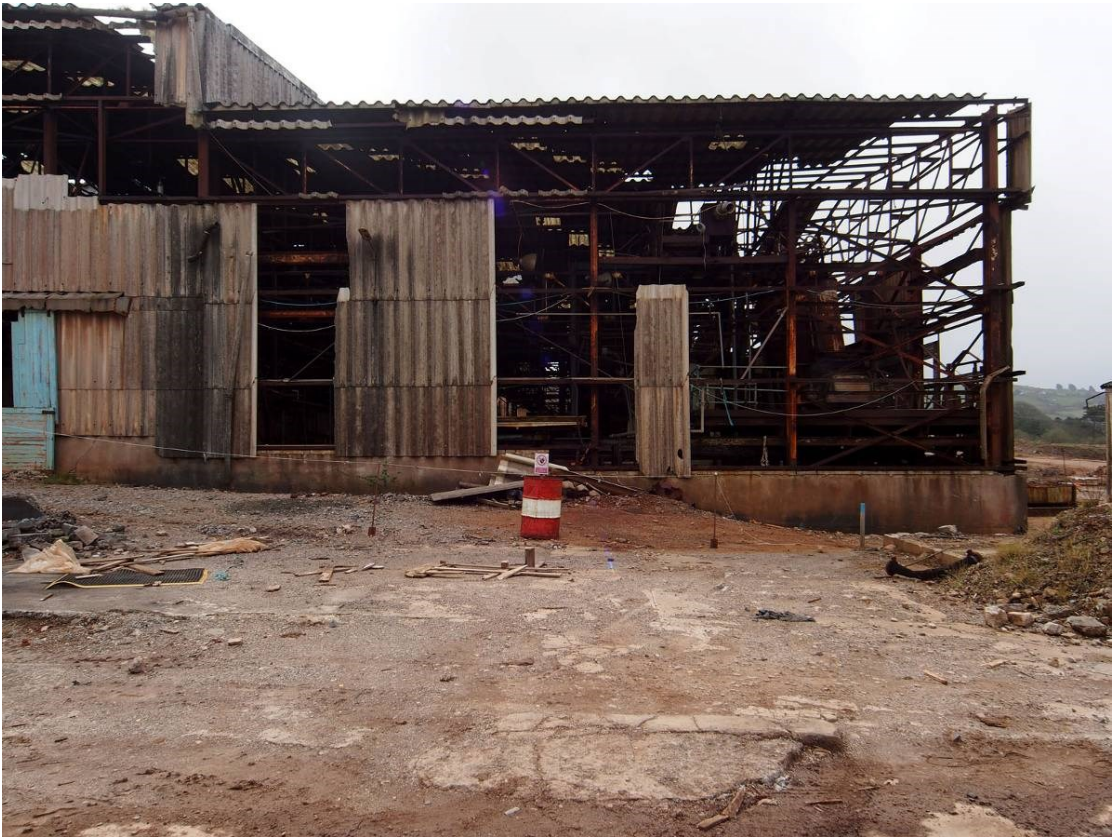
Fig 21. The north western corner of the mill, this building housing shaking tables and flotation cells, as well as other equipment.
