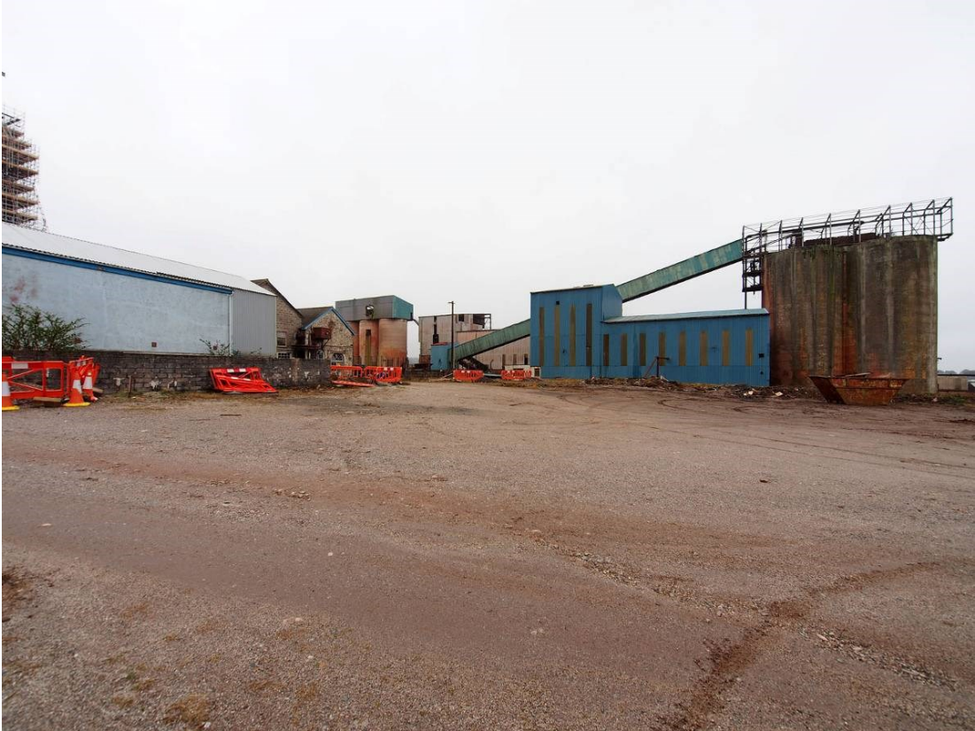
Fig 17. A general view of the mill from the east prior to its demolition.
