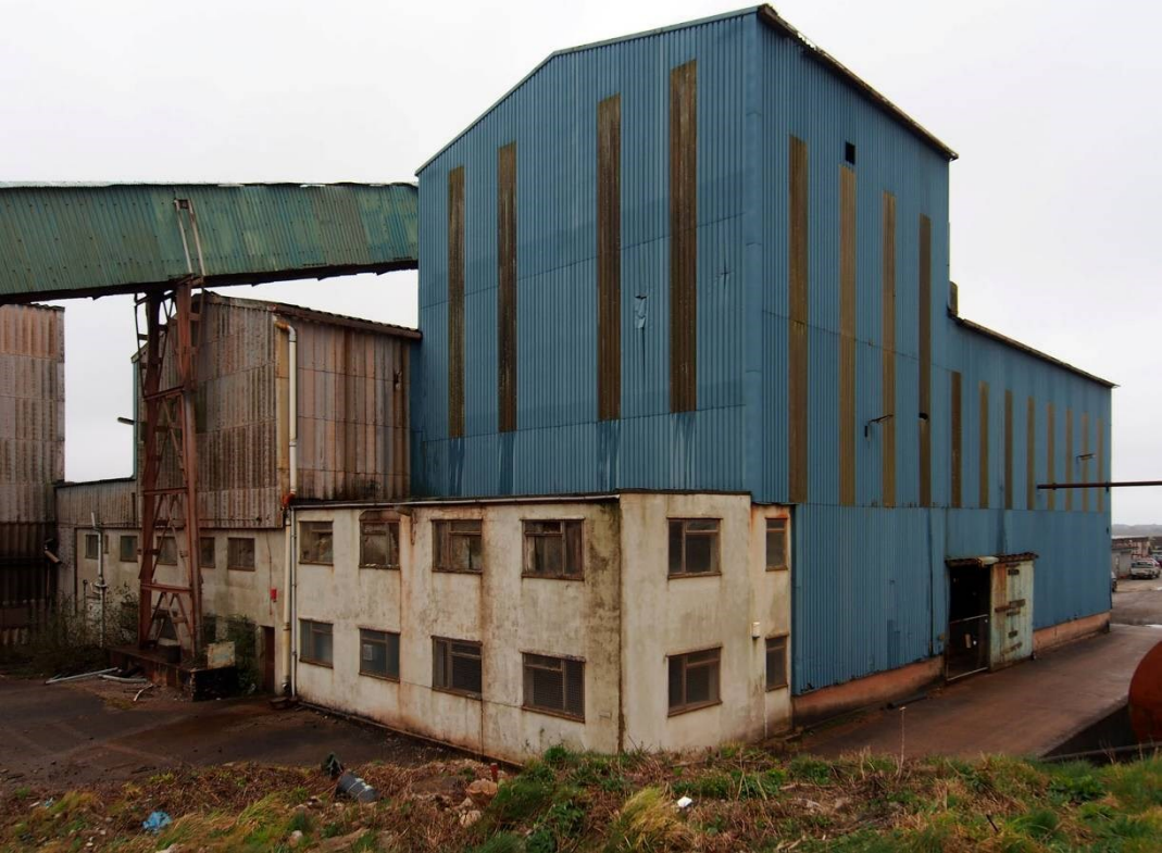
Fig 12. The tall building in the north eastern part of the South Crofty mill which housed banks of Humphrey spirals as well as other concentration plant.
