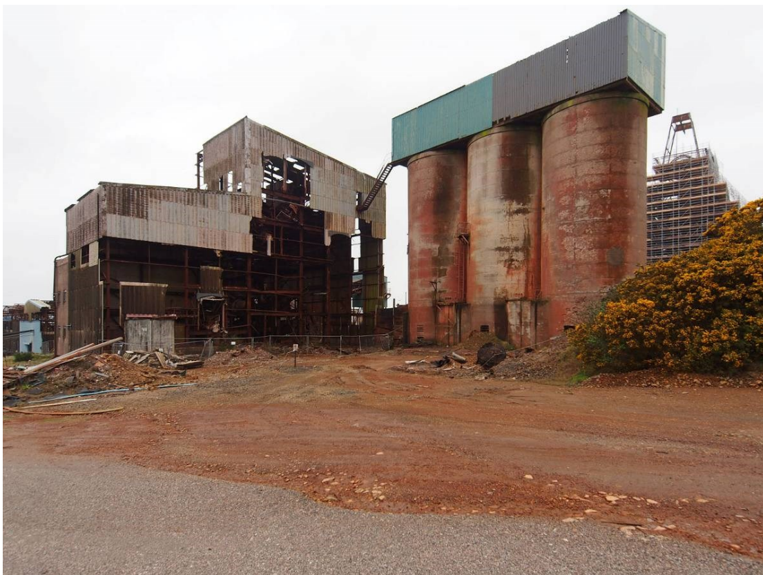
Fig 8. The primary ore bins (right) and primary crusher building (left), which had already lost considerable amounts of its cement asbestos sheet wall cladding.
