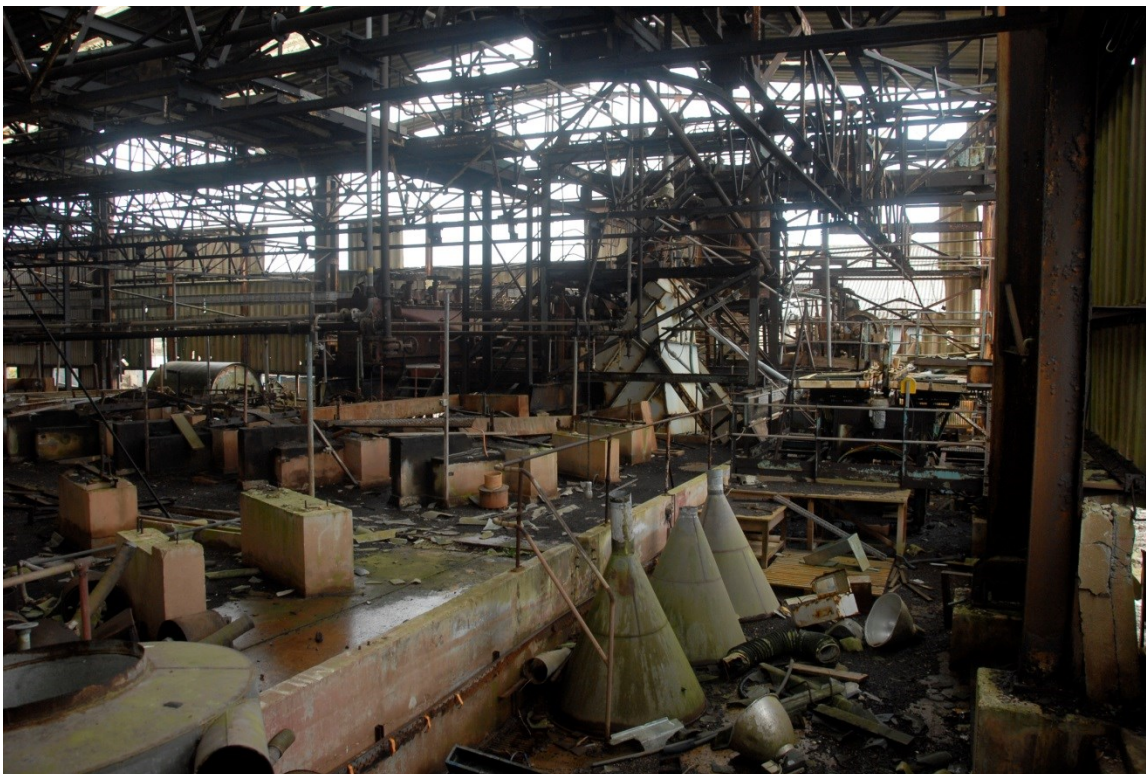
Fig 24. The interior of the northern end of the table plant. Most of the equipment had been stripped from this area of the mill, leaving only their concrete bases, though tables, ball mills and other equipment survived in the eastern section of the mill.
