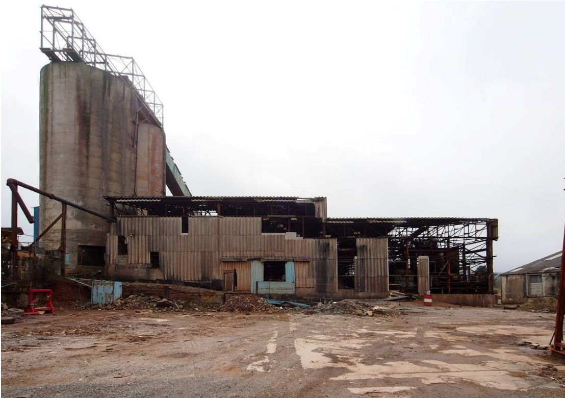
Fig 27. A view of the northern end of the mill from the north, showing the fine ore bins and ore conveyor (left) and the table plant (right).
