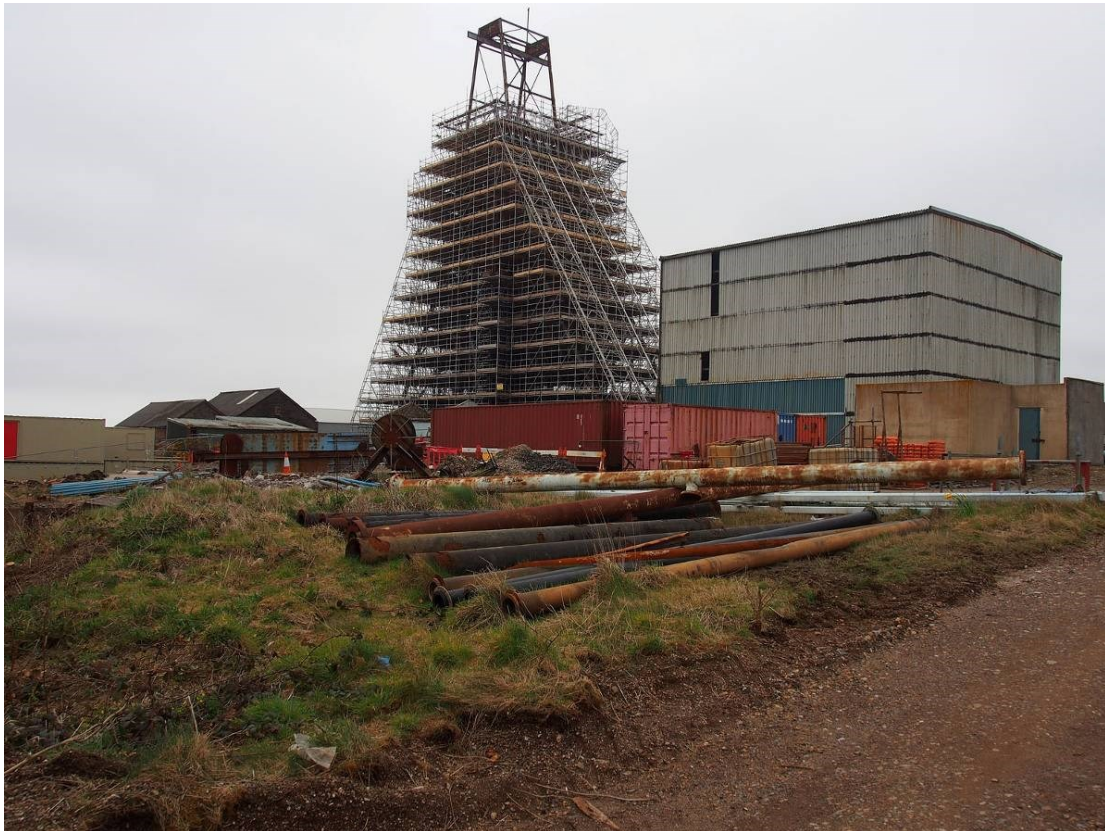
Fig 7. The headframe on New Cook's Shaft, scaffolded in preparation for conservation works and repainting in April 2013.
