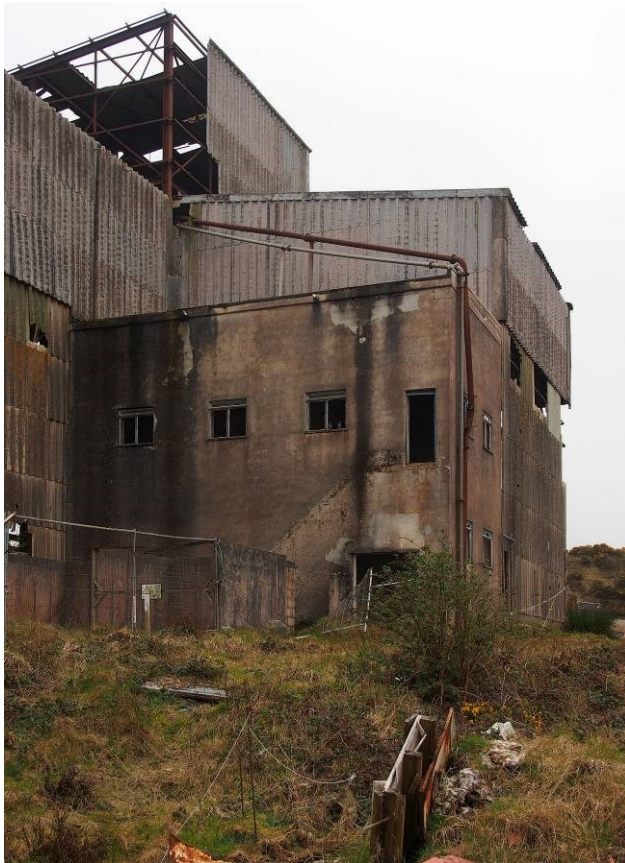
Fig 25. Part of the western elevation of the mill, showing its rendered blockwork construction and corrugated cement sheet cladding.
