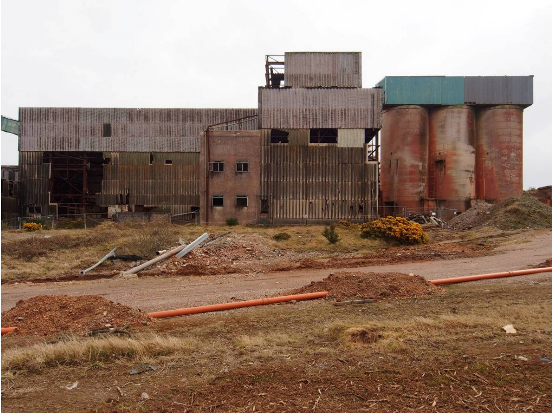
Fig 18. The primary crusher building and coarse ore bins viewed from the west.
