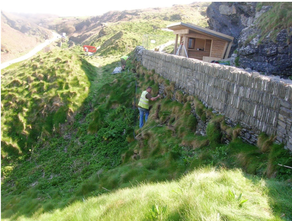
Figure 13. Route of service cable along exterior of barbican wall looking south, south-east.
