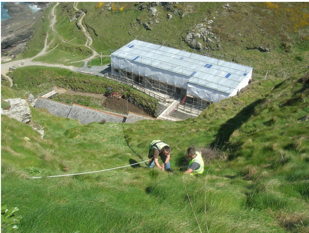
Figure 11. Course of cable trench from the Lower Ward ditch to the visitor centre in the valley below. View looking north-east.
