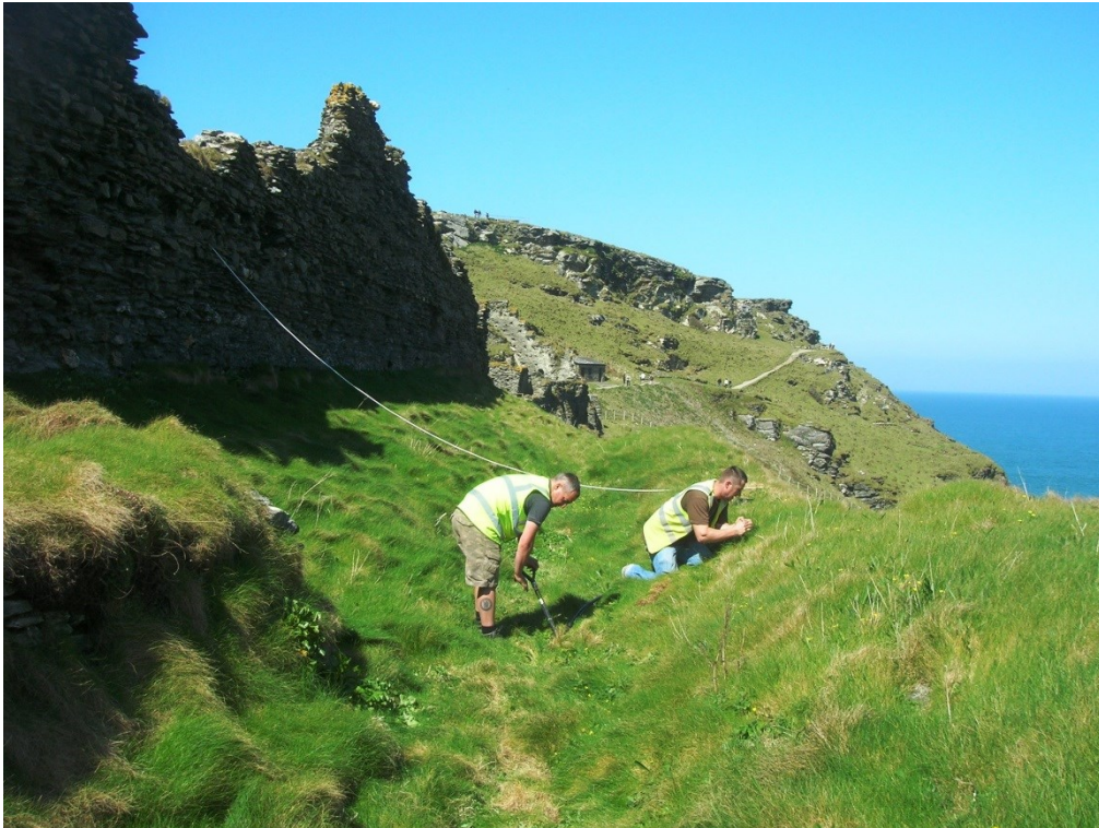
Figure 10. Cutting of service trench in ditch outside north-east curtain wall of Lower Ward.
