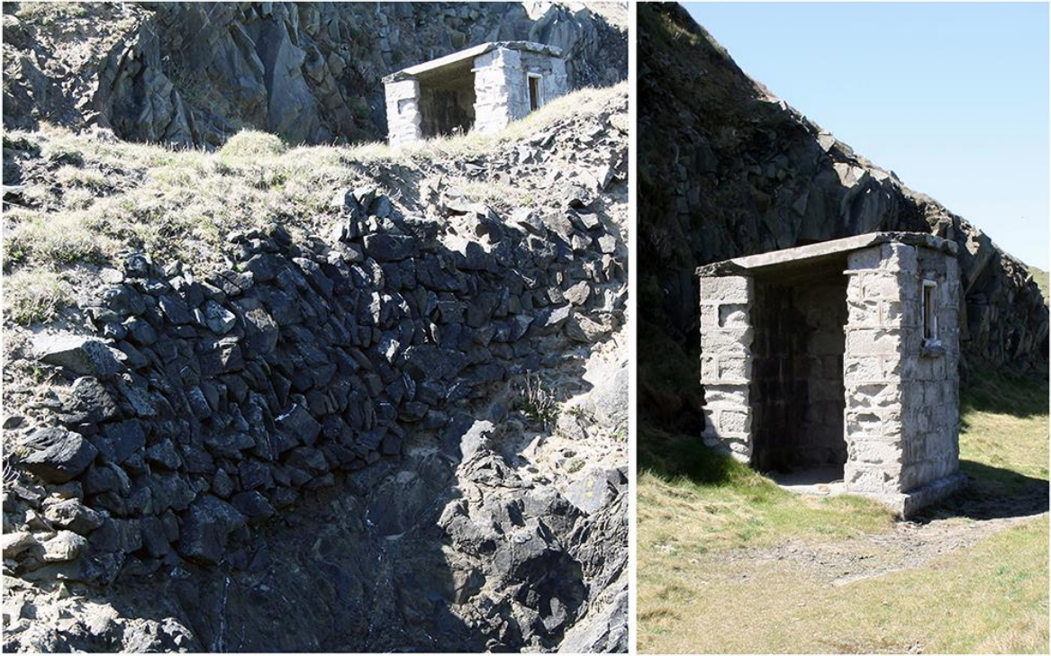
Fig 19 Retaining wall and small structure at the northern end of Stepper Point.
