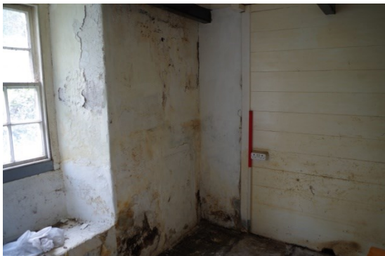
Fig 58 Interior study looking south-west showing inserted 19 th century planked wall abutting earlier partition
