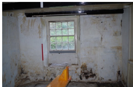
Fig 55 Interior study looking south showing truncated former front wall to left, blocked inserted fireplace to right and former door opening with inserted window
