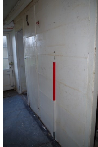
Fig 47 Interior 18 th or early 19 th century planked wall in hall looking east
