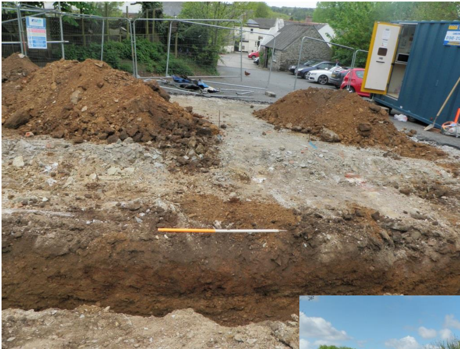
Fig 10 Looking south towards the Dolphin Inn, showing former track [9] in southern house foundation trench.
