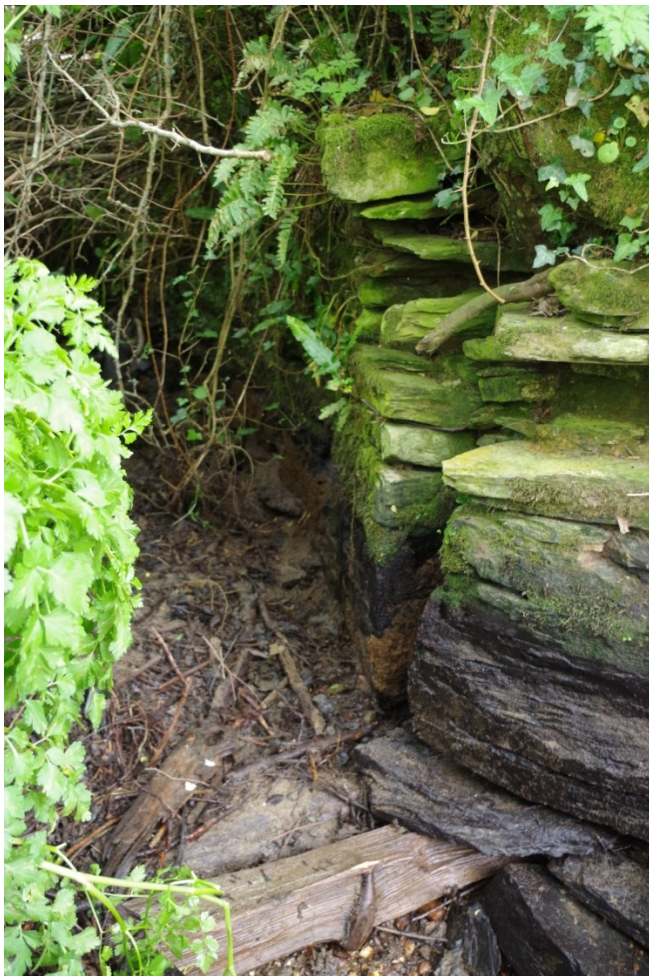
Fig 12 South wall of leat showing slot for sluice gate and timbers at base
