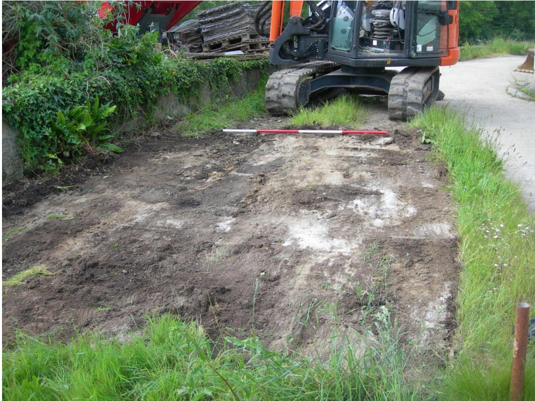
Fig 6 Works site stripped of turf with the concrete layer 2 exposed, from the north east The spread of concrete is probably associated with the laying of the roadway alongside.
