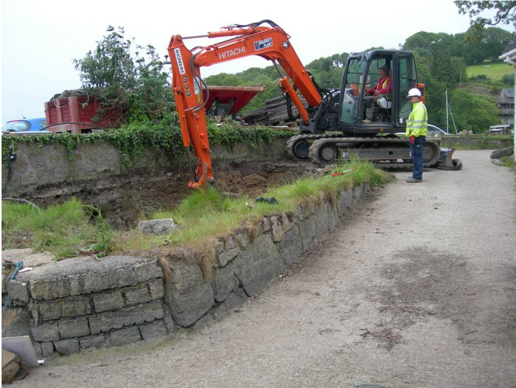
Fig 12 Revetment on the south east of the secondary road cut over the historic quay
