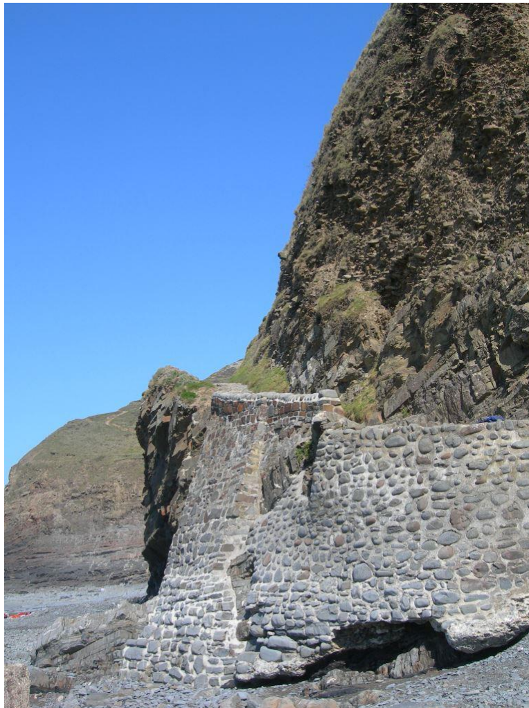
Fig 42 Vulnerable incline of sanding way to Welcombe Mouth near its end on the beach
