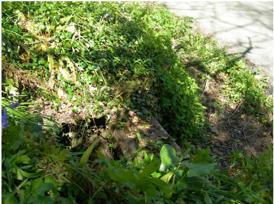
Fig 49 Well by the roadside near Watergap, with collapsed top (foreground, left)
