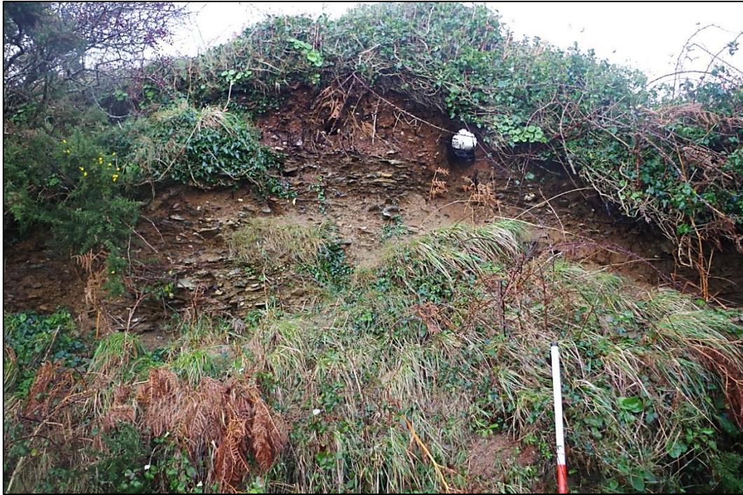
Fig 7 Severe erosion and animal burrowing on part of the southern rampart of The Bulwarks, looking southeast from one of the field lanes
