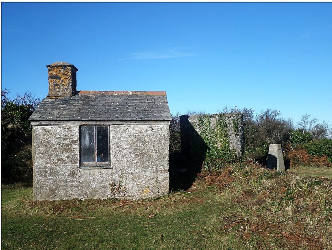
Fig 20 The watch house and lookout platform, looking northwest from inside the enclosure. Climbing ivy threatens the lookout tower and the walls of the watch house and the built structure shows signs of disrepair
