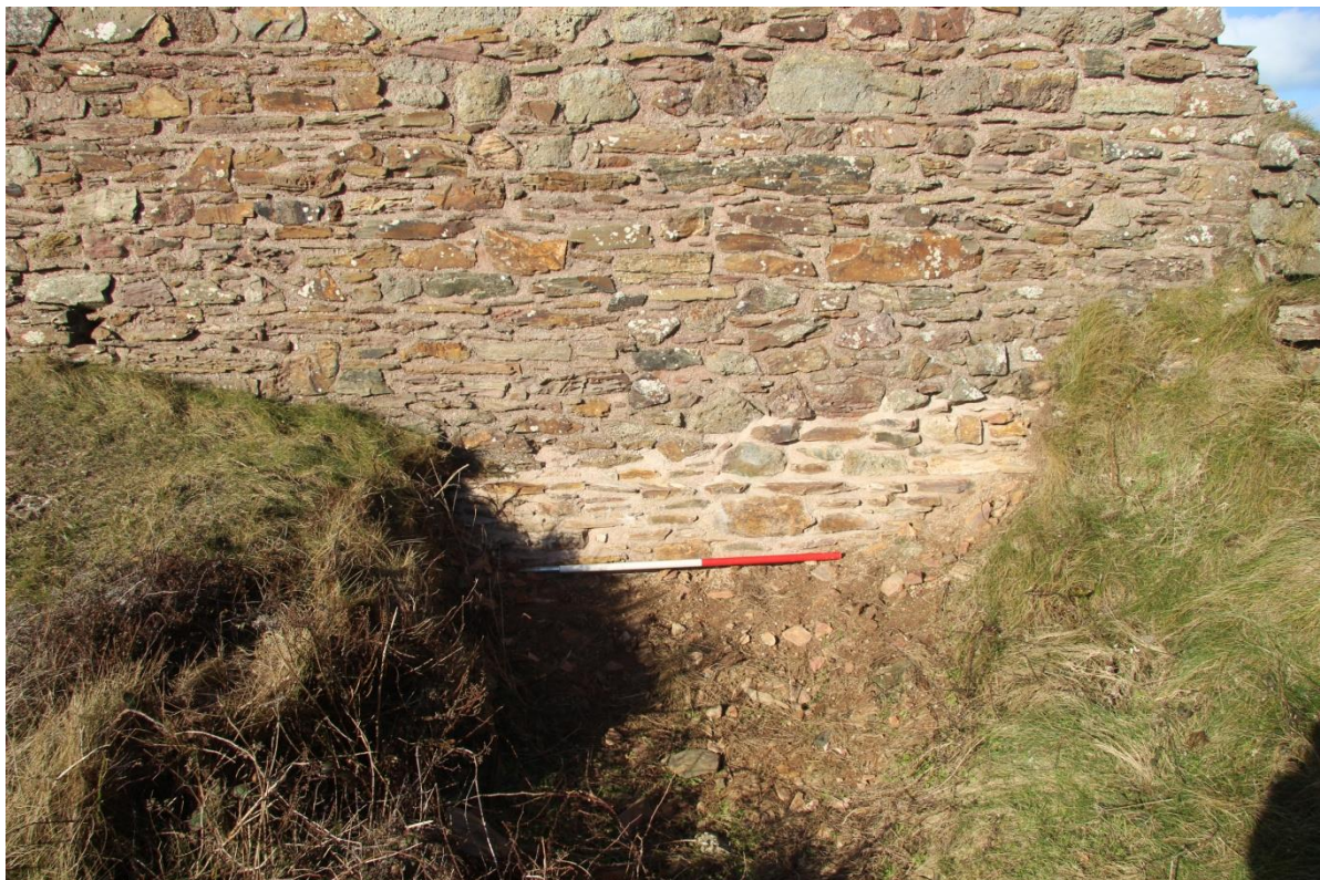
Fig 19. The repairs undertaken to the lower section of the walling of the horizontal whim engine house.
