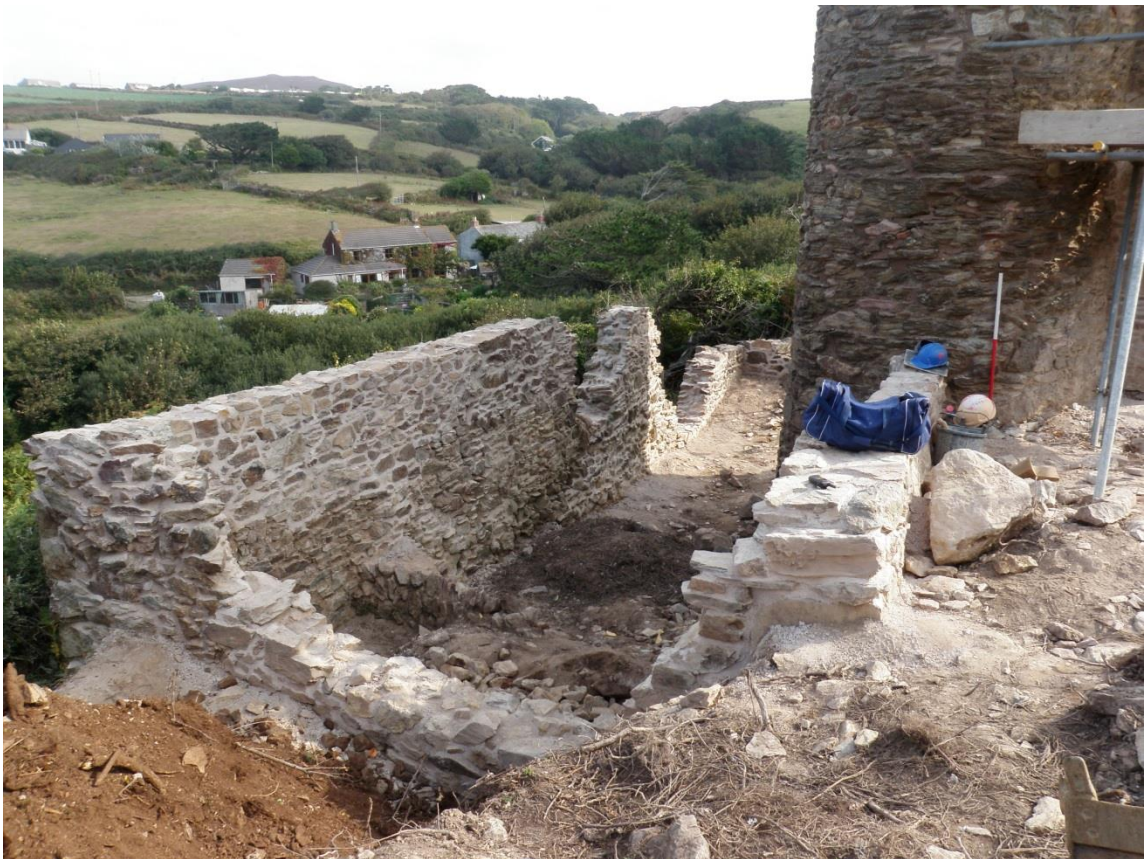
Fig 55. Conservation works in progress within the Charlotte United boiler house, which was fully re-pointed given its condition.
