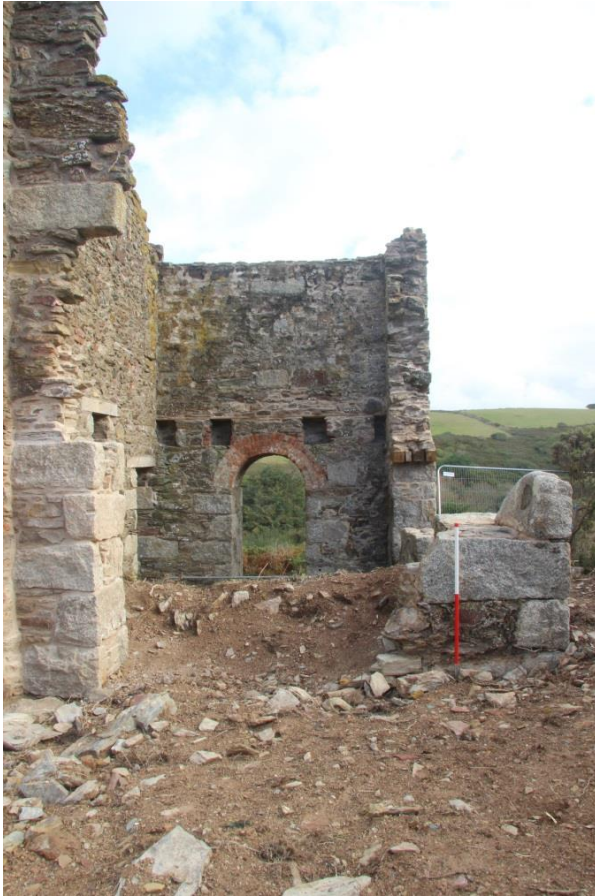
Fig 58. The remains of the pumping engine house at Charlotte United during its consolidation. The quoined reveal which formed the left surviving side of the cylinder opening was partially reconstructed to strengthen the building.
