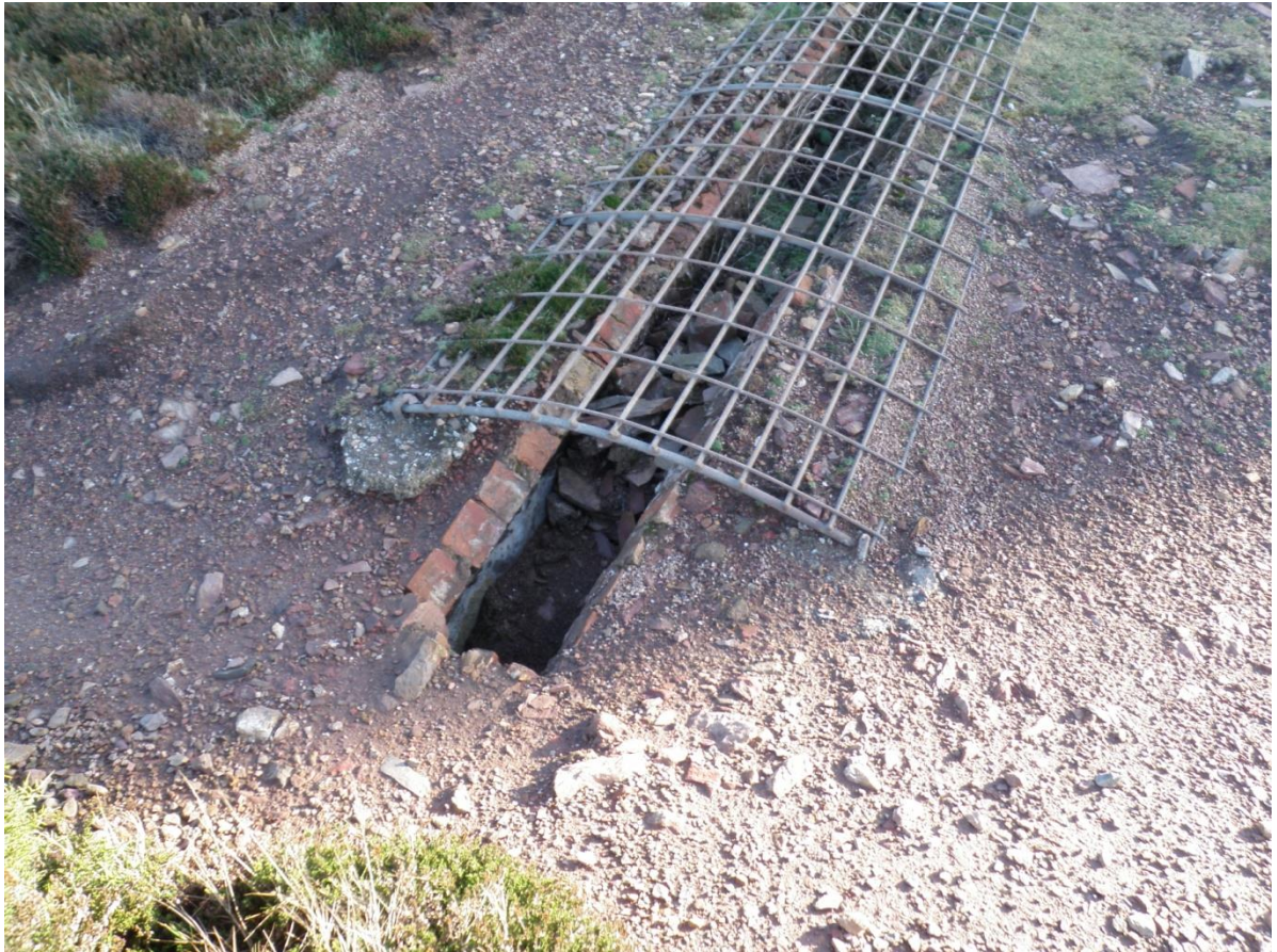
Fig 28. The lost brickwork from the head of the arched calciner flue where it runs just below the ground surface.
