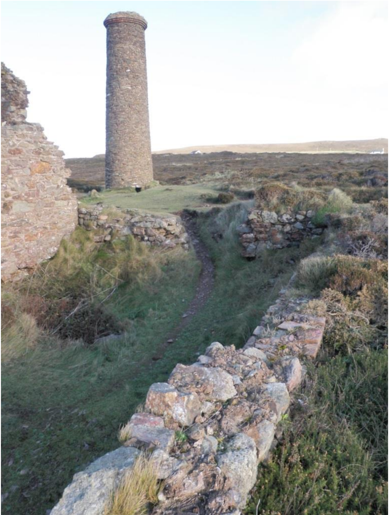
Fig 17. The eastern end of the boiler house associated with the all-indoor beam whim engine house, showing the lost masonry over the flue connection to the chimney and the poor state of the wall heads.
