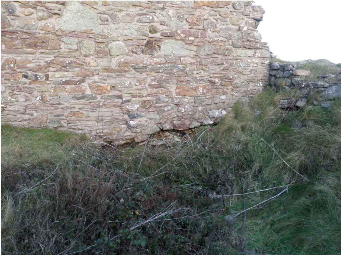
Fig 18. The eastern end of the southern elevation of the horizontal whim engine house, showing stone loss at its base.
