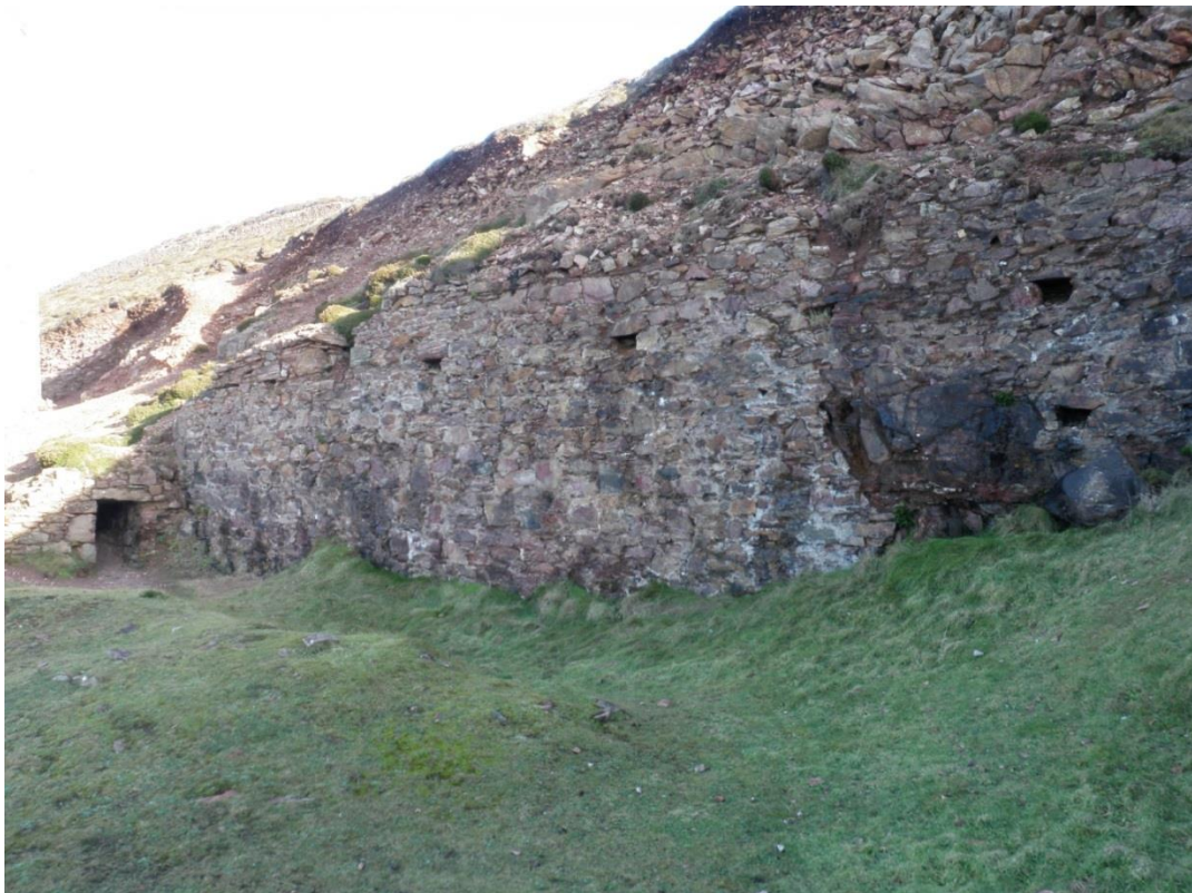
Fig 39. The remaining walling of the boiler house adjacent to the pumping engine house at Towanroath Shaft, showing the flue connection in its north eastern corner.
