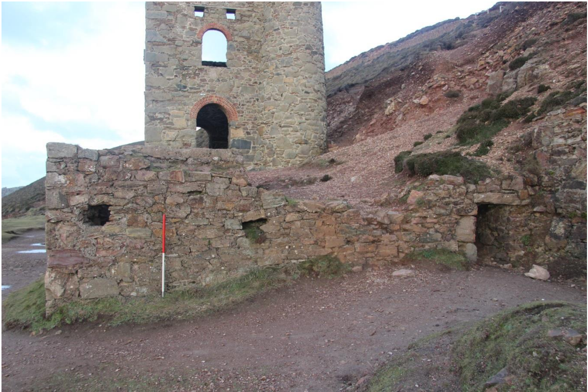
Fig 40. The southern end of the 20 th century horizontal engine house at Towanroath Shaft, with the flue entry from the boiler house to the right.
