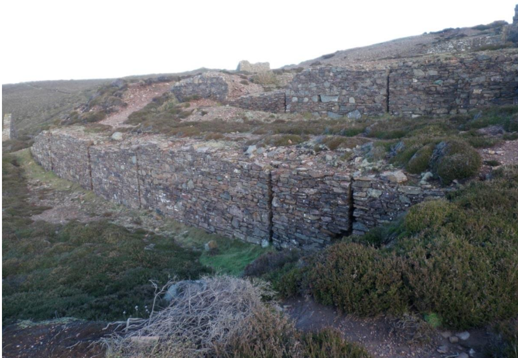
Fig 43. The walling of the Wheal Coates stamps and buddle floors to the north west of the stamps engine house.
