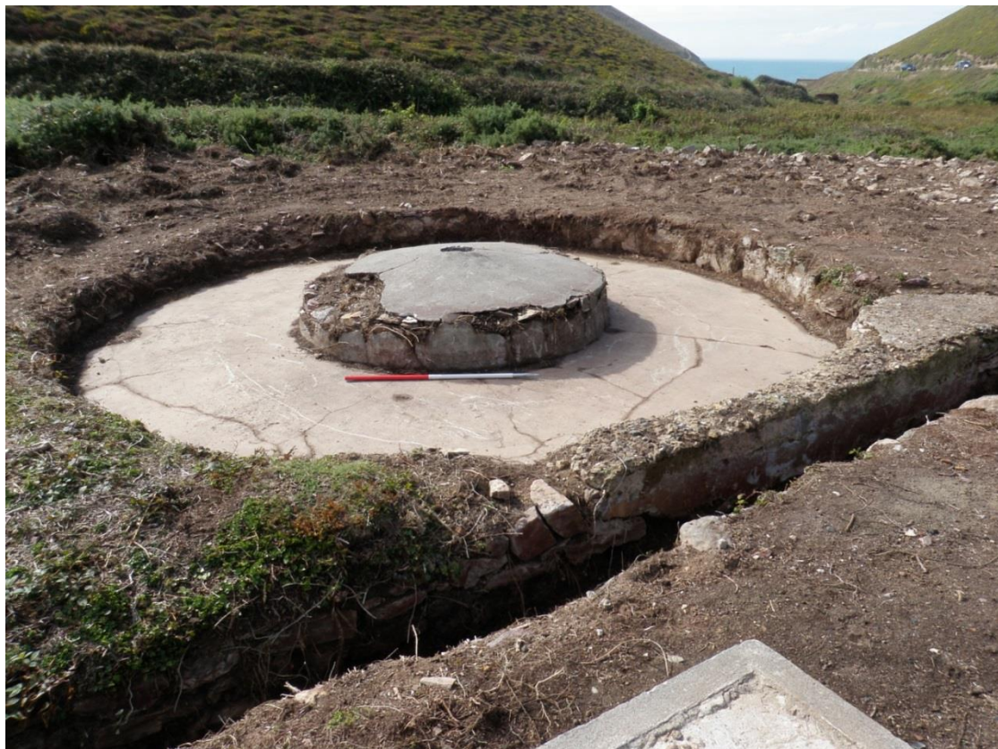
Fig 51. The convex buddle at the Old Century Works following the final removal of vegetation and rubble but prior to its consolidation.
