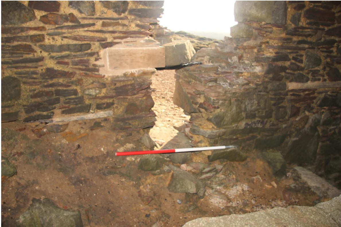
Fig 26. The replacement stub lintel inserted over the ground floor opening in the southern wall of the stamps engine house.
