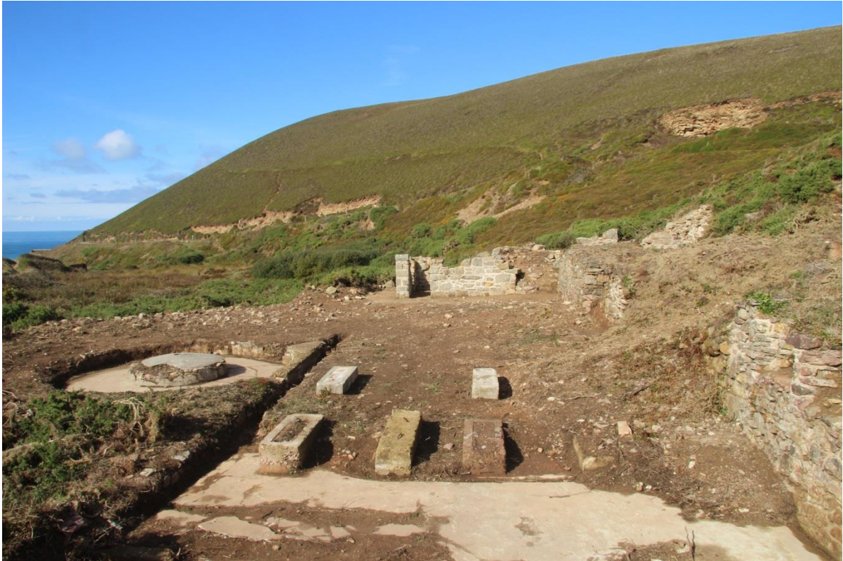
Fig 52. Looking north-west across the Old Century Works following extensive vegetation and rubble clearance.
