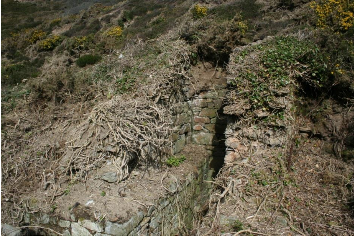
Fig 46. The Old Century Works stamps wheelpit prior to vegetation clearance and stabilisation.
