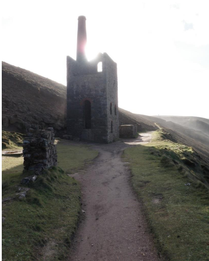
Fig 41. Towanroath Shaft engine house from the north, showing the low walling of the former change house in the foreground.
