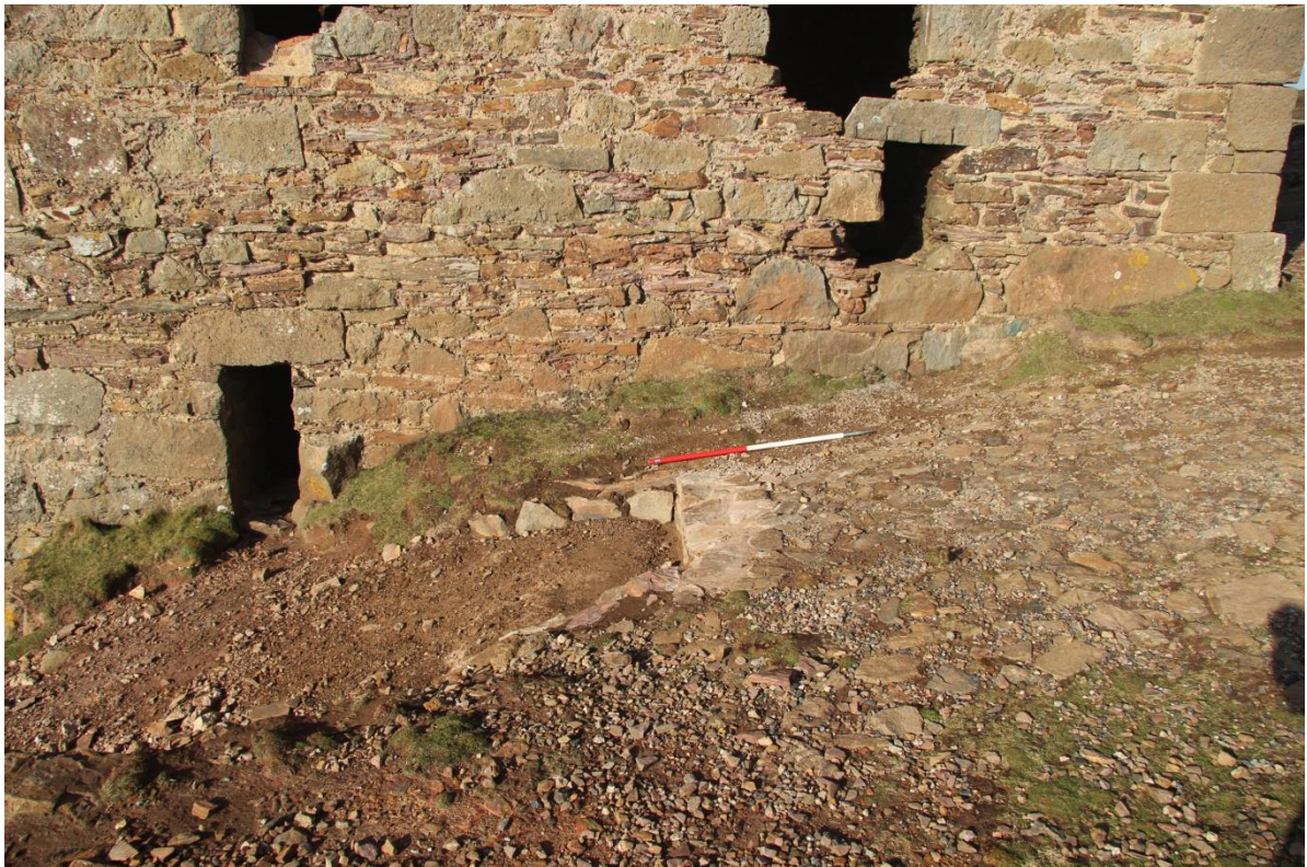
Fig 23. The repairs undertaken to the stamps tramway to stabilise it and prevent further foot erosion.
