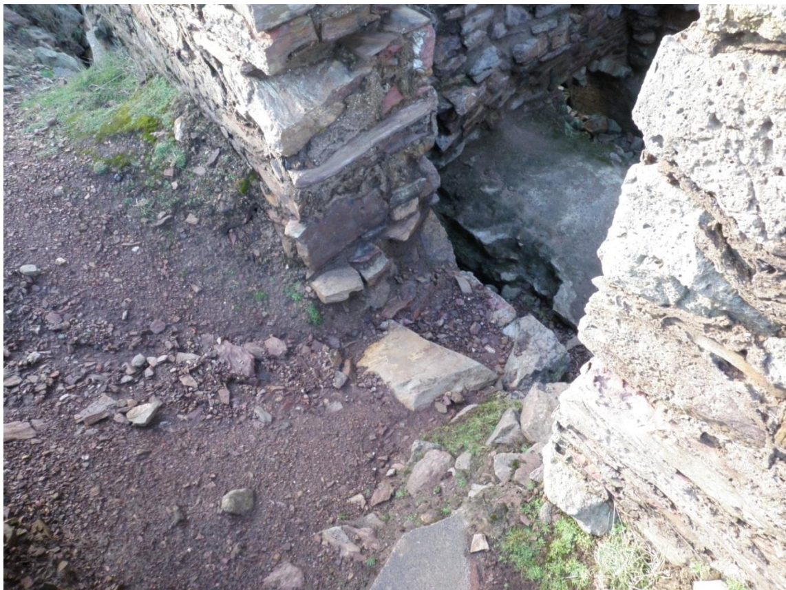
Fig 27. The eroded masonry forming the cill to the doorway in the eastern elevation of the reverberatory calciner.
