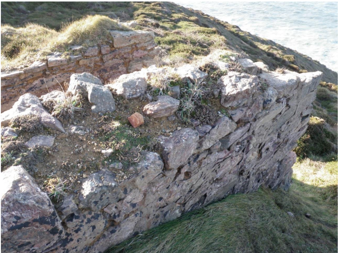
Fig 31. The poor quality of the wheelpit walling prior to works.
