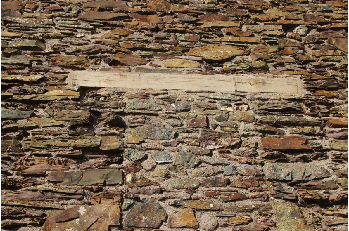
Fig 15. The replacement lintel over the blocked window in the southern elevation of the all-indoor beam whim engine house.
