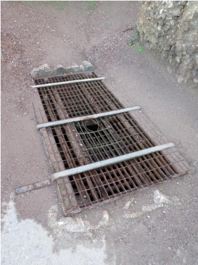
Fig 36. Towanroath Shaft, showing the steel barred grille inserted into the original concrete cap, the Lionweld grille set over it and the steel grille placed over that again. All had been damaged by visitors wishing to drop stones down the shaft.
