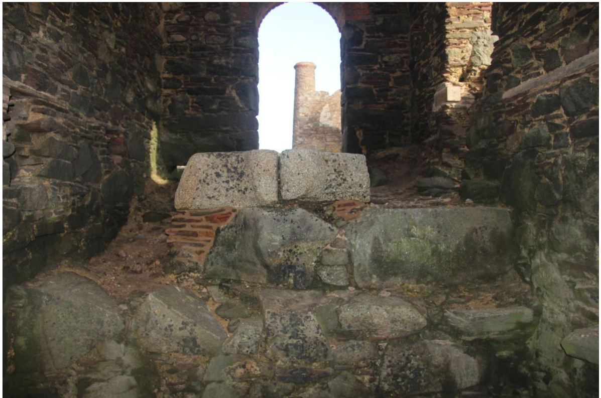
Fig 25. The underpinning masonry inserted beneath the western end of the cylinder bedstones in the stamps engine house.
