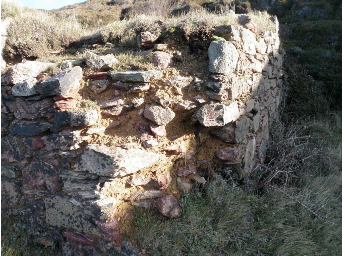
Fig 32. Lost masonry on the south western corner of the stamps gearing platform.
