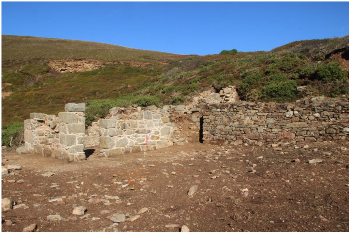
Fig 53. A general view of the structures at the western end of the Old Century Works following vegetation clearance and masonry conservation works.
