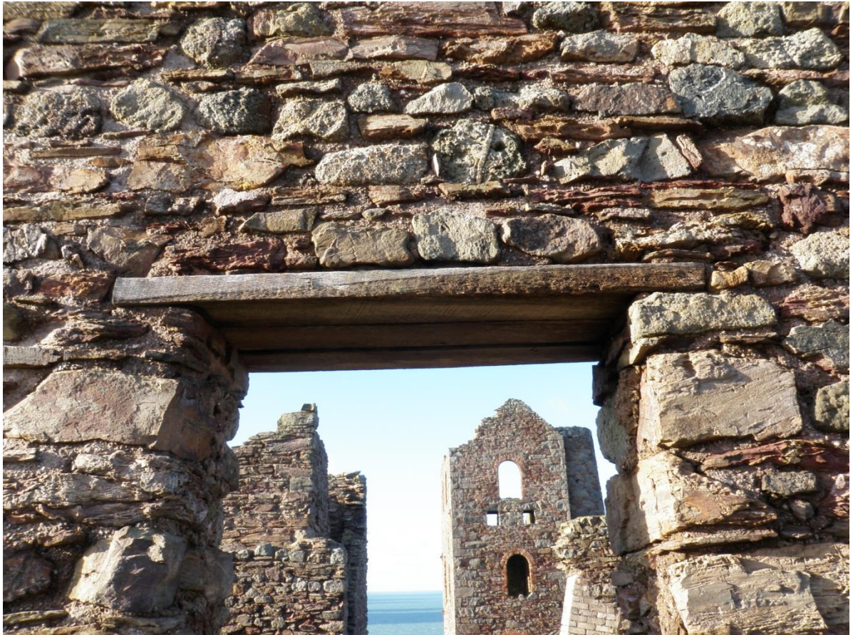
Fig 13. The lintel over the doorway in the eastern elevation of the horizontal whim engine house.
