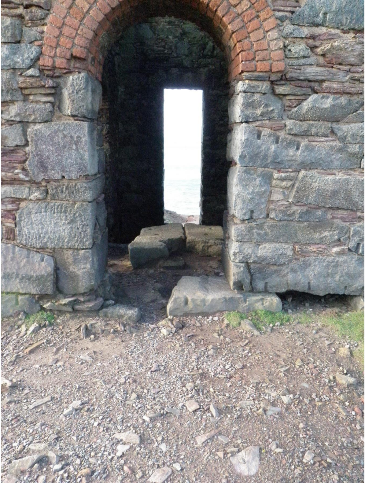
Fig 20. The cylinder opening in the eastern elevation of the stamps engine house, showing the low level flue connection to the boiler house which formerly abutted this side of the building.
