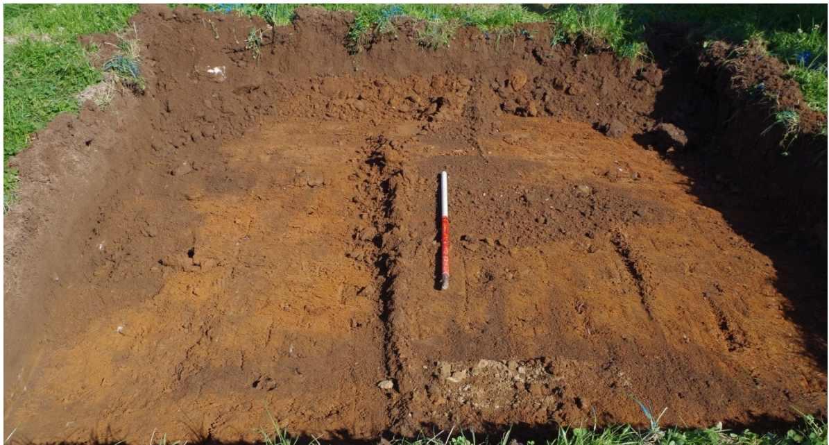
Figure 15. Excavation in Field 4 for the foundations of the substation showing the appearance of the topsoil (1) and subsoil (2) found across the site.
