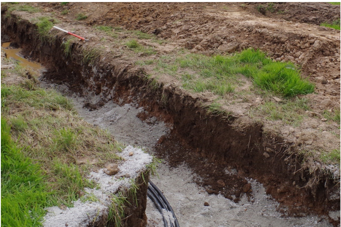
Figure 17. Probable parallel ditches [23], right opposite the black cables, and [25], left under the scale bar, at the northern extent of the cable trenching in Field 2.
