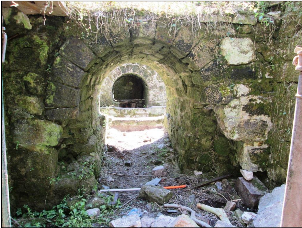
Figure 30 View of the Trevear power arch transmission tunnel before works (looking south) © CAU, CC 23/7/2014.
