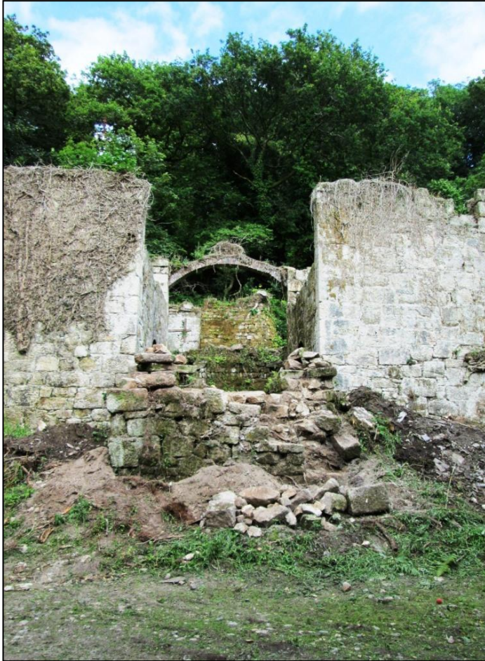
Figure 28 View of the west side of the Trevear wheelpit before works © CAU, CC 15/7/2014.
