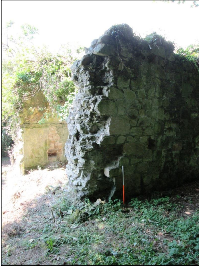
Figure 44 View of Trevear cottage south external elevation (from the south east) before works © CAU, CC 30/7/2014.
