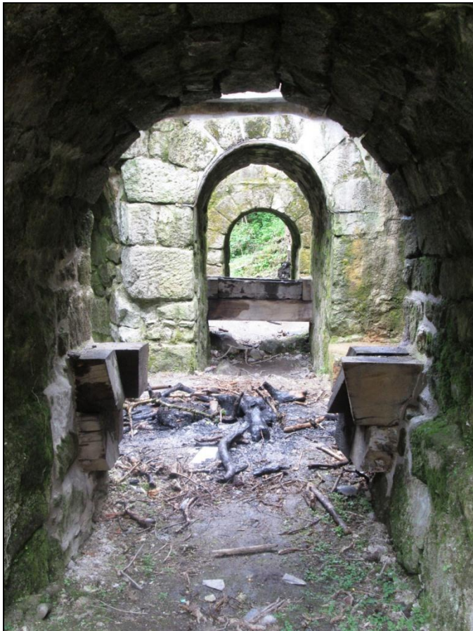
Figure 31 View of the Trevear power arch transmission tunnel after works (looking north) © CAU, CC 14/5/2015.
