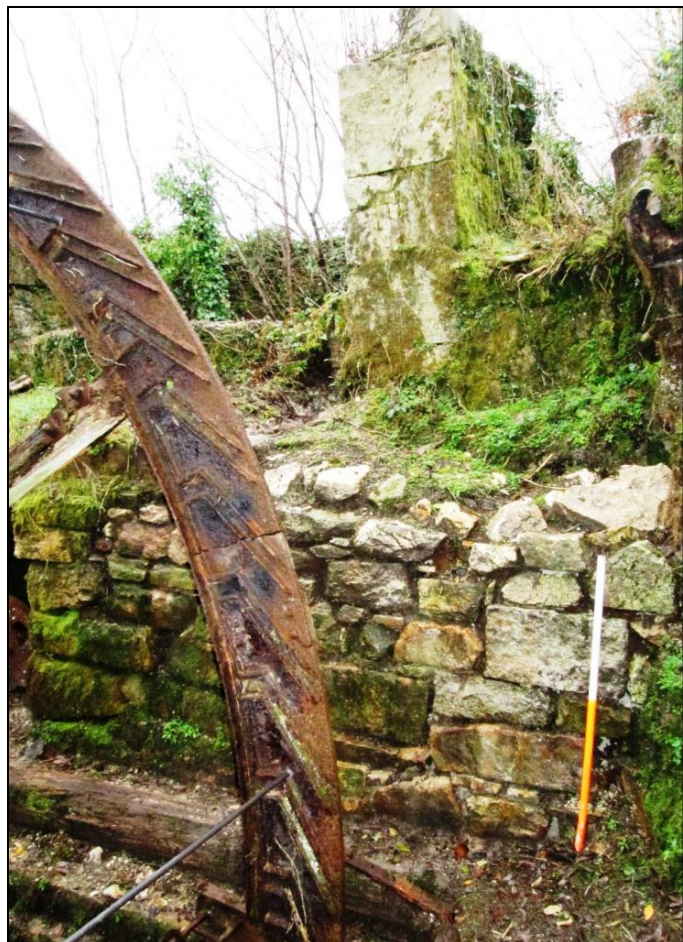
Figure 9 Similar view of the Wheal Arthur water wheel and south wall after repair works © CAU, CC 16/12/2014.
