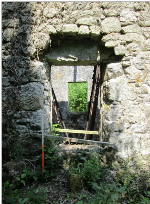
Figure 17 View of the upper northern mill window collapsed lintel before works © CAU, CC 23/7/2014.
