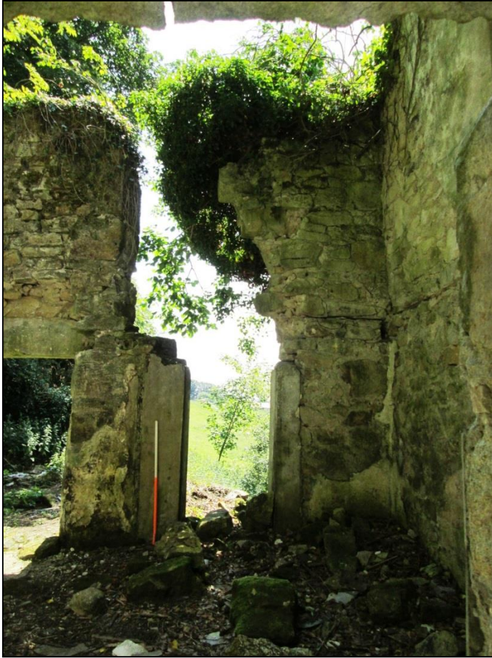
Figure 46 View of Trevear cottage inner south internal elevation (from the north) before works © CAU, CC 30/7/2014.
