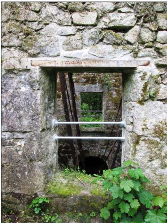
Figure 18 View of the upper southern mill window replaced lintel after works © CAU, CC 14/5/2015.
