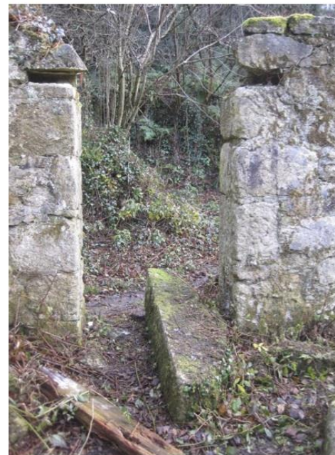
Internal view of opening - note remaining pockets for timber lintel and granite lintel on ground
