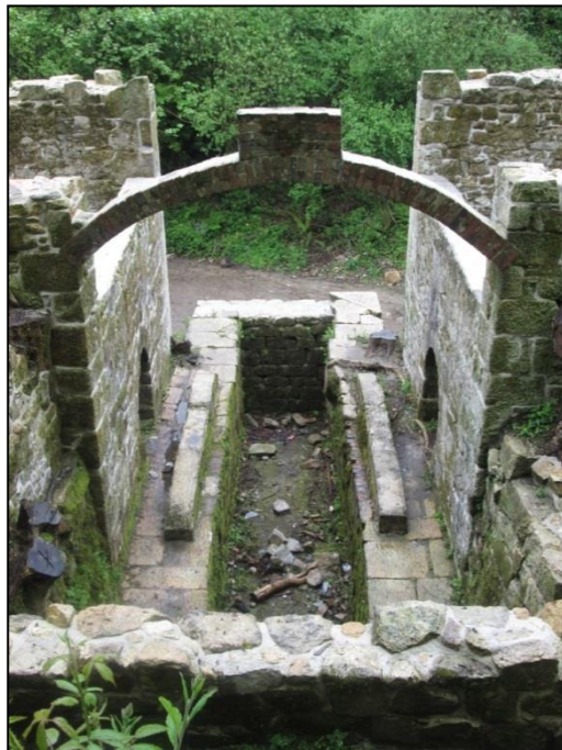
Figure 35 View of Trevear mill wheelpit (from the east) after works © CAU, CC 14/5/2015.
