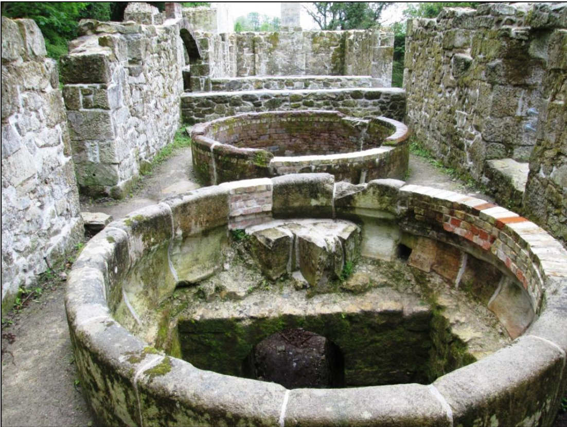
Figure 33 View of the first floor grinding pans and walls after works (looking south) © CAU, CC 14/5/2015.
