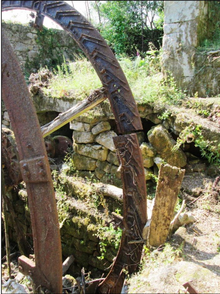
Figure 8 View (from the north) of Wheal Arthur water wheel rim break and south wall collapse before works © CAU, CC 23/7/2014.
