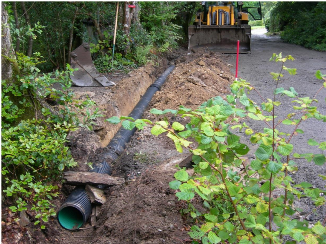
Fig 37 Lay-by with trench for pipe taking north east drain across opening from lane
