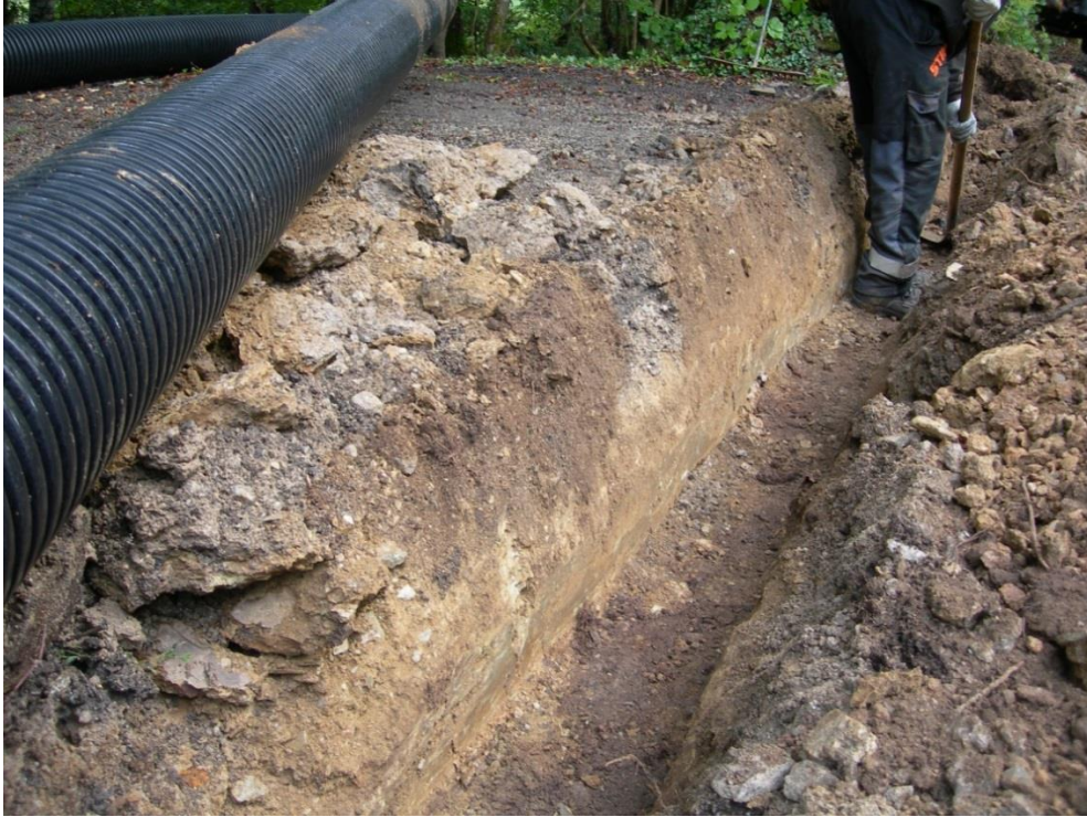
Fig 43 Trench for piping north east drain through lay-by, showing the lay-by's rab fabric
