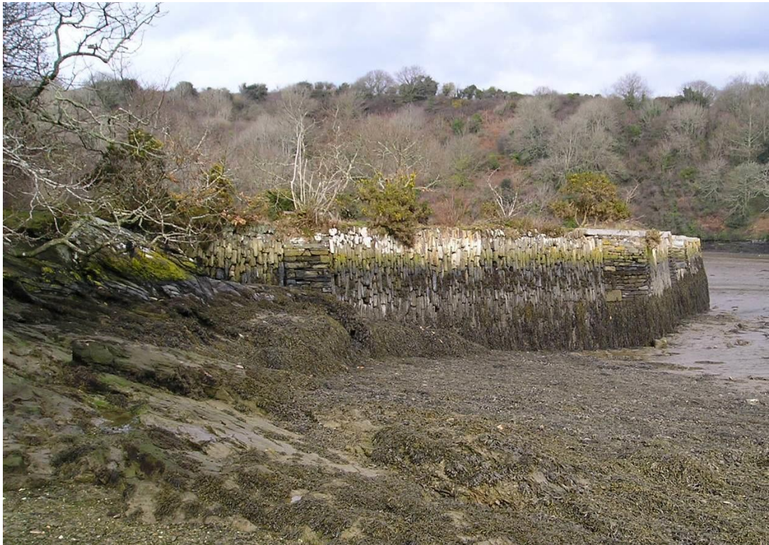
Fig 48 Roundwood Quay at the east end of the lane, from Lamouth Creek on its south The present quay is an early 19 th century rebuild and expansion of the smaller quay of the smelting works, recorded in 1786, itself built on an ancient landing place served by the ridgeway (Photograph by Graeme Kirkham for CAU).
