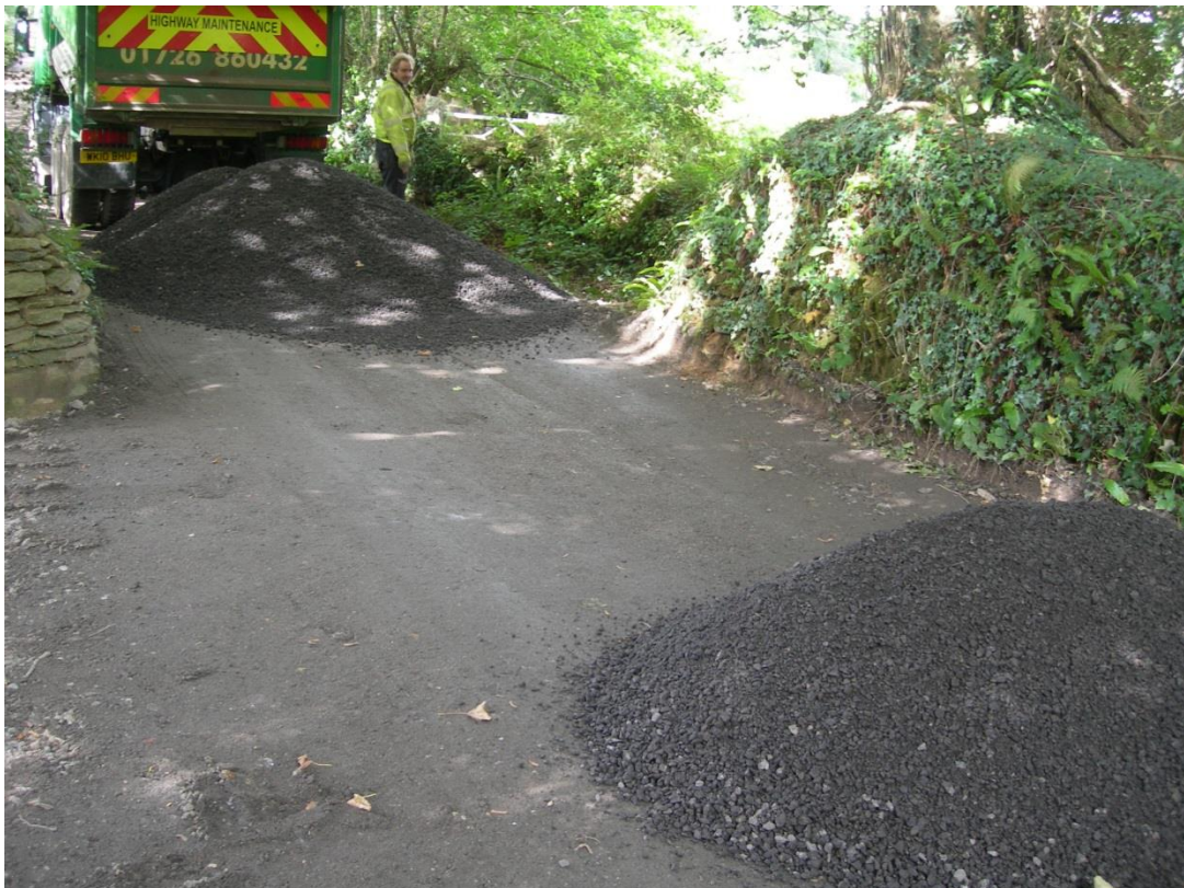
Fig 27 Tarmac planings for finishing the road surface, beside the outer cross-rampart. The rampart can be seen in section on the right between the two piles of planings.
