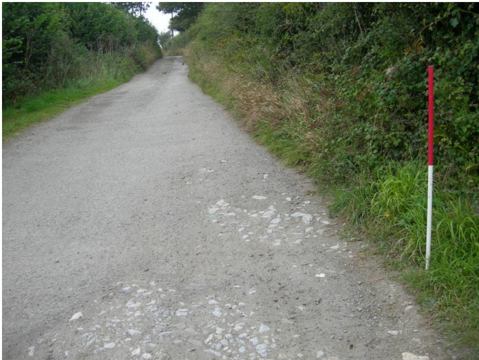
Fig 6 Centre of the lane, with limestone metalling emerging from earlier resurfacing (NGR SW 83332 40432, looking west).
