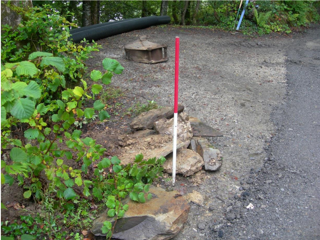
Fig 36 Lay-by above caravan north of oval fort, prior to laying of drain, looking NE
