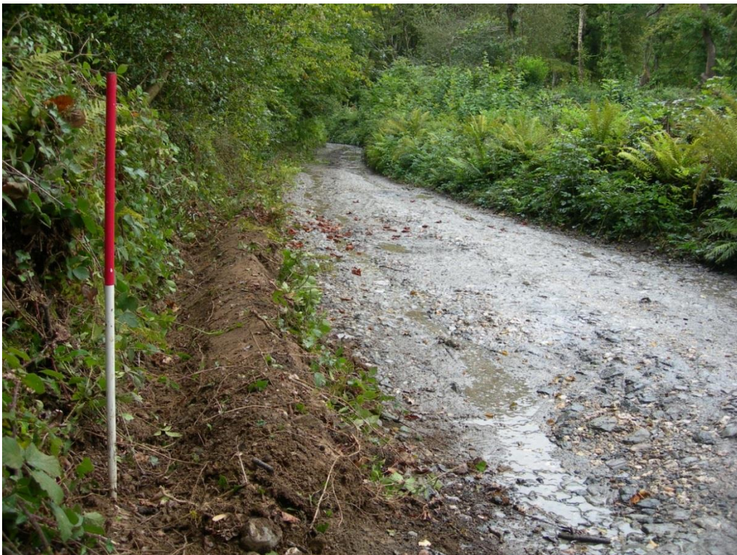
Fig 31 South western drain, with spoil turned onto the roadside, from its upper end
