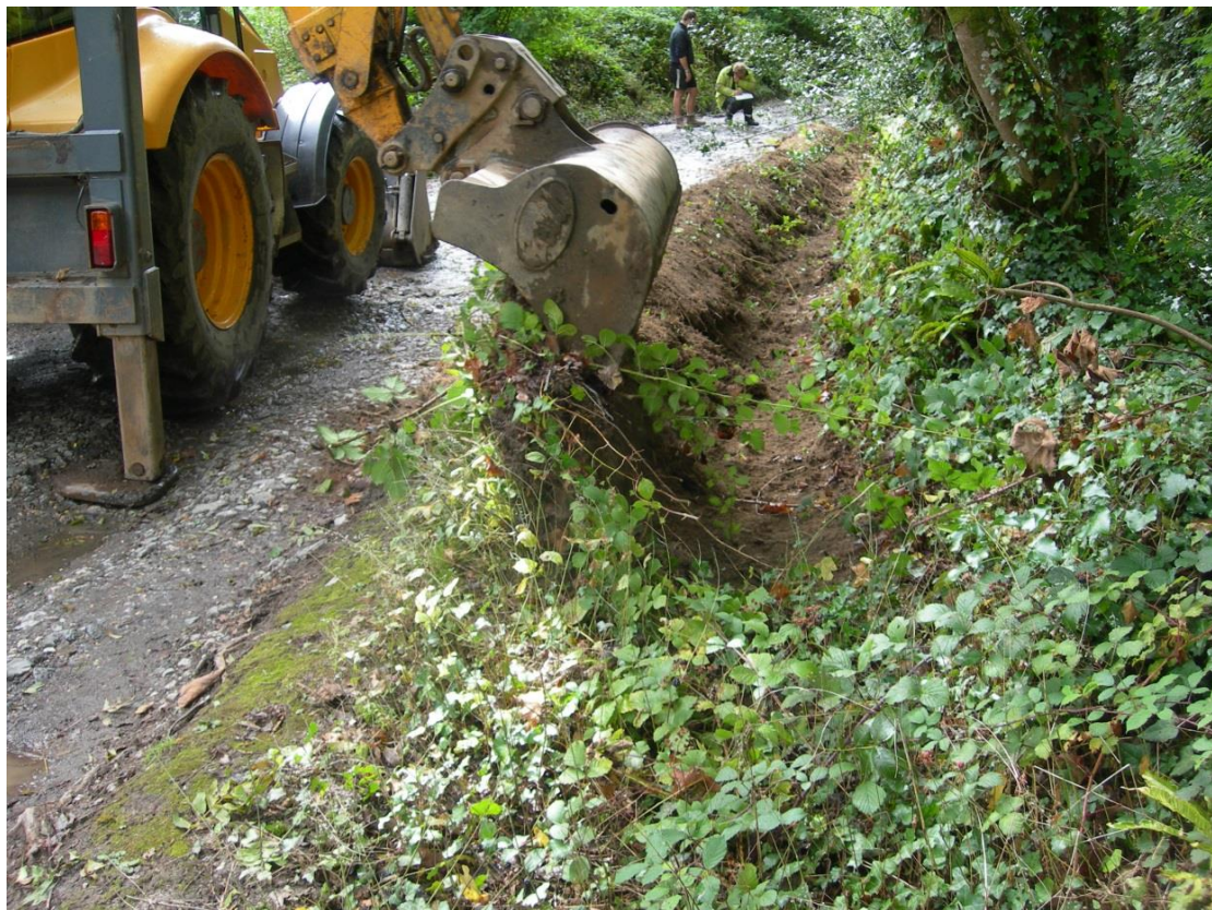
Fig 35 Excavation of north east drain; the inner cross-rampart is by the people beyond
