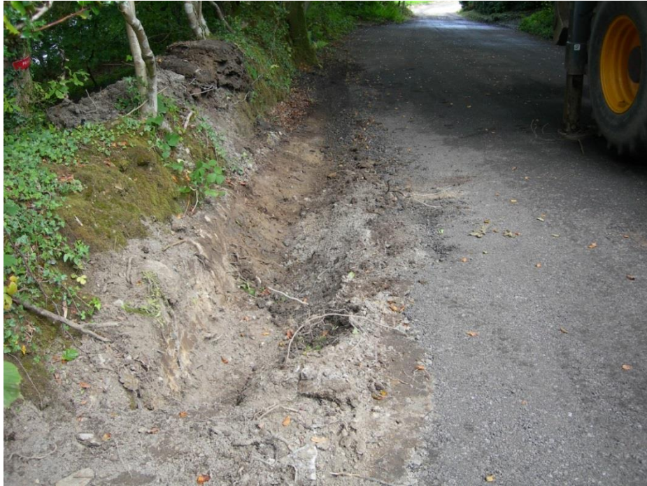
Fig 38 Lower end of north east drain, with spoil 'cast up' on lane boundary, looking NE
