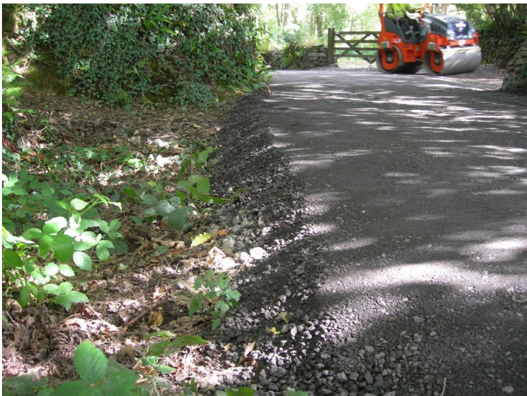
Fig 29 New road surface on the causeway over the ditch of the outer cross-rampart This required lengthy rolling to smoothen it, the causeway material being relatively soft.
