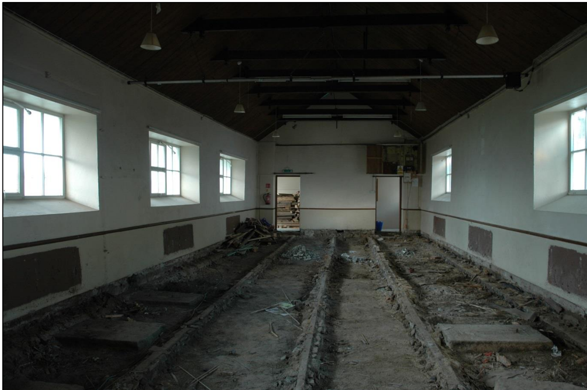
Figure 8: View of interior of Devoran Village Hall looking west, showing floor joists and stones B and C.
