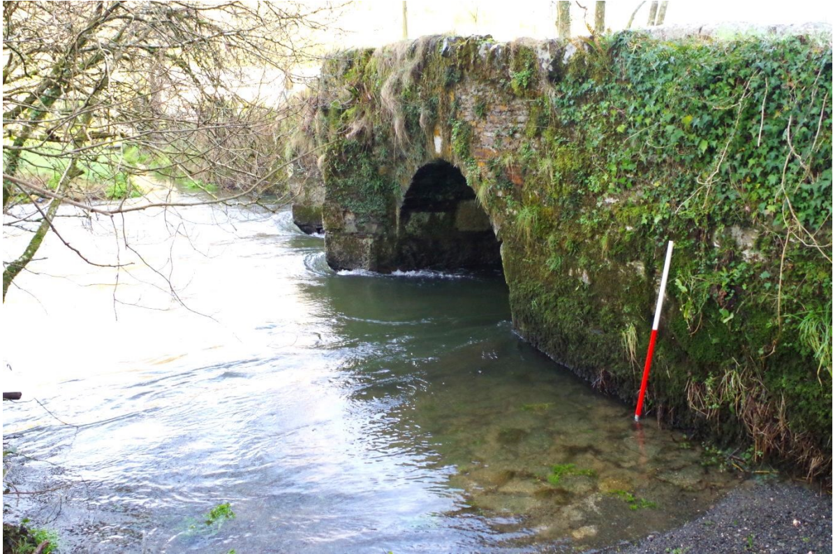
Fig 4 West elevation from the southern side. The cobbled surface of the access way is visible beneath the water surface.
