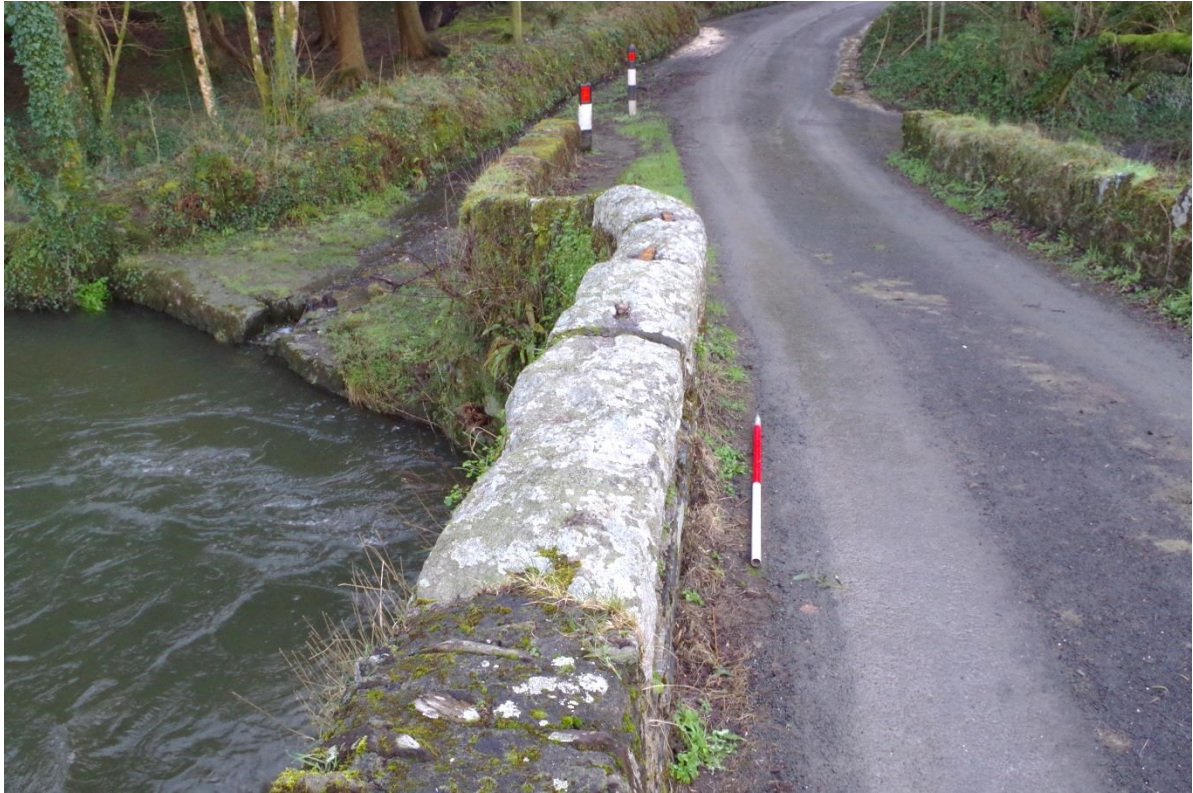
Fig 5 The line of five granite coping stones on the south eastern parapet. Note, the iron ties joining the blocks and access way to the left.
