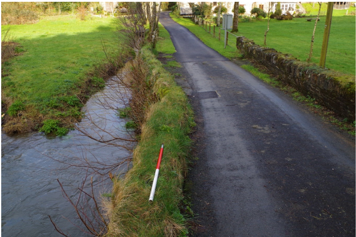
Fig 6 Young saplings growing out of the north western parapet. Note, the overflow leat of Trekener Mill to the left.
