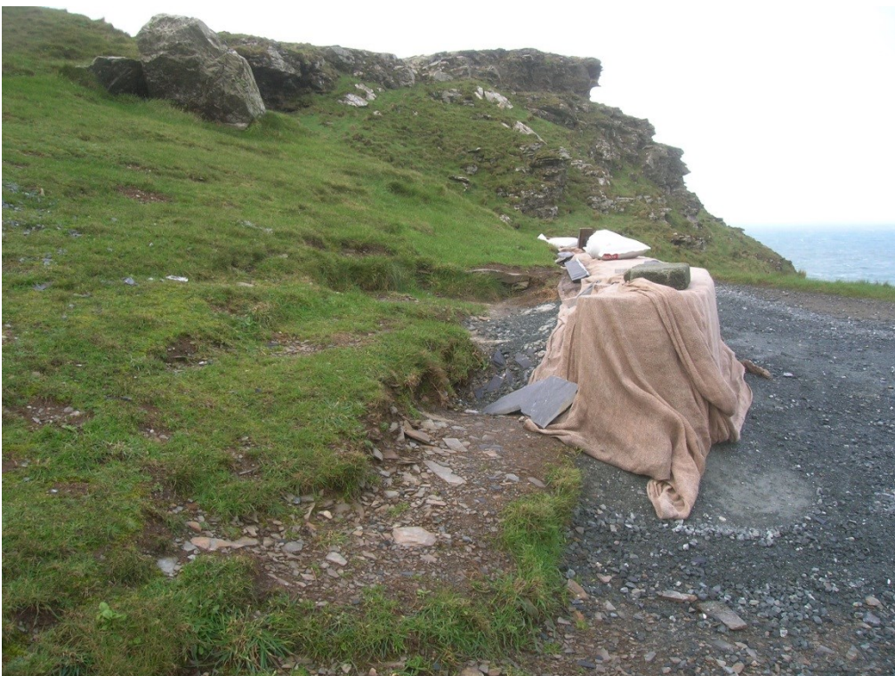
Figure 10. Bench 1. Walling completed. Gap behind wall and the hill scar will be infilled with soil and turfed over.
