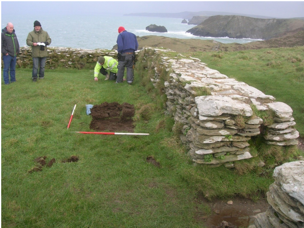
Figure 8. Excavation of slots for slate slabs in progress within garden (Sign 19). Slot 1 is in the foreground, with slot 2 in the process of being dug.
