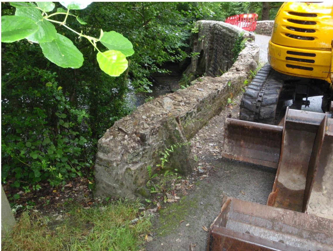
Fig 9 Damage to the eastern coping, south side of the Clapper Bridge.
