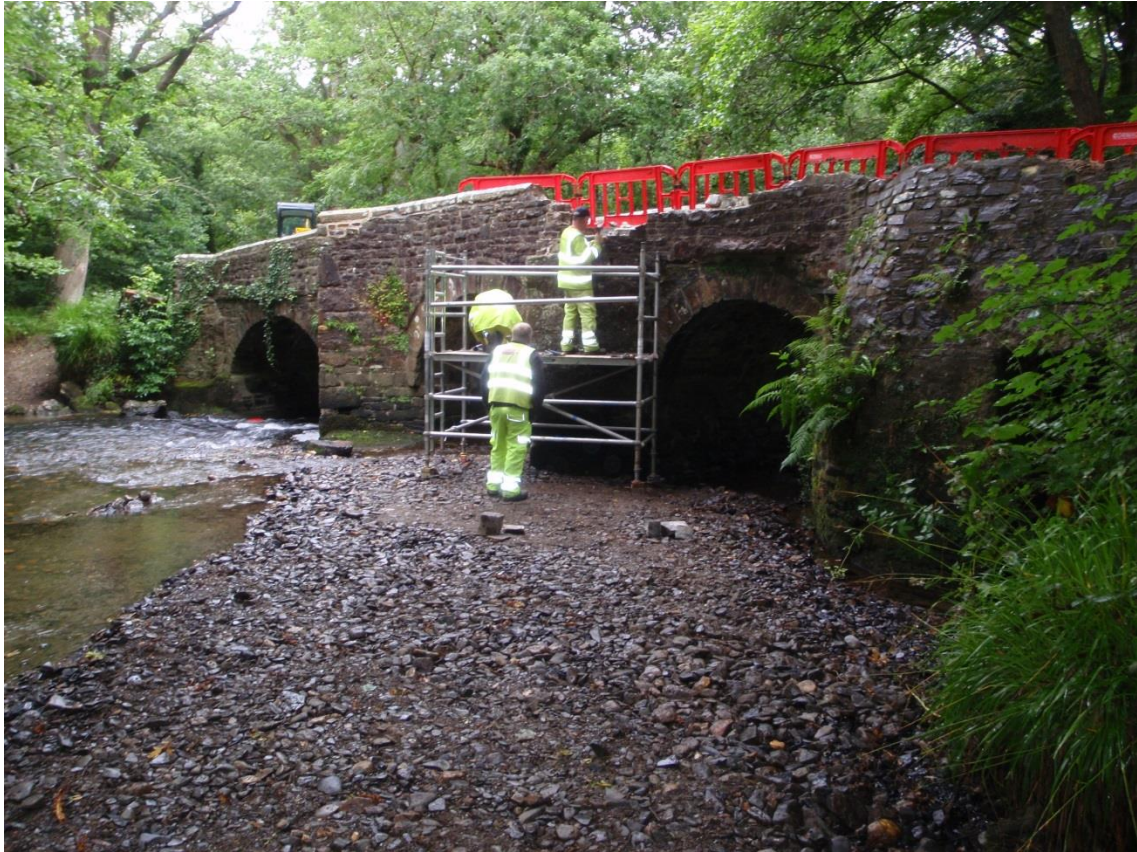
Fig 10 Damage to the wall and cutwater on the north side of Clapper Bridge.
