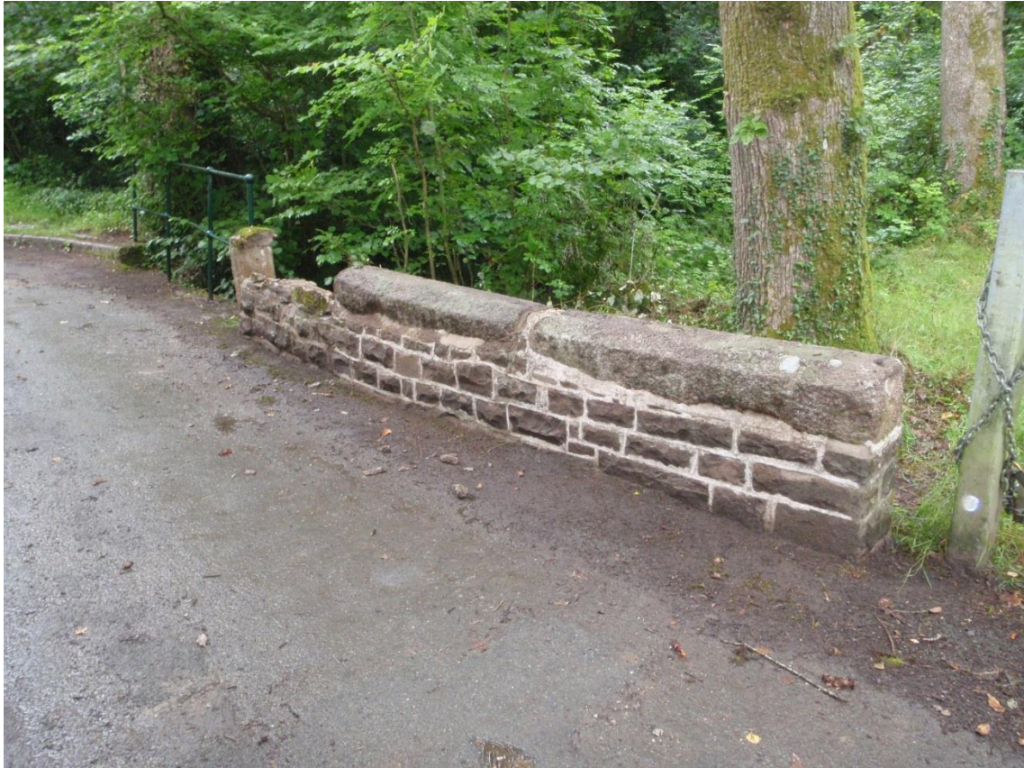
Fig 8 Damage and recent repairs to the Bay Park Clapper Bridge.
