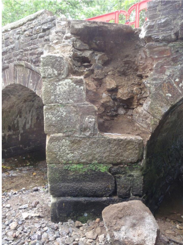
Fig 12 Beneath the damaged cutwater.
