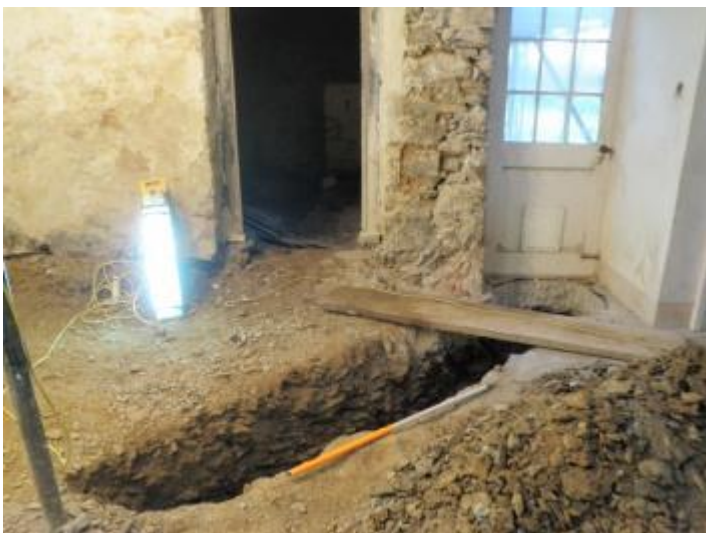
Fig 6 Top – Looking west across the excavated floor level showing the western wall base. Note the roots extending in from outside. Middle – Looking north in to the former stable showing the exposed wall masonry and concrete flooring prior to the trench excavation. Above left- the internal excavated pipe trench. Above right – the excavation of the external trench in progress.
