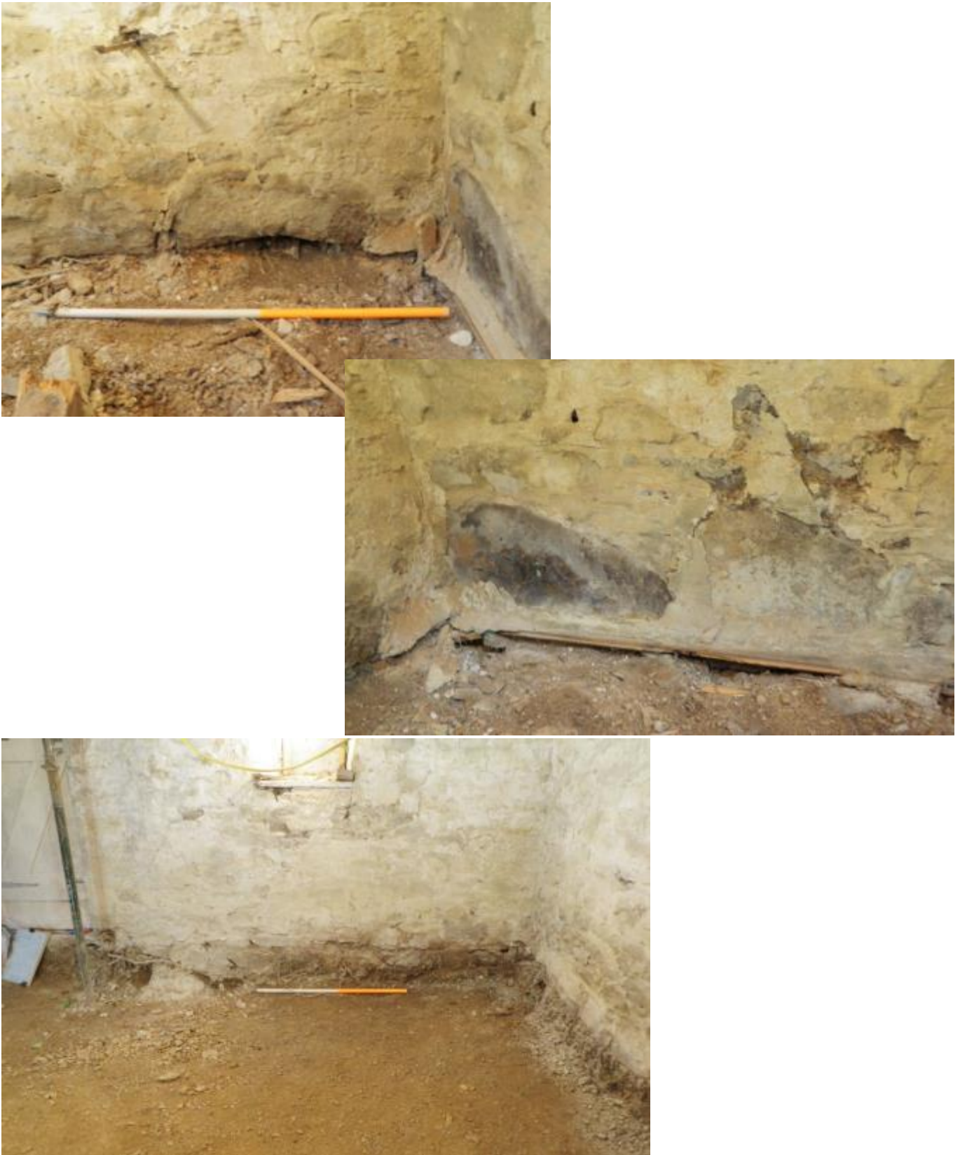
Fig 5 Top – Looking west at the notably large foundation stones supporting the wall in the north western corner of the room. Middle – looking north towards the remnant wooden flooring, showing loose animal disturbance beneath it. Bottom – looking south towards the former trial pit, showing the probable pillar-base stone.
