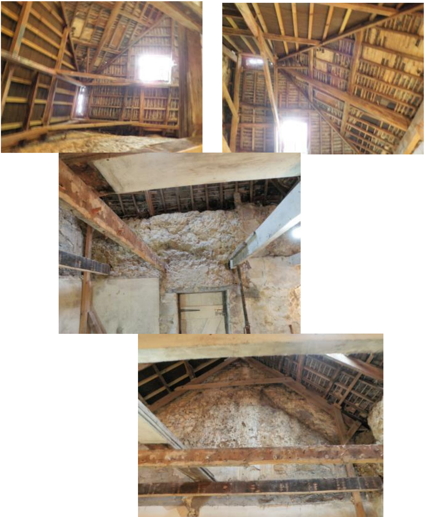
Fig 7 Top left and right - Looking at the exposed roof timbers, showing frequent phases of repair. Middle - View of the south wall showing phasing within the exposed cob walling, a former roof line and the later ceiling supports cutting in to it. Right - looking east at the exposed cob walling against the stone vicarage wall (clearly showing an earlier lower roof line).
