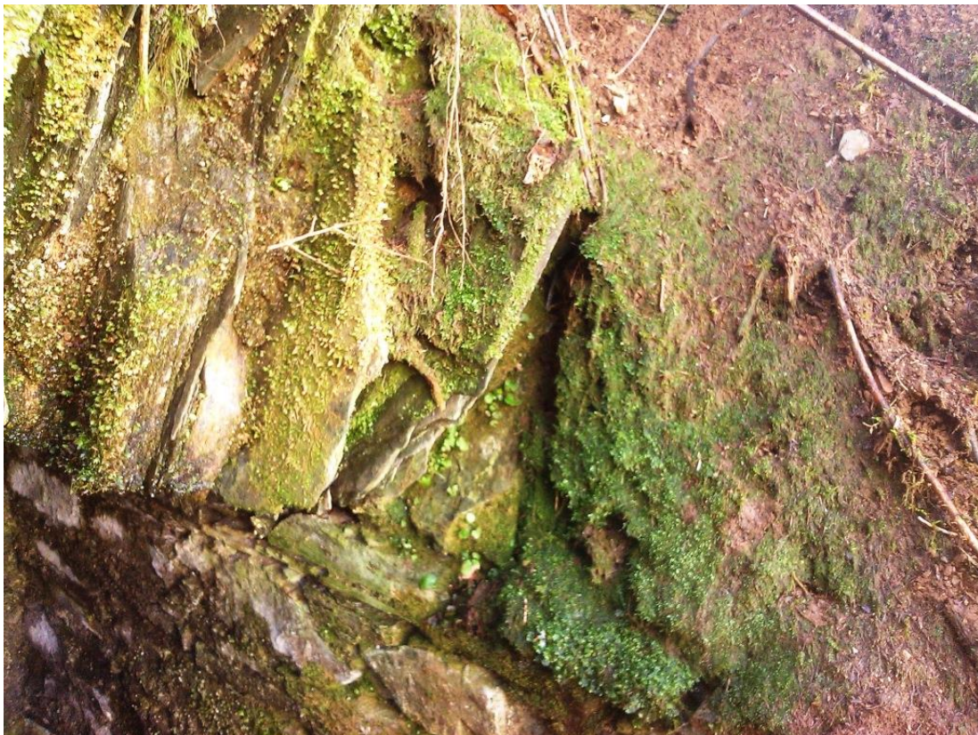
Fig 17 Outer part of the surviving roofing on the north-west side of the well house, with remains of the collapsed vaulting in front (the mossier slabs, right of photo)
