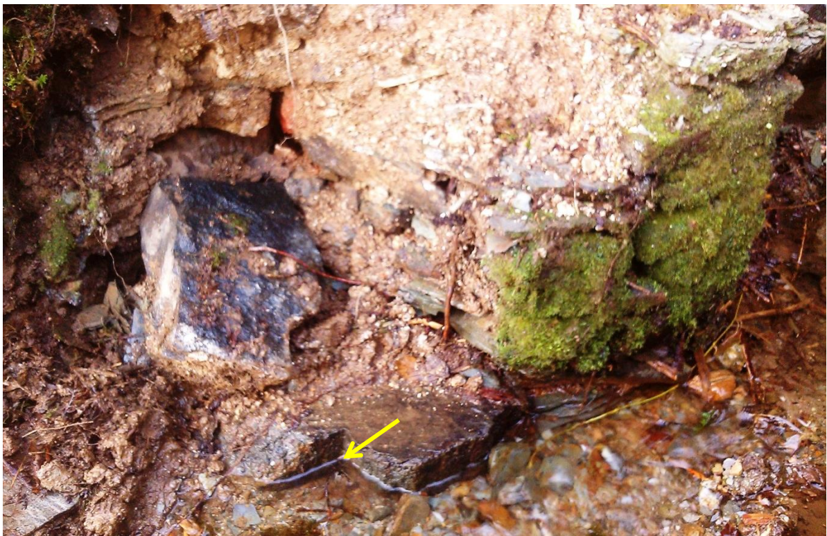
Fig 4 South-east side of the doorway showing a stone at the entrance, rebated for a door, and above it, collapsed stonework
