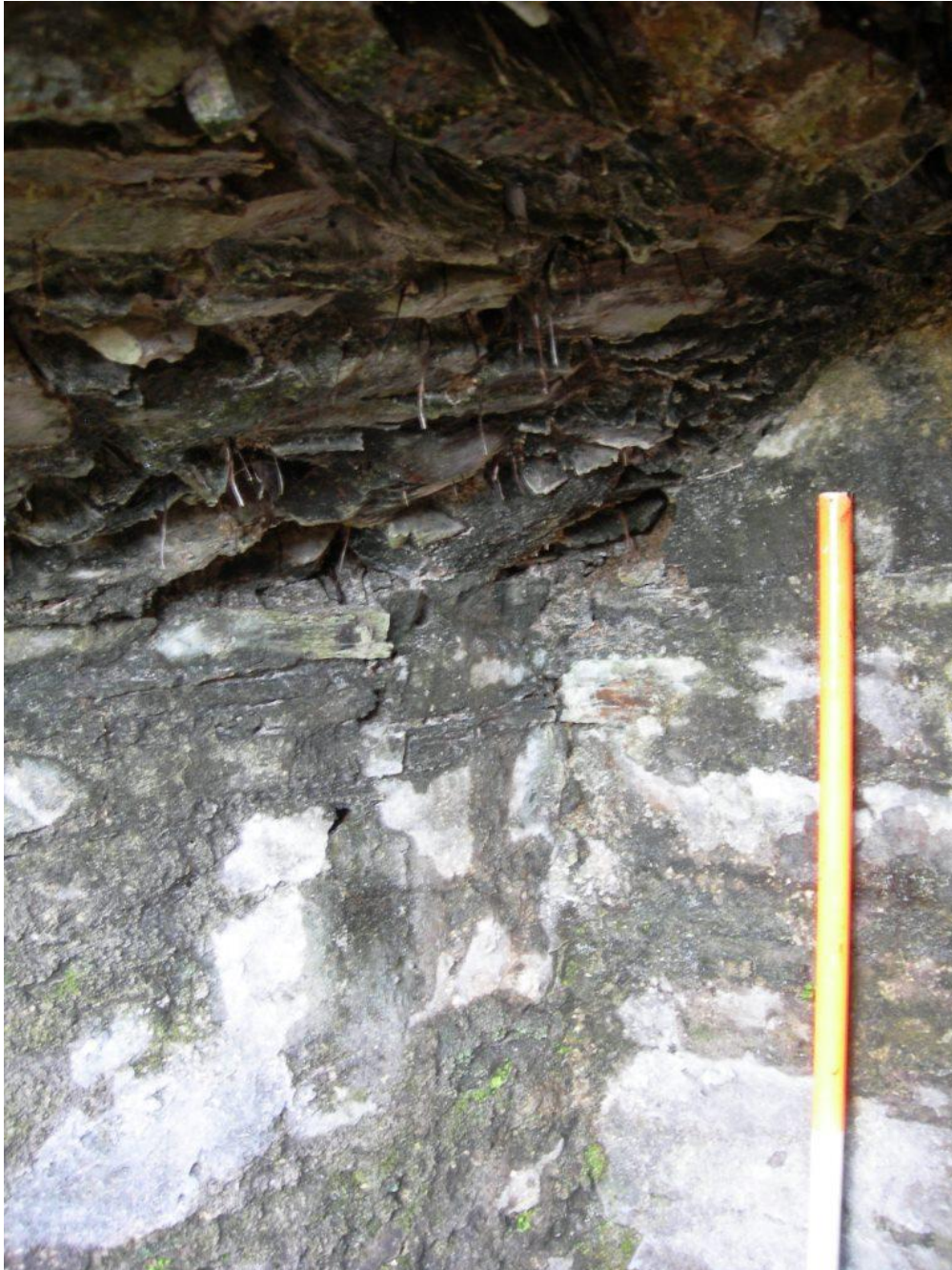
Fig 13 South corner of the well house, with its rear wall rising to the right with the arch of the vaulted roof of rough slate slabs (scale divisions are 0.5m)
