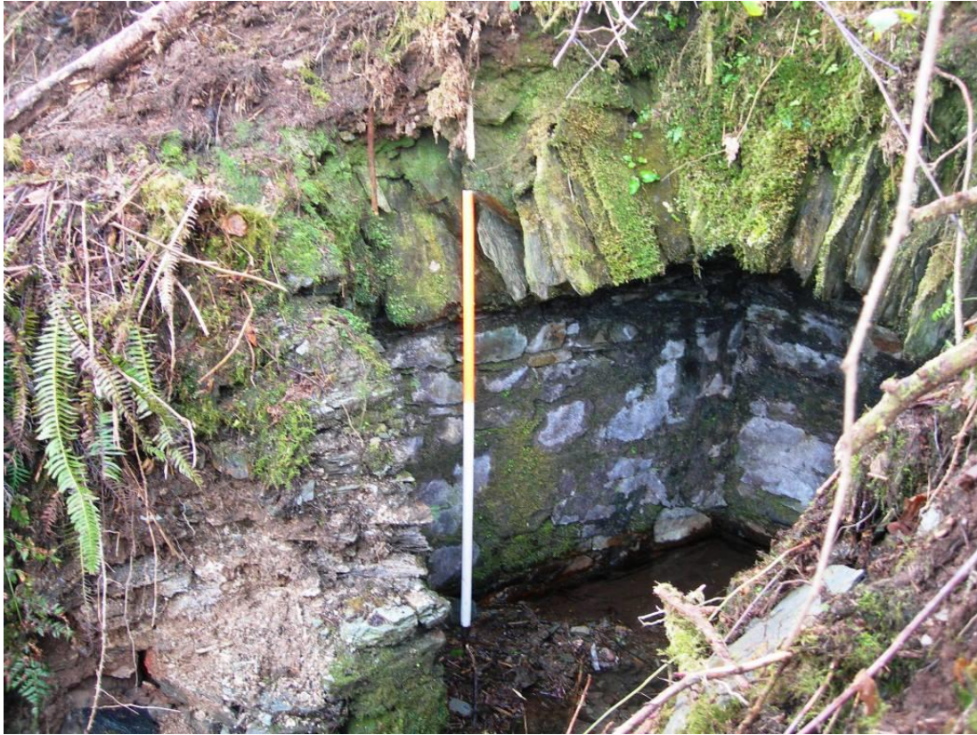
Fig 16 Well house from the north, showing decay of front wall and loss of roof above
