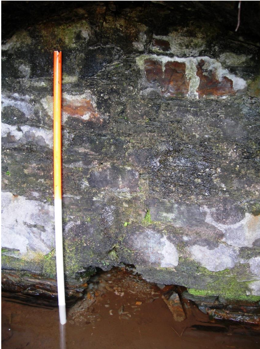
Fig 15 Rear wall inside the well house, with damage to stonework in its centre (1m scale)
