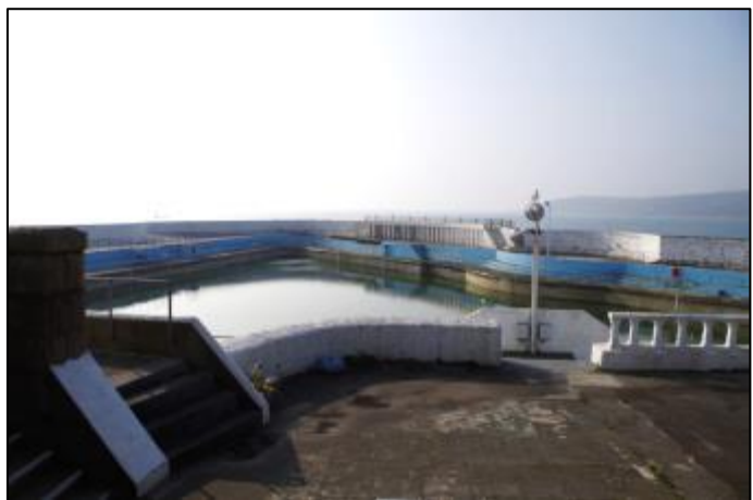
Fig 12 The Jubilee Pool lido, Penzance, built in 1935 on the foreshore of a small cove to the west of the main harbour. The lido incorporates the early 19 th century Battens Wharf.
