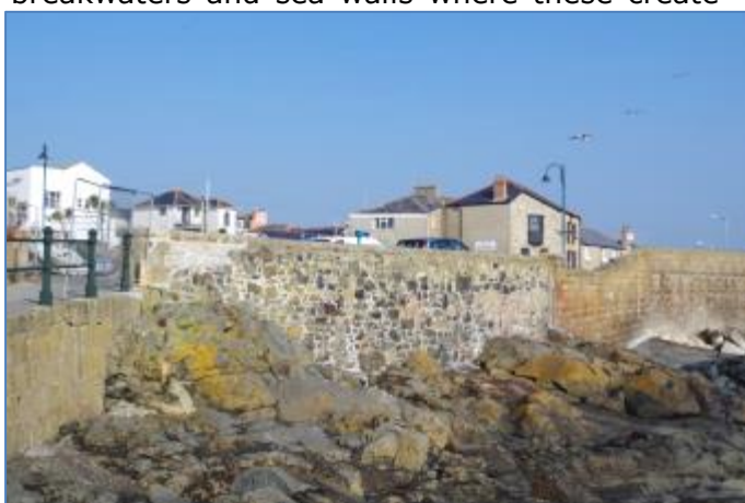
Fig 14 Historic phases of sea wall construction adjoining the South Pier, Penzance Harbour.
