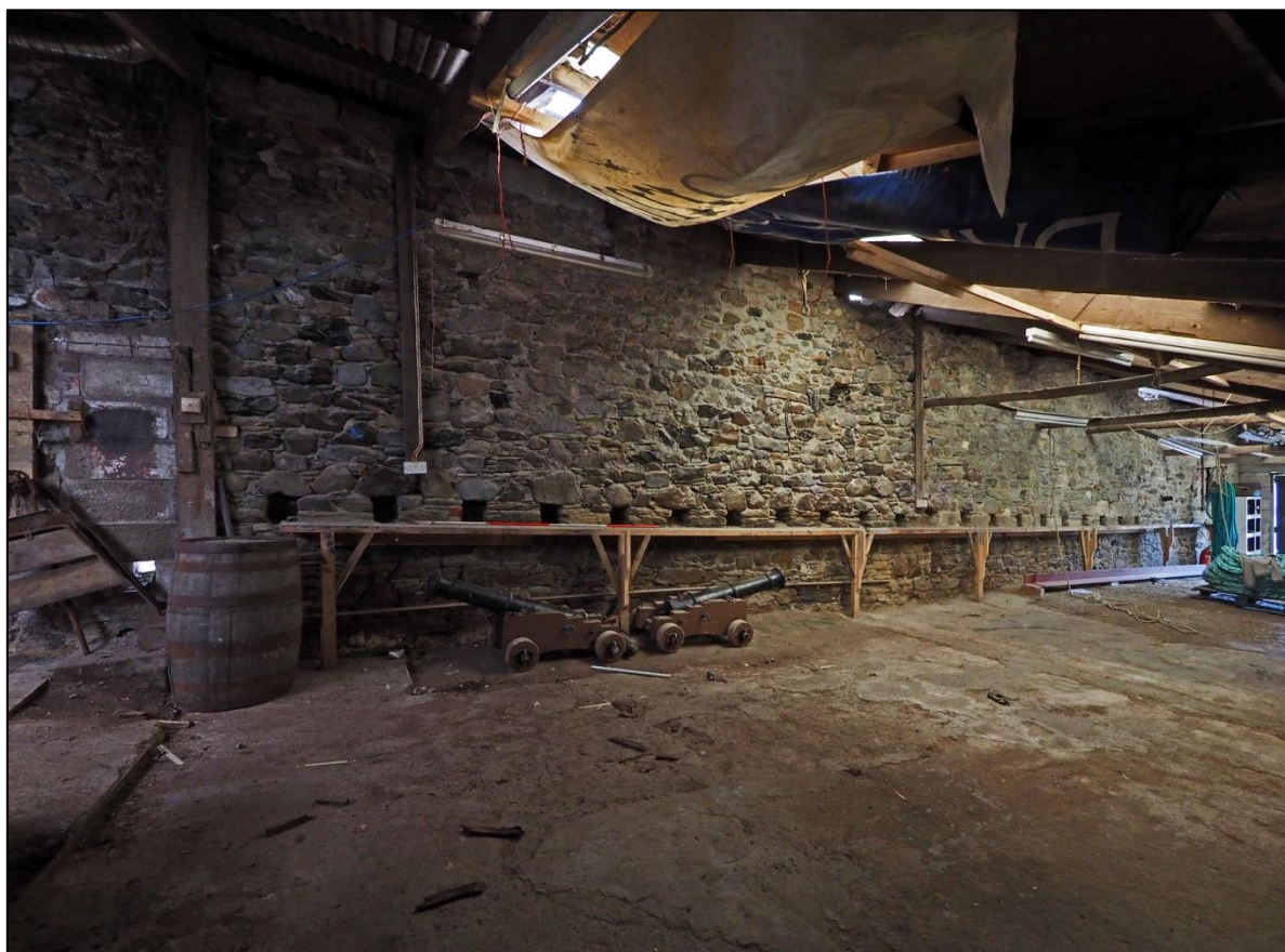
Fig 22 Interior of a former pilchard pressing shed at Charlestown, with pressing beam sockets in the wall. The building was subsequently used as sailmaker's workshop and store and is being converted into a restaurant (Photograph: Eric Berry).
