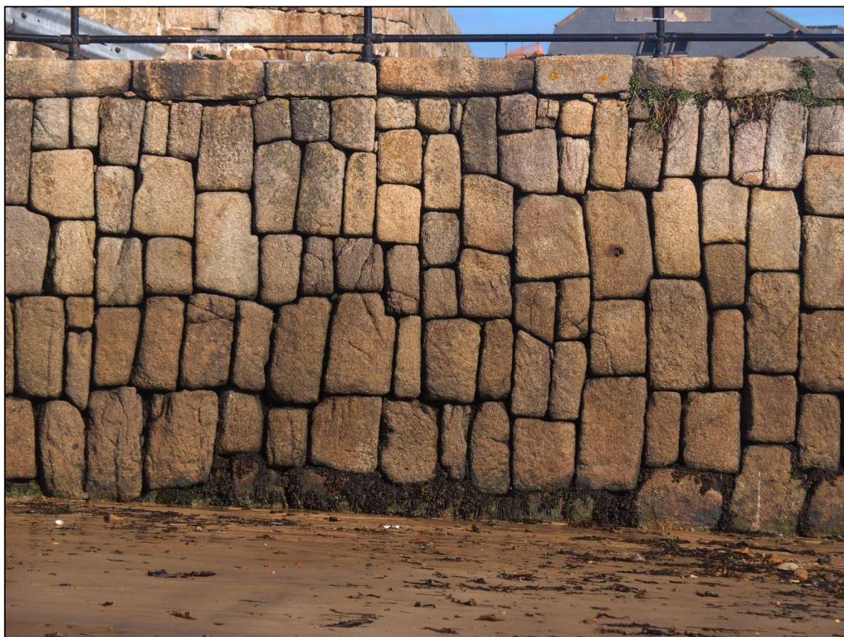
Fig 10 The Old Quay at St Mary's Harbour has demonstrable evidential value, the original quay, dating to the early seventeenth century was rebuilt between 1749 and 1751 (Photograph: Eric Berry).
