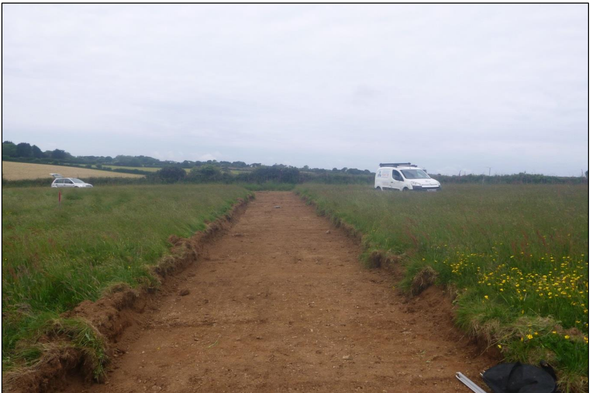
Figure 4: Post excavation view looking west along the path of the access track.
