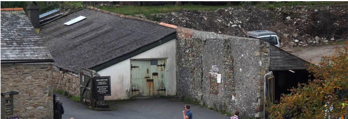
Fig 12: Subject sheds from across the harbour dock (note the spine wall against which the two lean-to roofs abut)
