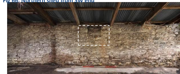
Fig 68: Northern shed NW wall with second blocked window within dashed line, the blocking fitted with chute
