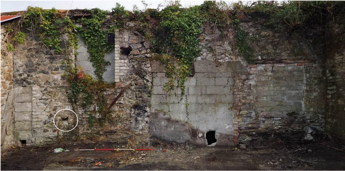
Fig 11 : This is the right-hand (SW) end of the spine wall that runs between the two subject sheds (see also elevation phase drawing) The socket towards the left (circled) is the last of a series of pressing-bean sockets, most of which are visible within the northern shed
