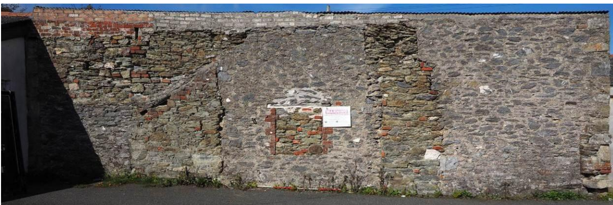
Fig 10: SE wall of northern shed, NE end (see also Fig 7: annotated elevation from other side))
