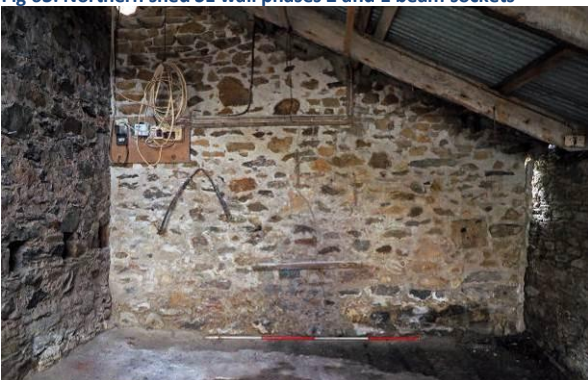
Fig 65: Northern shed SW later inserted wall
