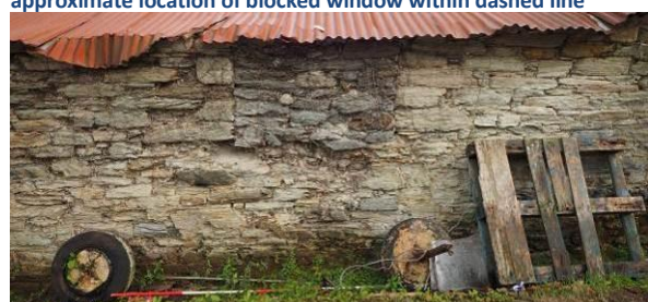
Fig 26: : NW wall of northern shed showing blocked window towards right of surviving wall
