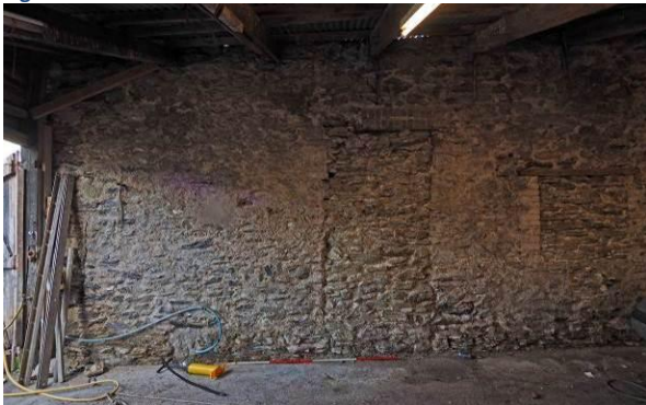
Fig 53: Northern shed SE wall far left (note blocked openings)
