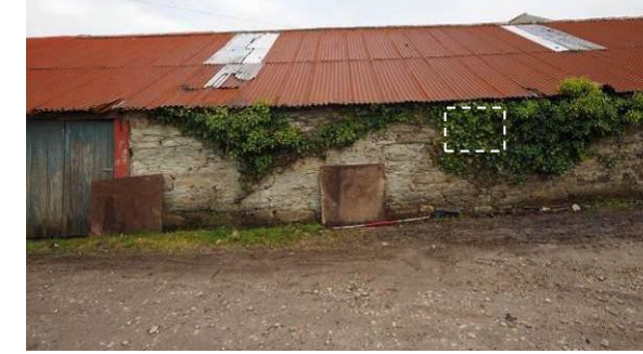
Fig 24: : NW wall of northern shed, right of centre with approximate location of blocked window within dashed line
