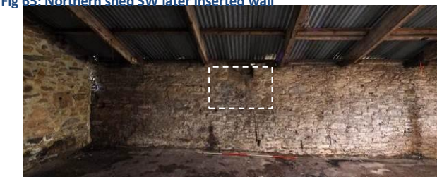
Fig 67: Northern shed NW wall far left with blocked window within dashed line, the blocking fitted with chute
