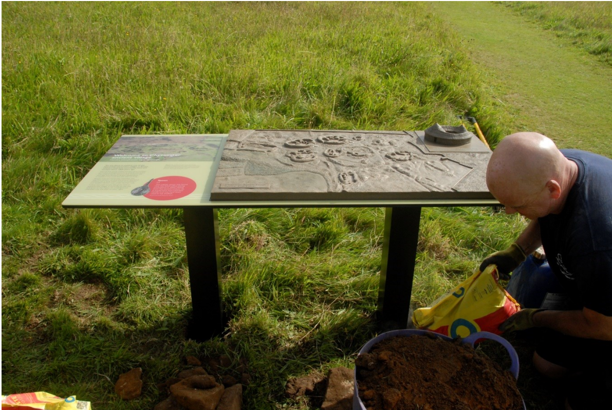
Fig 22. Concreting in the legs for new Interpretation Panel 1 near the ticket hut at Chysauster. This panel incorporates a 3D plan of the site derived from the 2016 Historic England survey.
