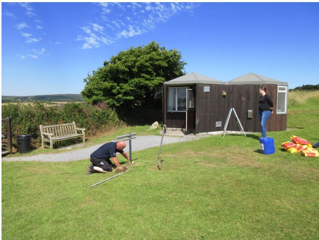
Fig 11. Hand excavating to remove the original Operational Sign 1 near the Chysauster ticket hut.
