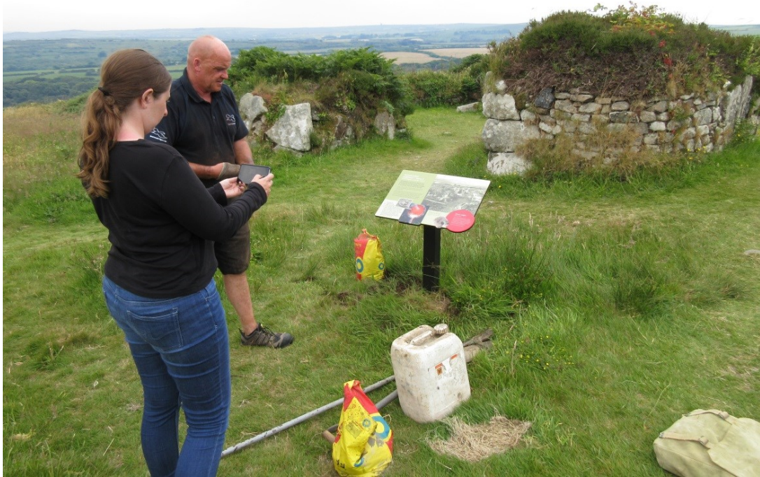
Fig 20. Completion of the installation of new Panel 7 adjacent to Houses 3a and 3b at Chysauster.
