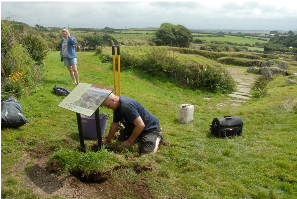
Fig 25. Replacing the turf at the site of Panel 2 at Carn Euny. The new interpretation panel was mounted on the original shallowly-buried baseplate rather than being set into postholes.
