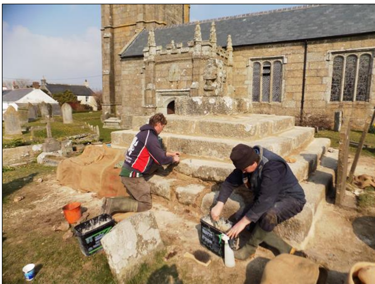
Fig 32 Conservation work in progress: deep pointing of the joints of the cross pedestal in a lime-based mortar (AGL, APJ).
