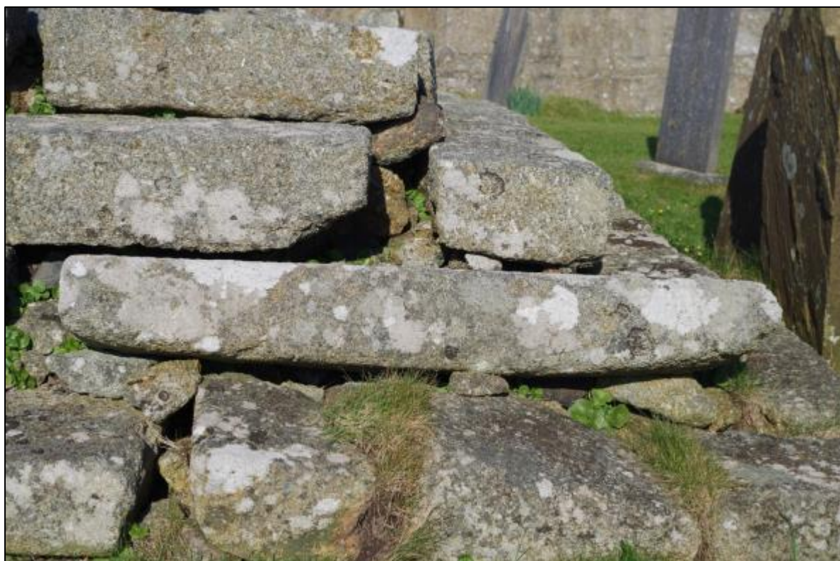
Fig 11 Detail of south east corner showing uneven and collapsing stonework (JG).
