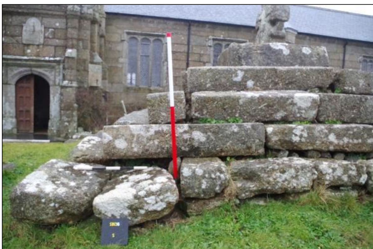
Fig 12 South west corner showing slumping of stonework (JG).
